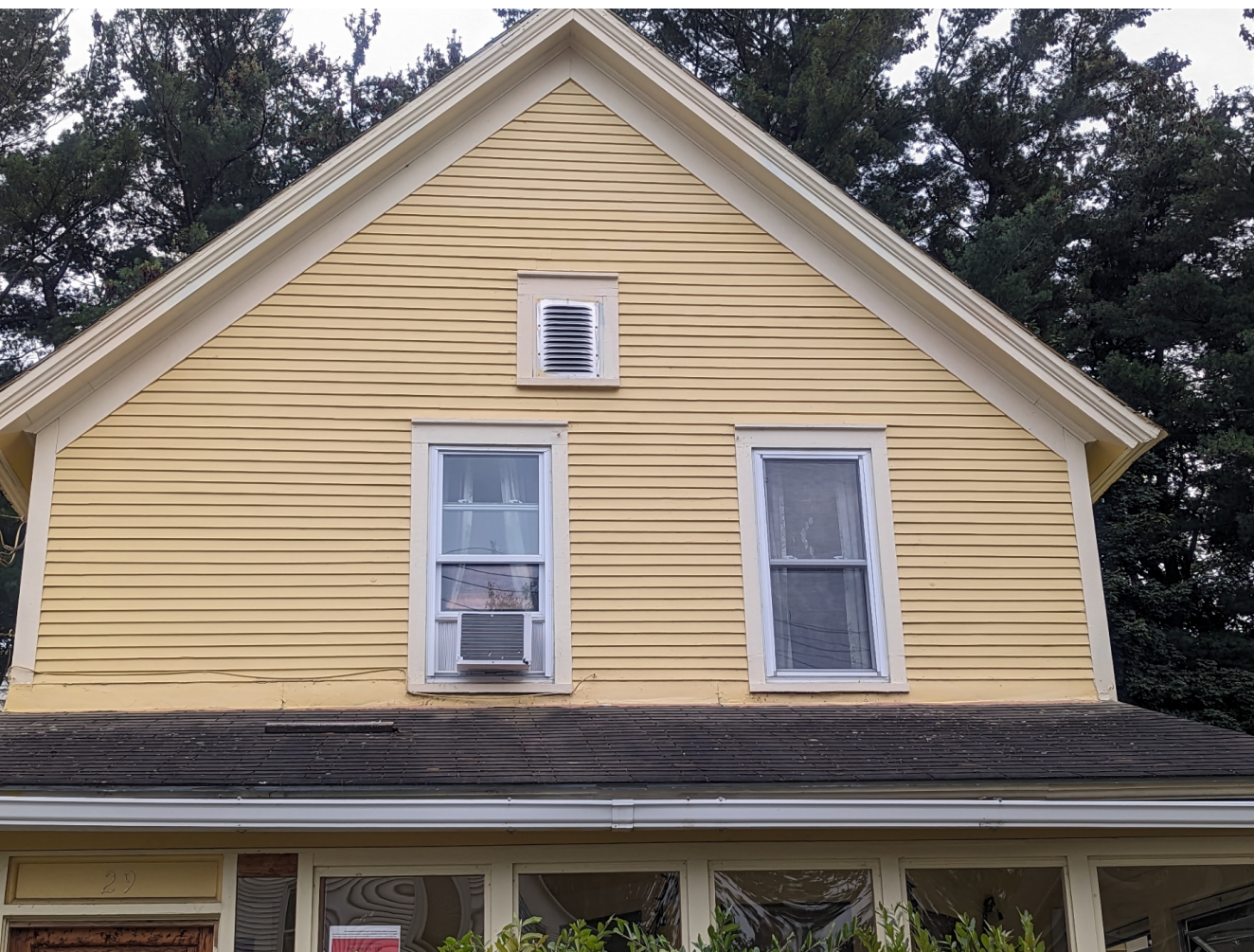
Figure 4: Fl2 N wall Bedroom (2) 2-3
