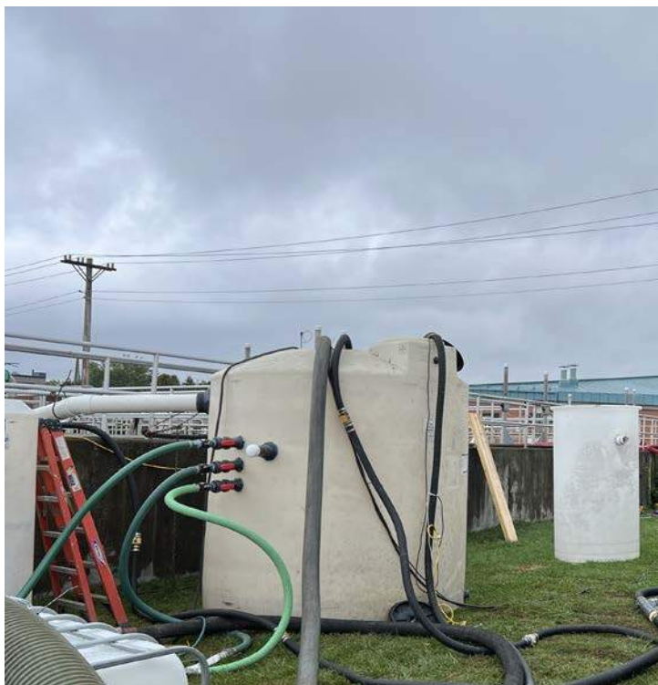
Figure 8: Influent Mixing Tank
