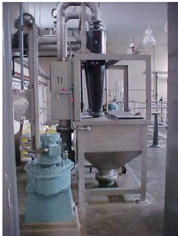
Hydro Cyclone Unit
