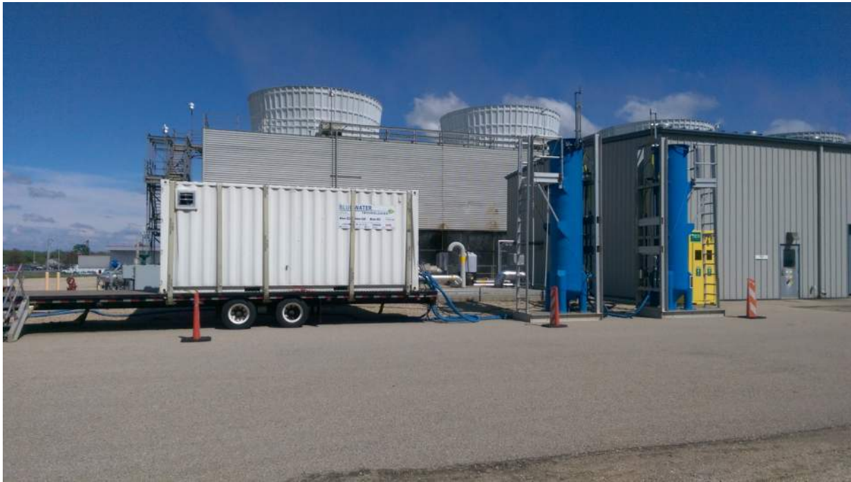
Filters in line with container and trailer (Energy Plant - WI).
