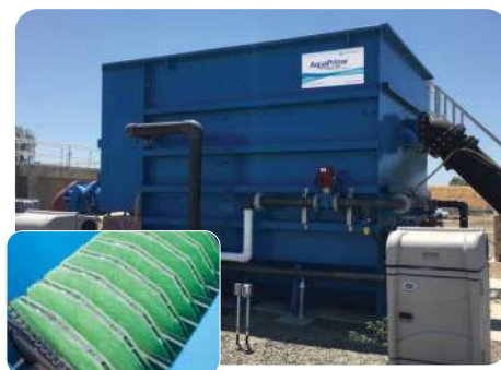
Linda County Water District, Olivehurst, CA
