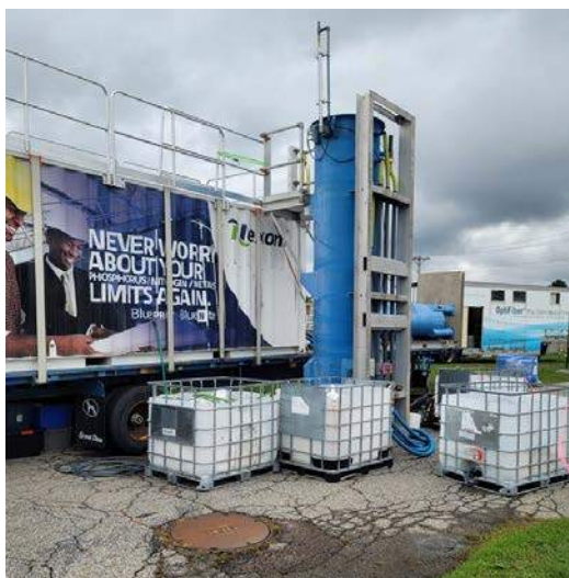
Figure 3. Blue PRO pilot at the Burlington treatment facility
