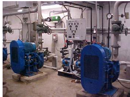
Sand Return Pumps
