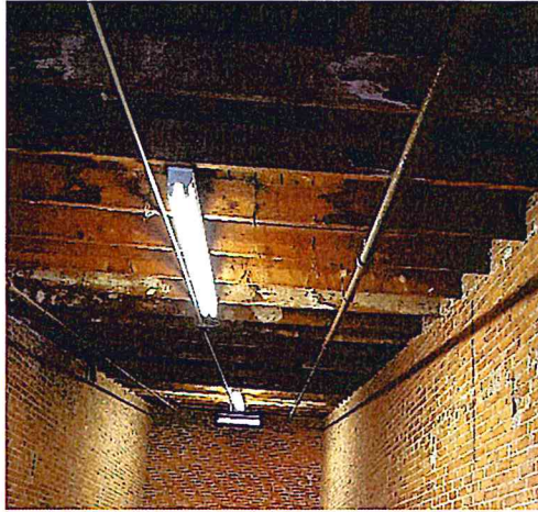
RAFTER ROT AND SAG
