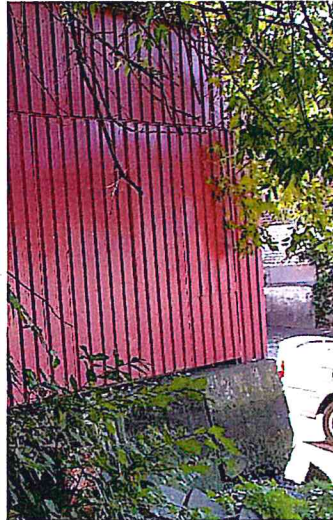
FOUNDATION FAILURE @ NW CORNER
