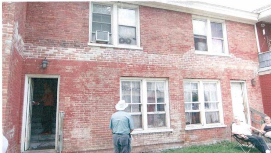
East side of wing facing George Street. Replacement windows on second floor, ghost of former porch below second floor windows, replacement bricks and mortar evident in various locations.
