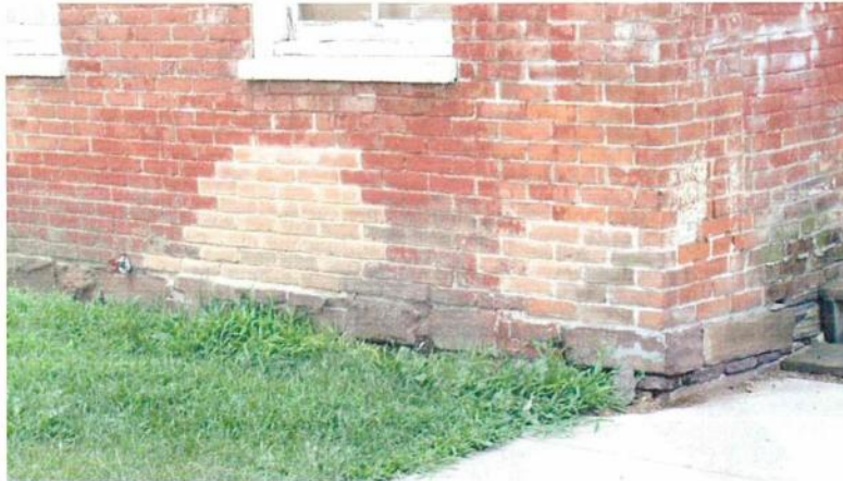
Northeast corner of main block with inappropriate brick and mortar replacement, loss of mortar in foundation.
