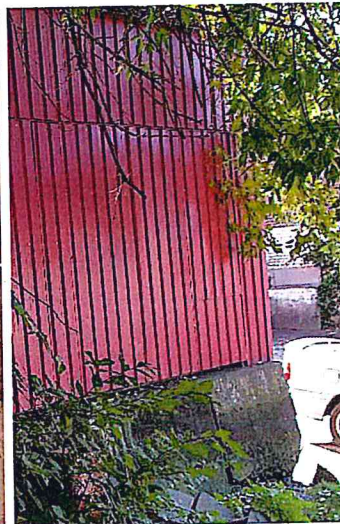
FOUNDATION FAILURE @ NW CORNER
