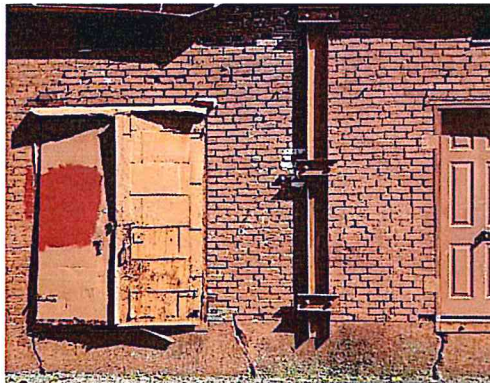
FOUNDATION AND WALL CRACKS
