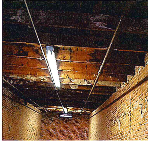
RAFTER ROT AND SAG
