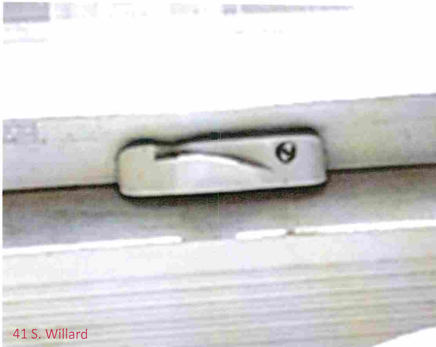
Conditions observed on 2-18-16 Photo taken by William Ward (close up of previous photo)
