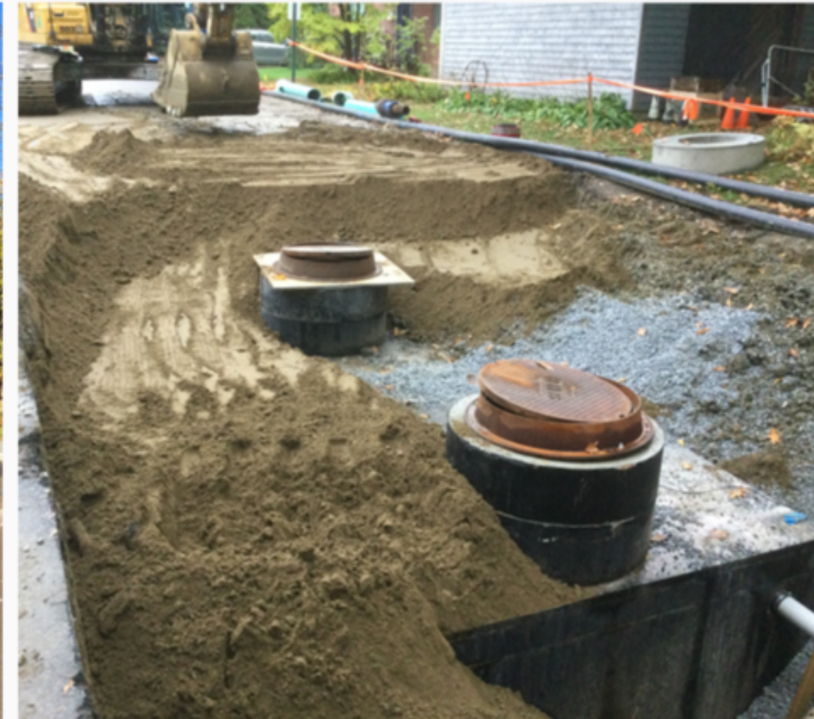
Fletcher Place Pump Station
