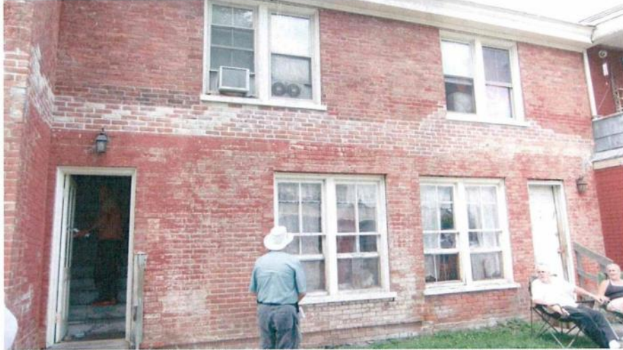
East side of wing facing George Street. Replacement windows on second floor, ghost of former porch below second floor windows, replacement bricks and mortar evident in various locations.
