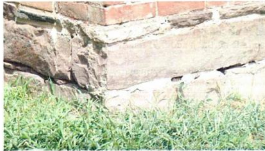
Detail of foundation exterior with missing mortar.
