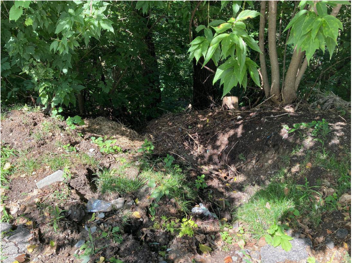
Photograph 3: View to north showing close-up of gully formation (Photo 2) from excess surface runoff at top of slope
