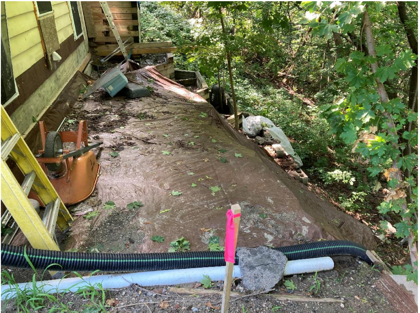
Photograph 12: View to west of the top of the slope behind the residence showing covered scarp and slump mass downslope from scarp
