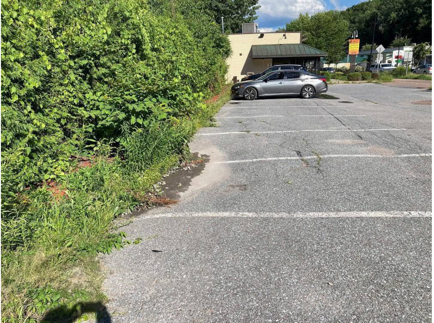
Photograph 14: View to east towards GBG Indian Kitchen showing localized incipient earth slumping in parking area at center of photograph; note area of recent ponded water; exposed historical failure scarp is present beyond trees to left.
