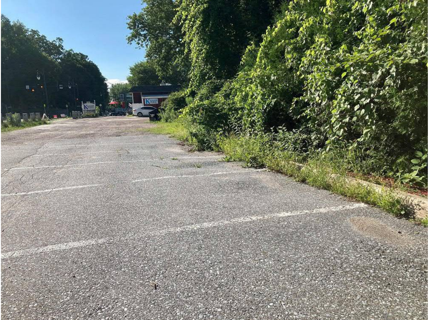
Photograph 13: View to west toward Kismayo Kitchen (505 Riverside Avenue) from GBG Indian Kitchen showing stressed pavement and surface depressions as an indicator of incipient soil slumping; exposed soil scarp is present beyond trees to right-center.
