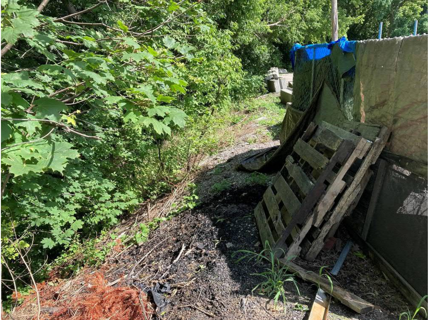
Photograph 9: View to east of top of slope adjacent to the eastern parking lot of Bluebird BBQ showing rounded surface expression of slope resulting from sheet flow during precipitation events; no surface expression of slumping or cracking apparent, but ongoing surface erosion will continue to cut back slope (see Photo 10 for view in opposite direction)
