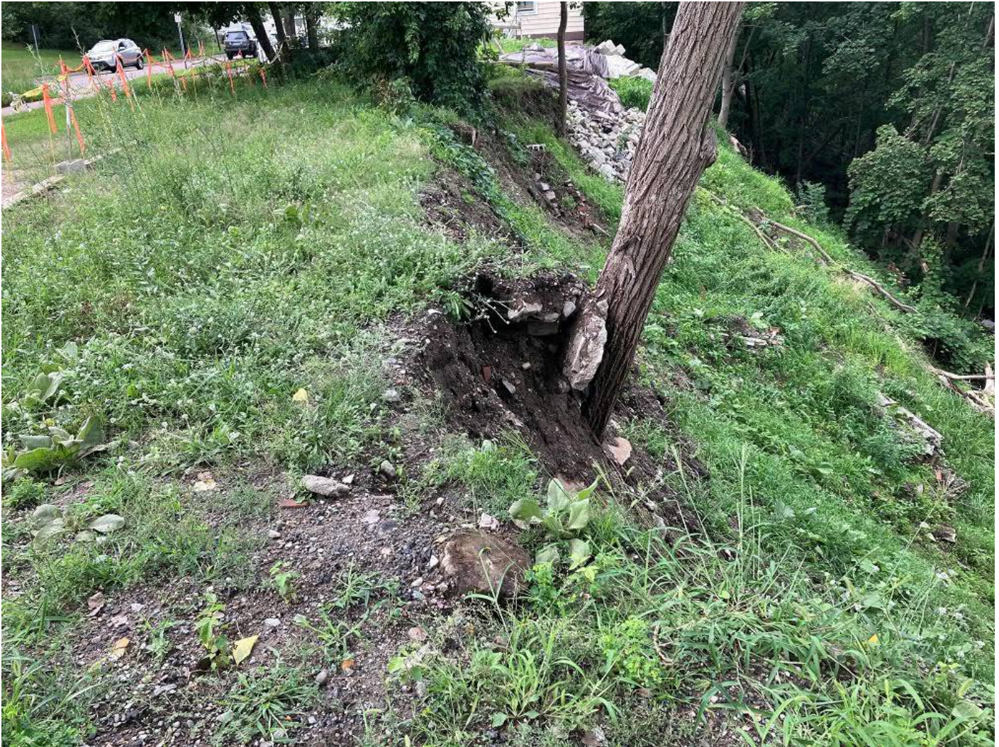
Photograph 25: View to west toward residence at 389 Riverside Avenue showing failure scarp at top of slope and overgrown slide/slump debris to center-right
