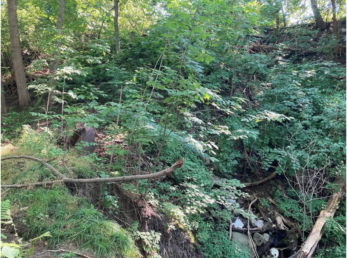
Photograph 7: View to southeast of stormwater discharge pipe (center of photograph) and gully formation from discharge; note debris in gully and exposed soil scarp at top of slope (top right of photograph) east of Kismayo Kitchen building
