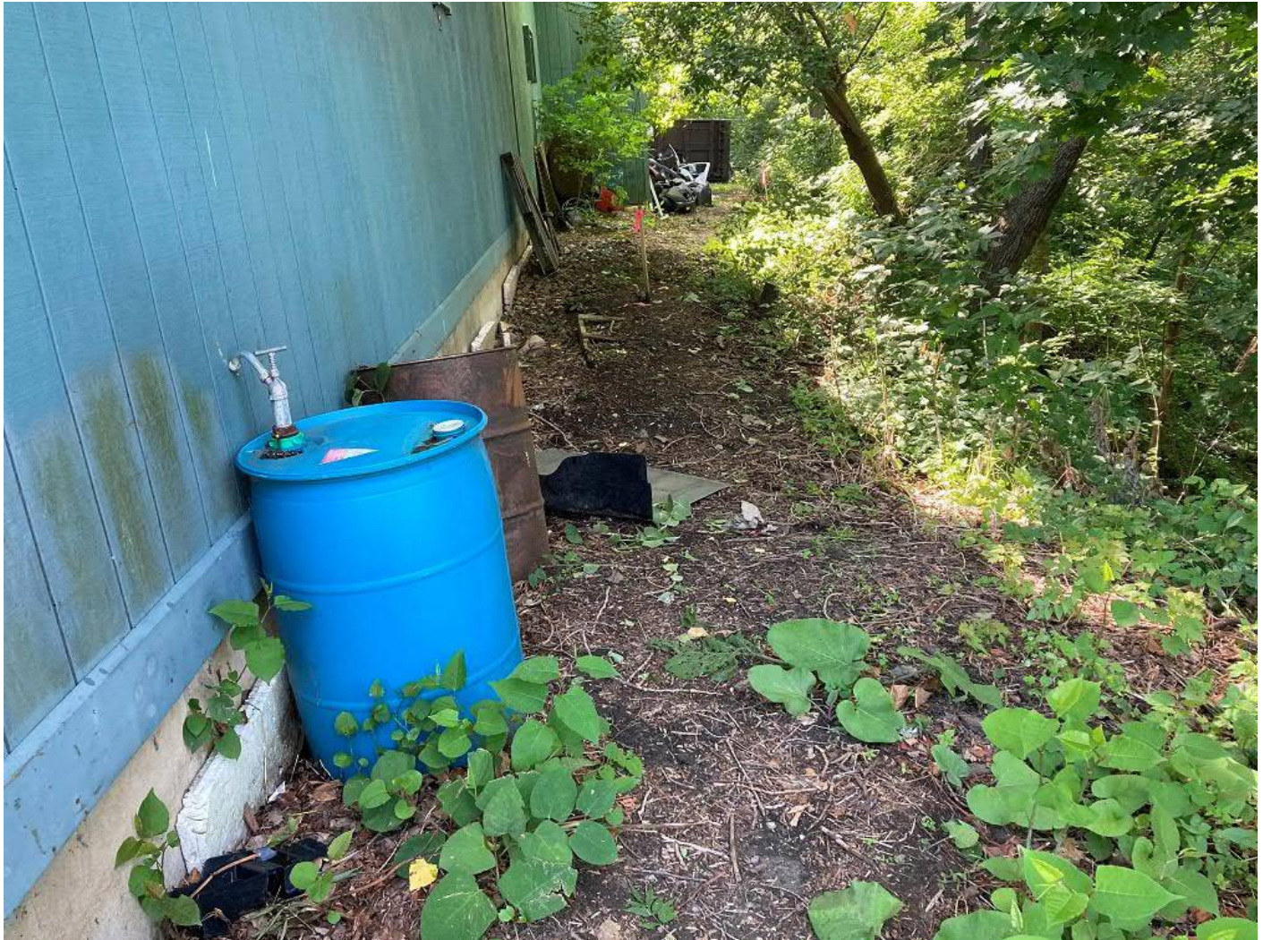
Photograph 3: View to west behind Burlington Collision showing incipient slumping at center of photograph; note leaning trees top right; soil scarp obscured by vegetation at center-right of photograph.
