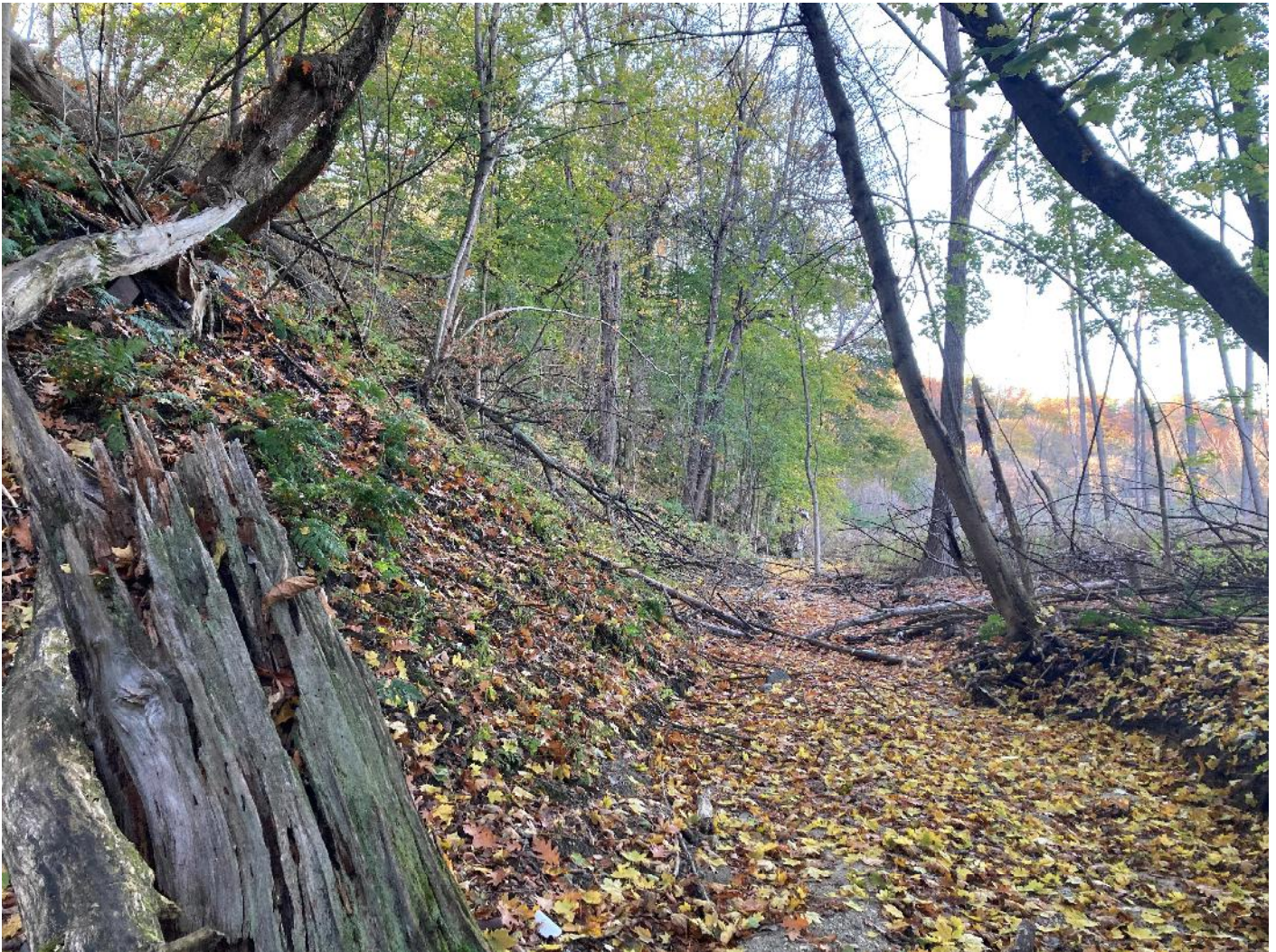
Photograph 26: View west-northwest showing discharge channel at base of slope; channel is directed towards wetlands at right-center of photograph; future high-flow events will continue to erode into toe of slope as shown in foreground.
