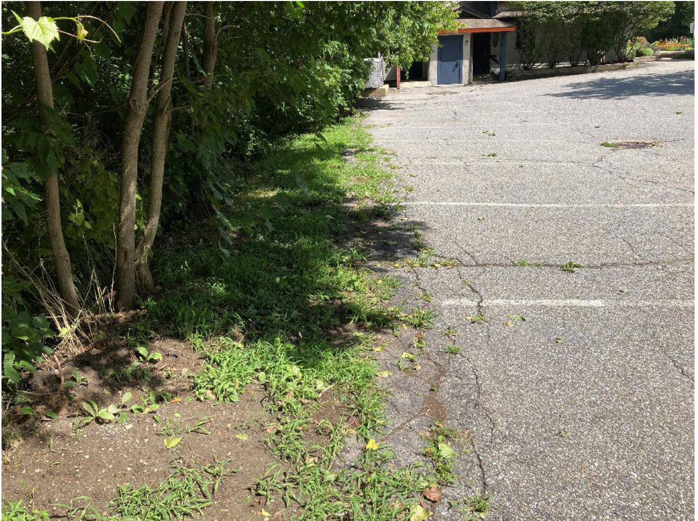
Photograph 2: View to east towards Bluebird BBQ building showing stress-release cracking in pavement at top of slope in west parking; cracking in pavement is a possible indicator of ongoing creep; gully washout from surface flow can be seen at bottom left of photograph
