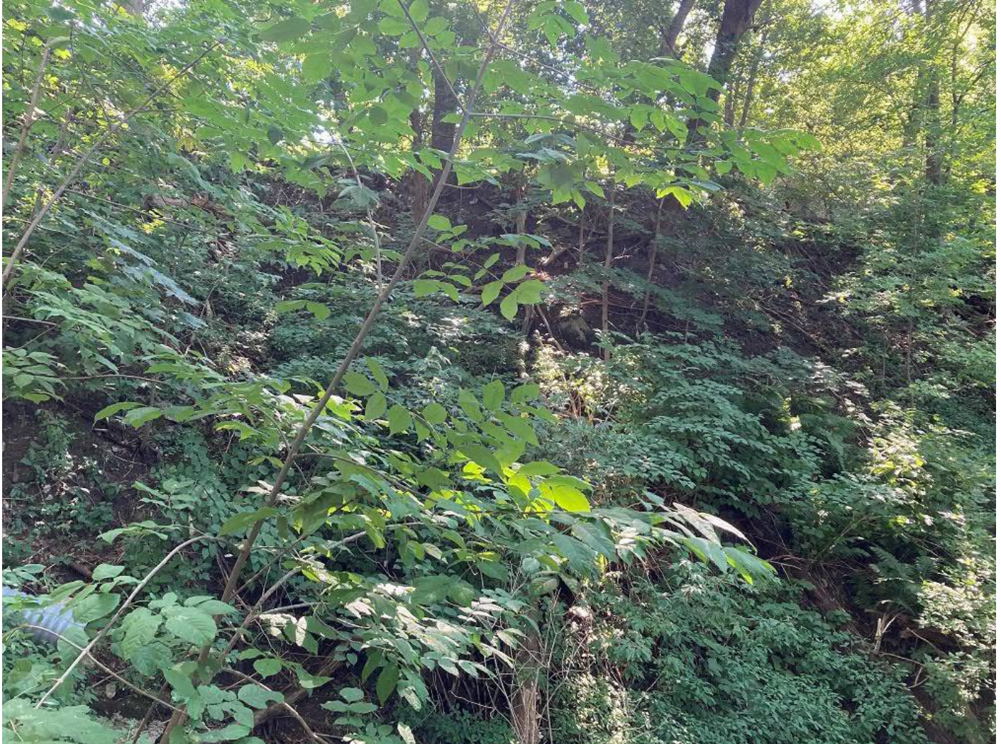
Photograph 6: View to southwest of exposed face of historical failure scarp; Kismayo Kitchen building can be seen at top right; note density of summer vegetation; exposed soil will continue to erode during precipitation events and top of slope will be subject to future localized failures; not discharge pipe at lower left of photograph.
