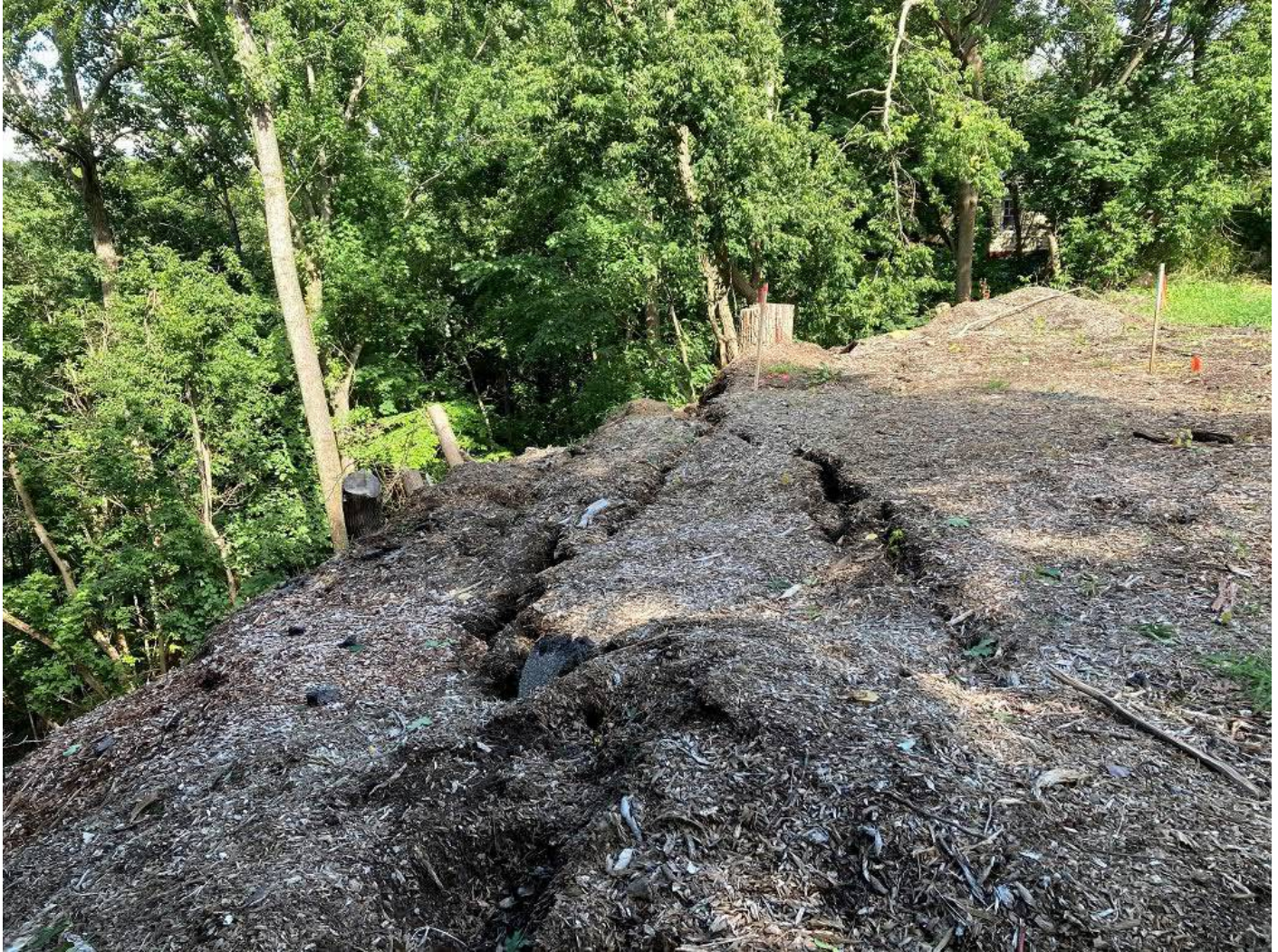
Photograph 6: View to northeast, additional view of crown cracks at top of slope, east of Burlington Collision building
