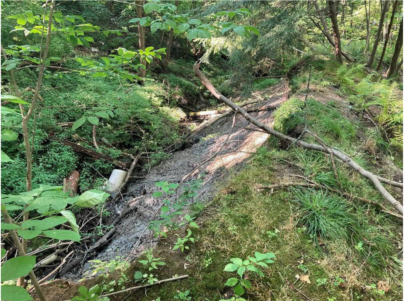
Photograph 8: View to north northwest of large gully formed in historic downslope slump mass by stormwater discharge; sides of gully will continue to collapse and expand with ongoing stormwater discharge; note density of summer vegetation.
