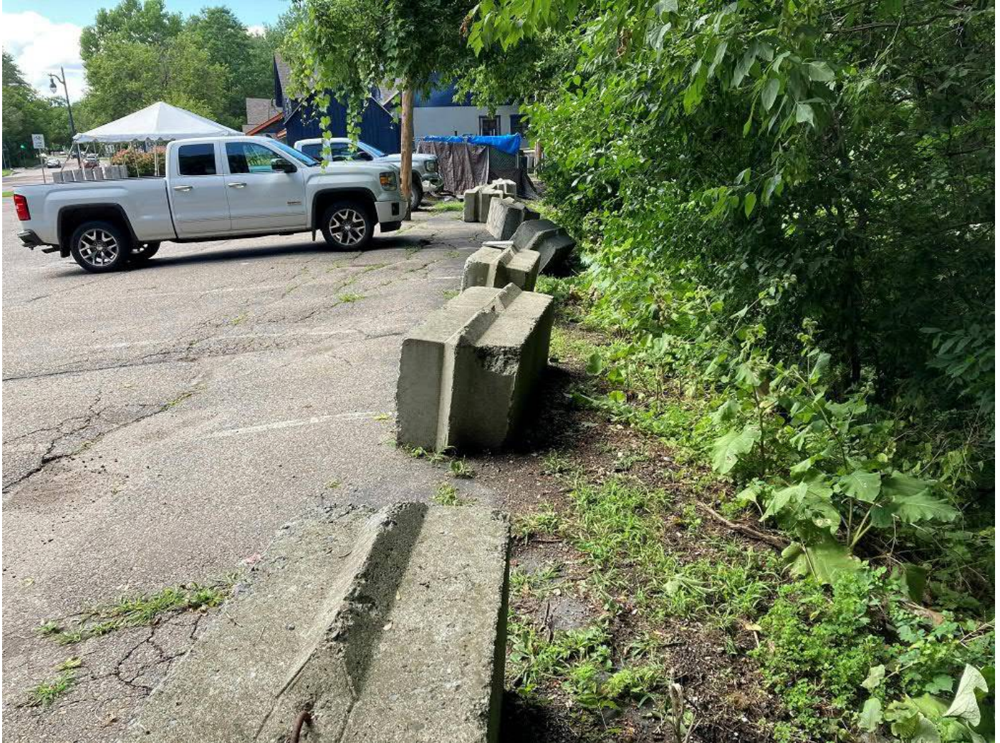
Photograph 10: View to west toward Bluebird BBQ building showing top of slope at eastern parking lot; asphalt parking most likely sloped to induce surface flow away from slope; note lean of blocks at top center, a possible expression of incipient surface slumping and slope cutback
