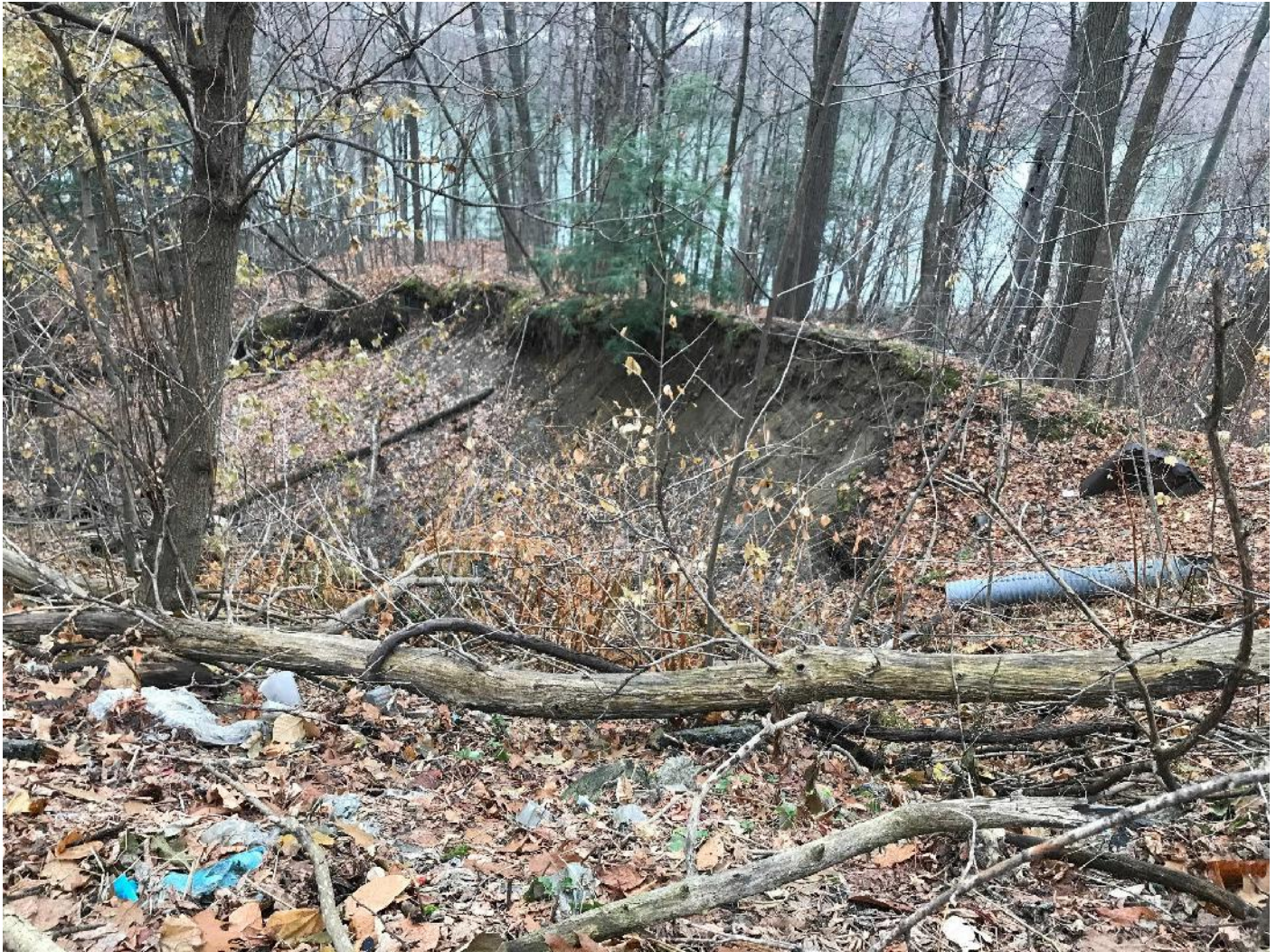
Photograph 9: View to north of gully shown in Photographs 7 and 8, taken in December 2019 during slope inspection conducted by Hoyle Tanner Associates; note significant difference in density of winter vs. summer vegetation; exposed side slopes will continue to erode during discharge events as base of slope erodes and collapses.
