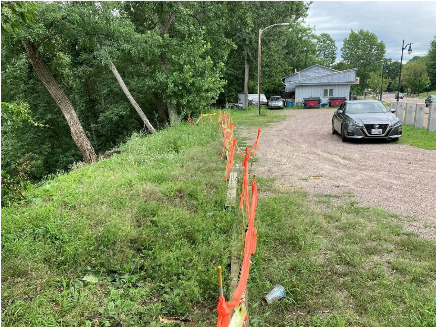
Photograph 24: View to east towards Hall's Hitches and Welding showing stable platform to right of flagging (i.e. no evidence of surface slumping or cracking) and top of failed slope at extreme left; note lean of trees top left; note monitoring well center right
