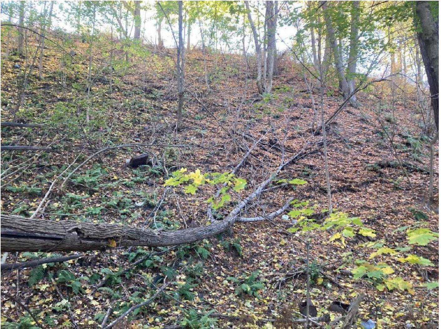
Photograph 18: View to southwest of slope west of Culvert 3 pipe showing exposed soil surface exposed to erosion during precipitation events; exposed surfaces will continue to erode; note no distinct lean of trees at mid and top of slope.
