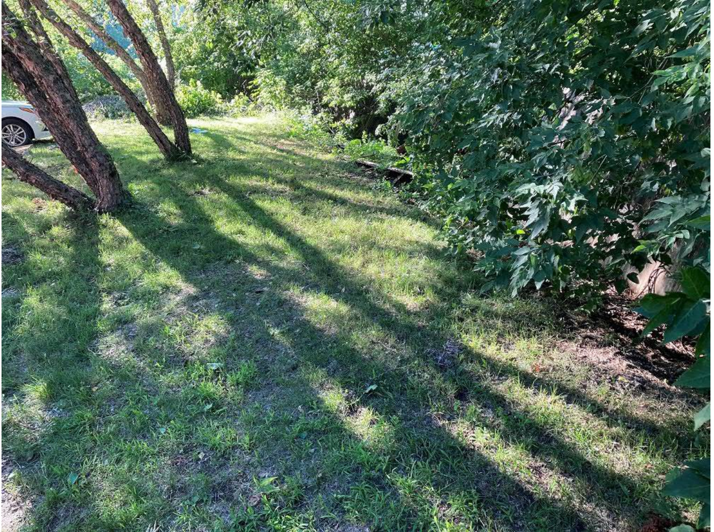
Photograph 2: View to west of Kismayo Kitchen building showing beginning of scarp formation at top of slope and irregular ground indicative of incipient slumping; note direction of lean of trees at upper left
