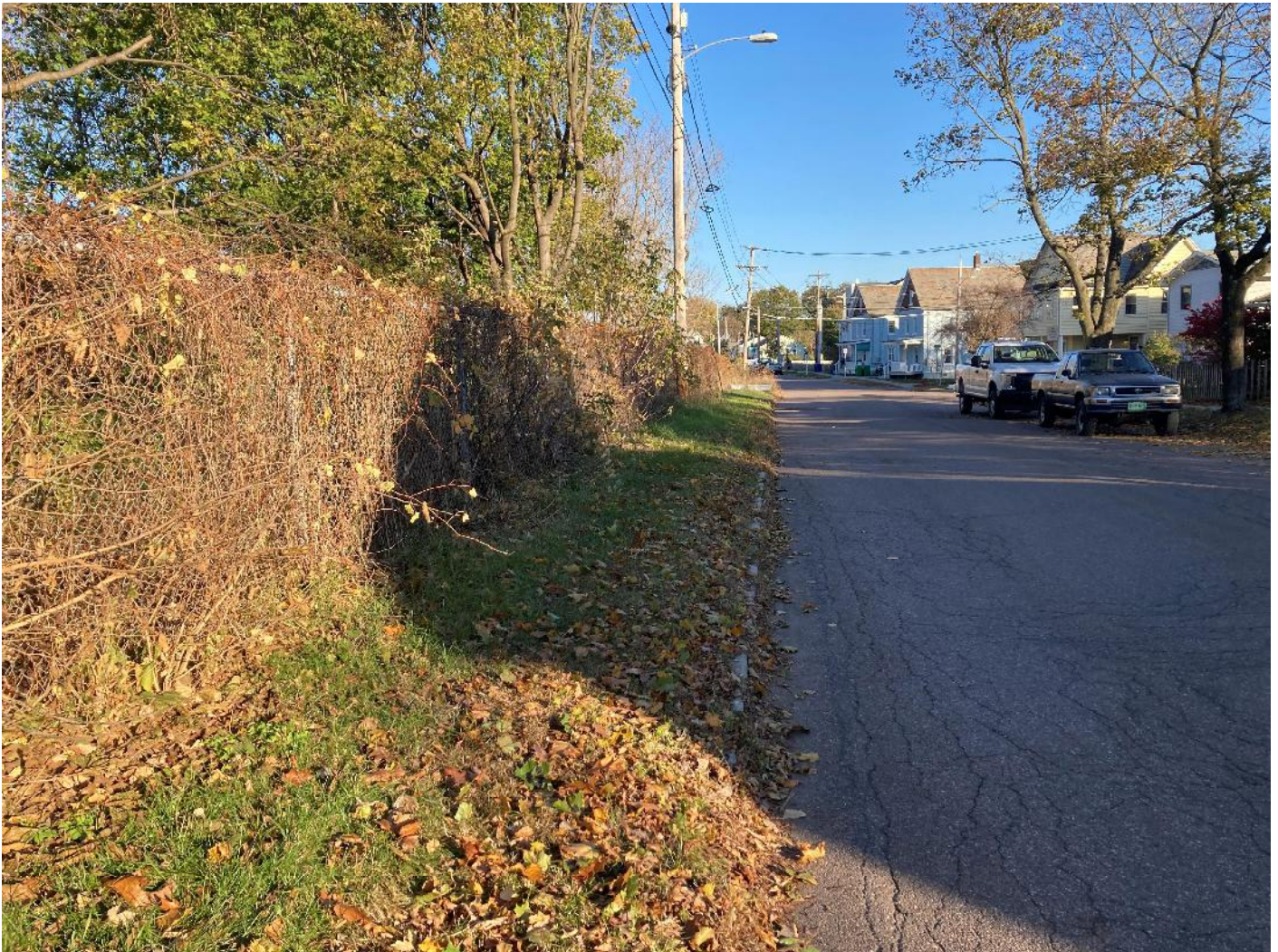
Photograph 30: View to east along Manhattan Drive at the top of the slope; no distinct scarps or disturbed ground observed; note stressed pavement cracking.
