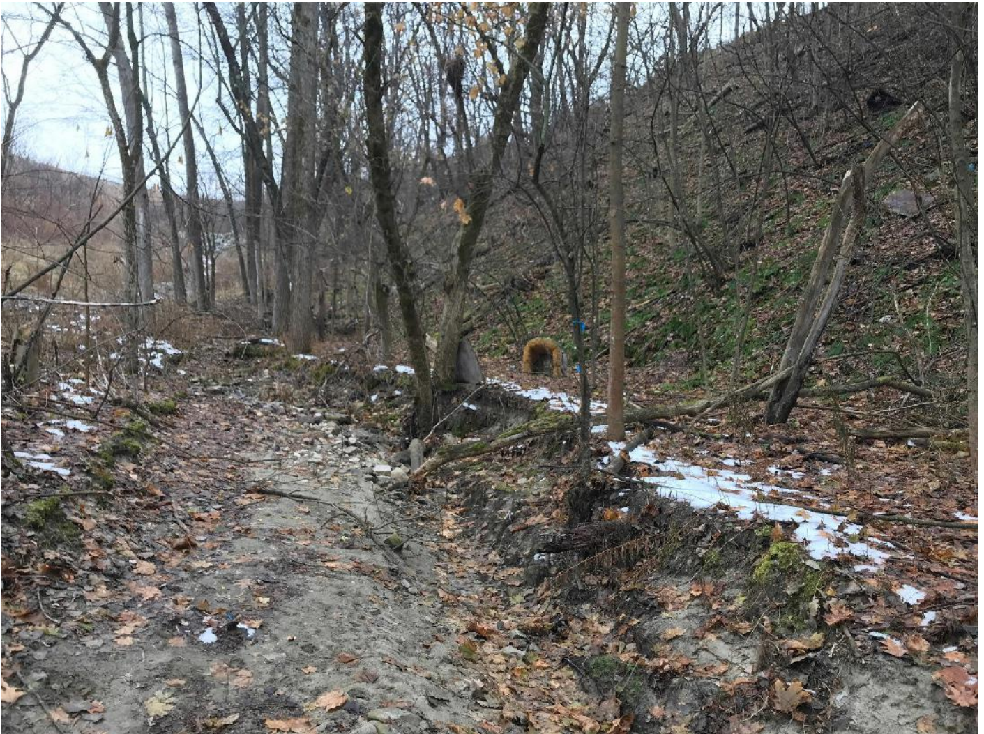
Photograph 12: View to east taken by Hoyle, Tanner & Associates in November 2019 showing toe of slope west of Culvert 2 and east of Culvert 3; unlined discharge channel from Culverts 1 and 2 in foreground; note intensity of erosion from surface flow cutting back towards toe of the slope.
