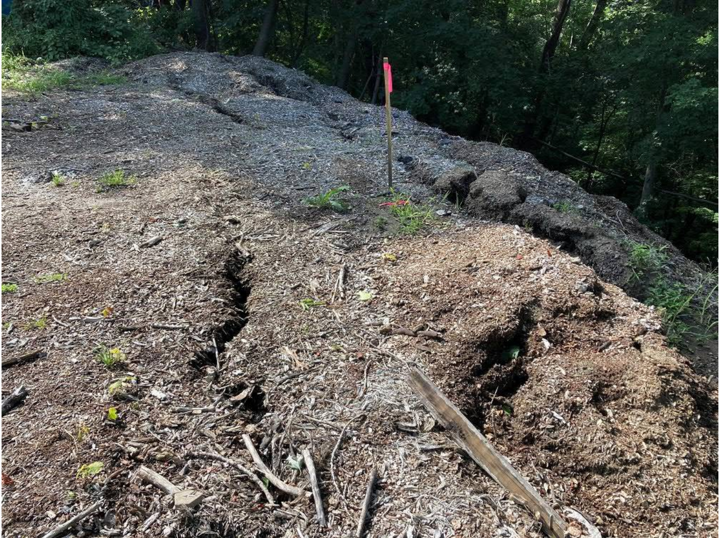
Photograph 5: View to west northwest, east of Burlington Collision building, showing crown cracks and beginning of future slump/slide, at top of former failed slope
