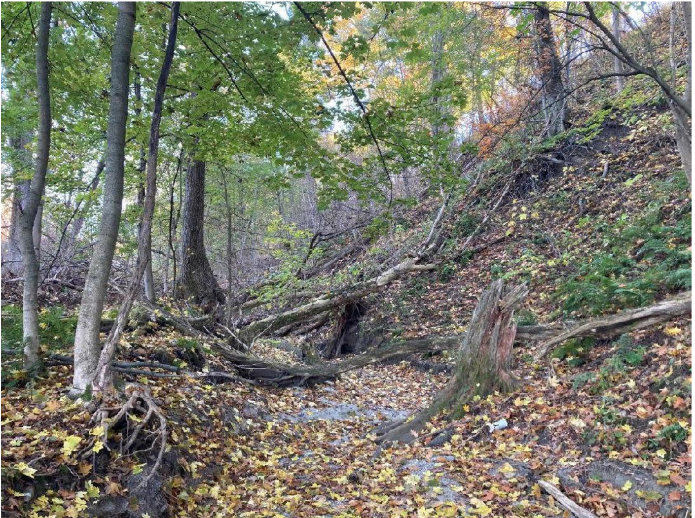
Photograph 25: View to east showing erosion channel and failed lower portion of slope west of Culvert 4 pipe.
