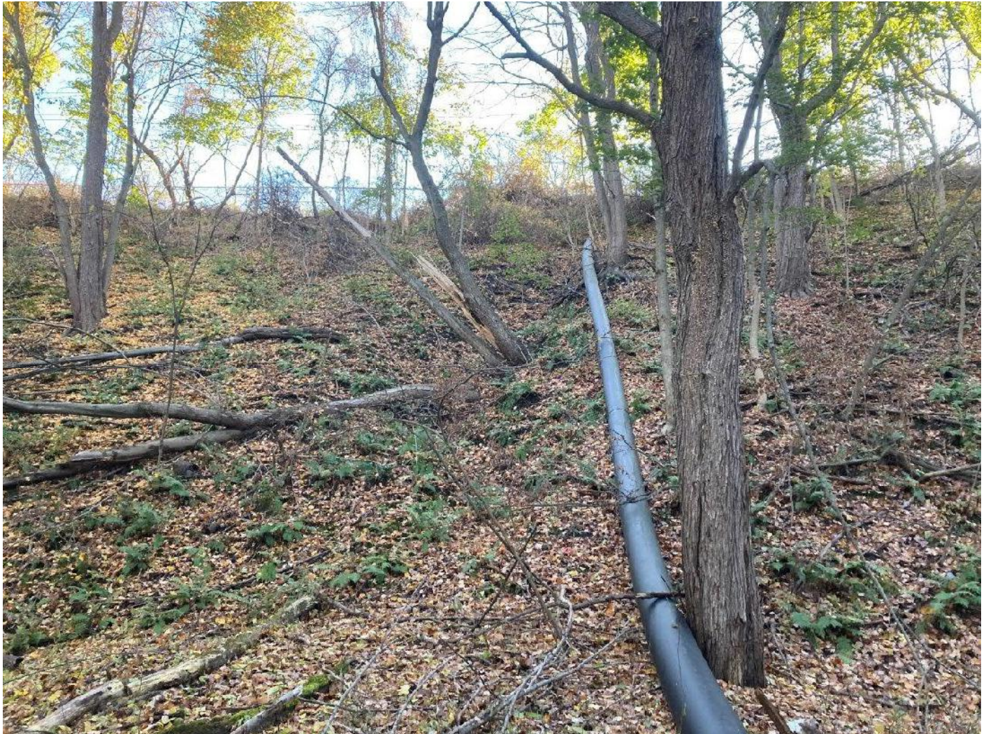
Photograph 14: View to south towards Manhattan Drive showing exposed discharge pipe to Culvert 3, and soil erosion and gully formation at top and mid-slope.
