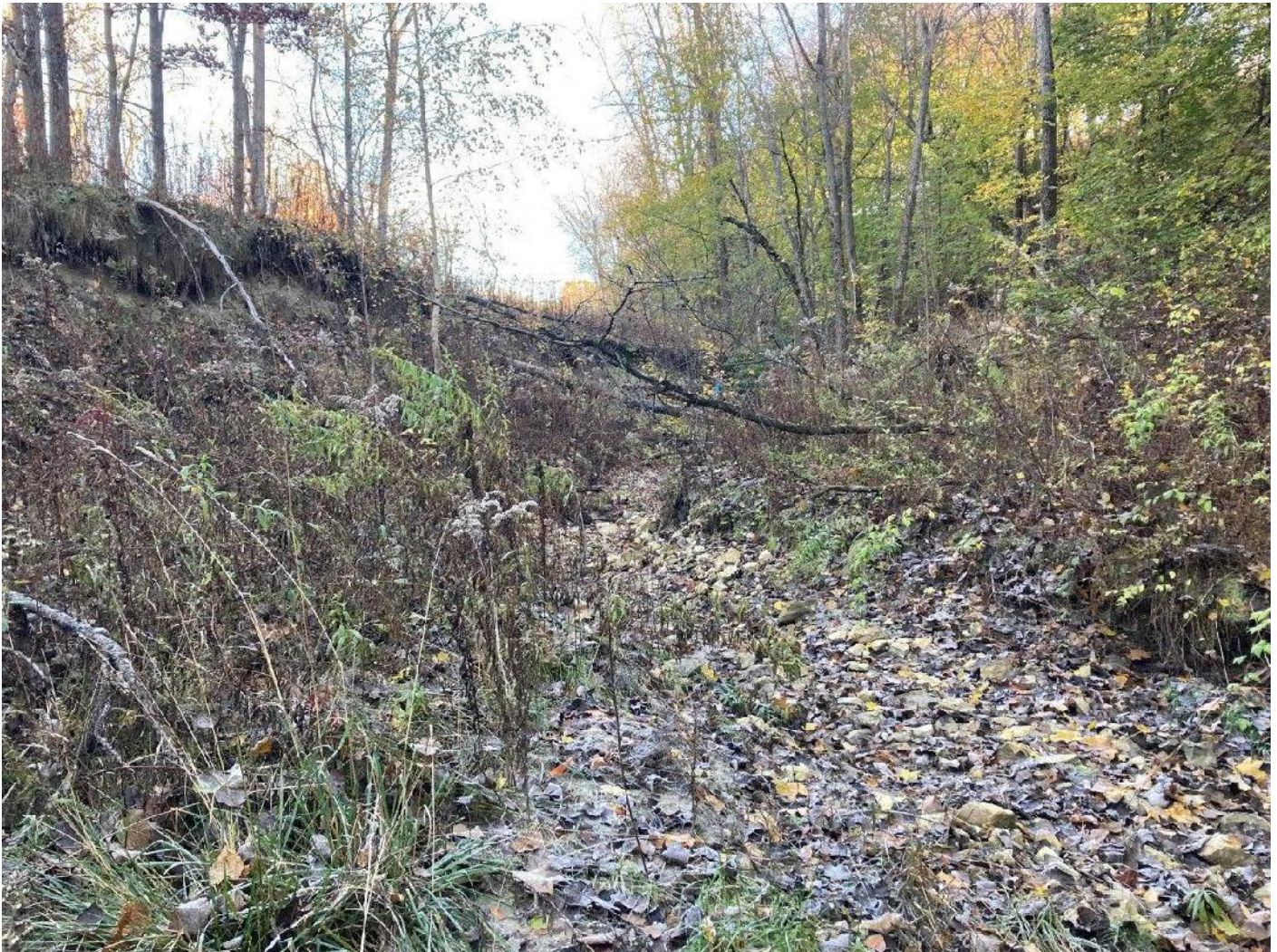
Photograph 22: View to east from position of Photograph 21 showing large erosional gully north of toe of Manhattan Drive slope.
