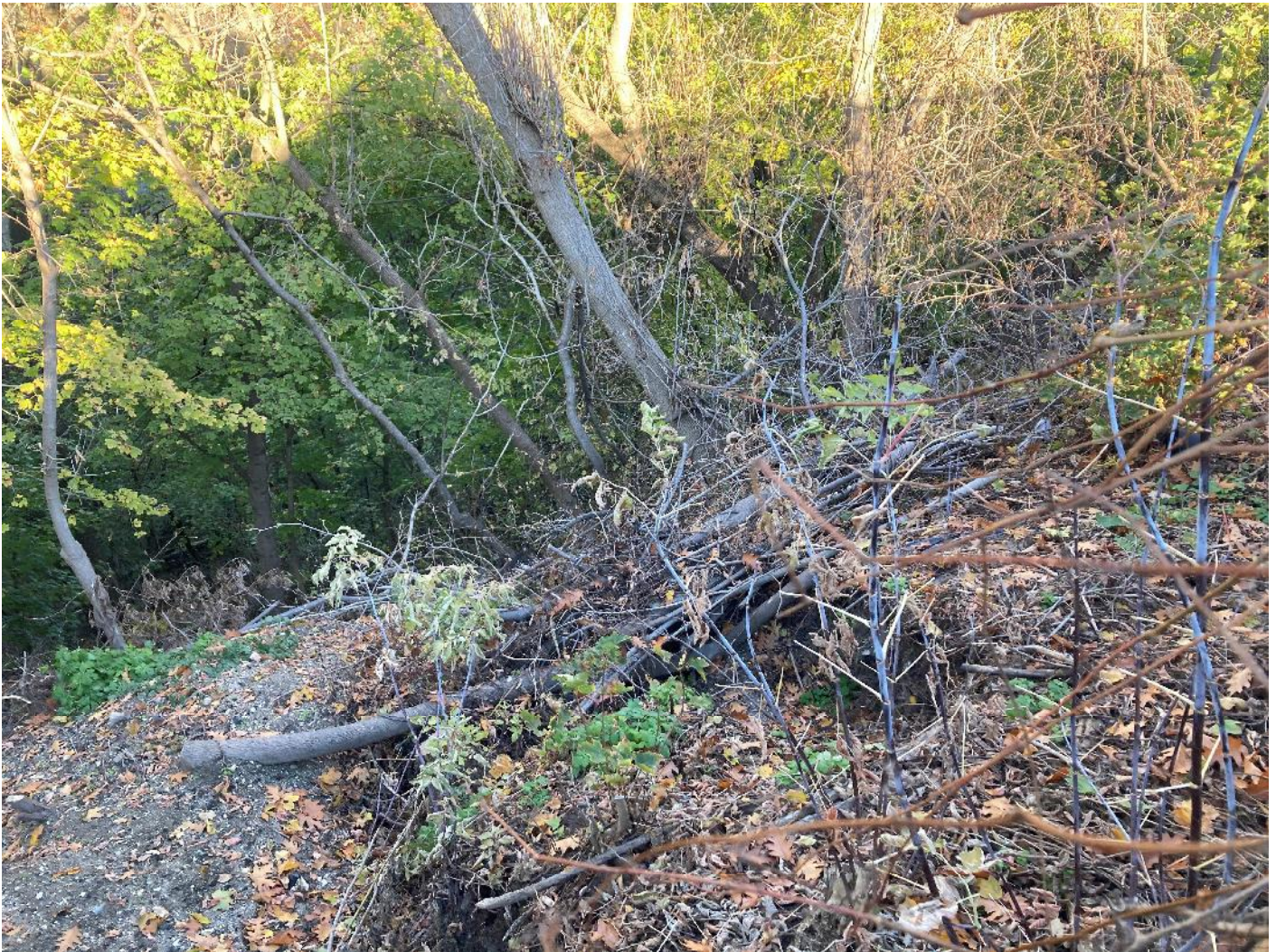
Photograph 29: View to north from top of slope on Manhattan Drive showing minor surface failure; note lean of trees at center of photo and exposed soil at bottom right.
