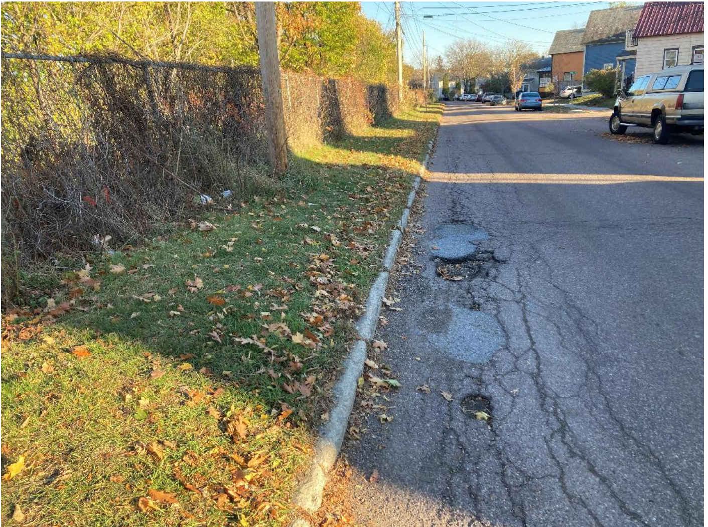
Photograph 28: View to east along Manhattan Drive from Convent Square at top of slope; no distinct ground disturbance observed; stressed asphalt cracking may be a result of slope creep?
