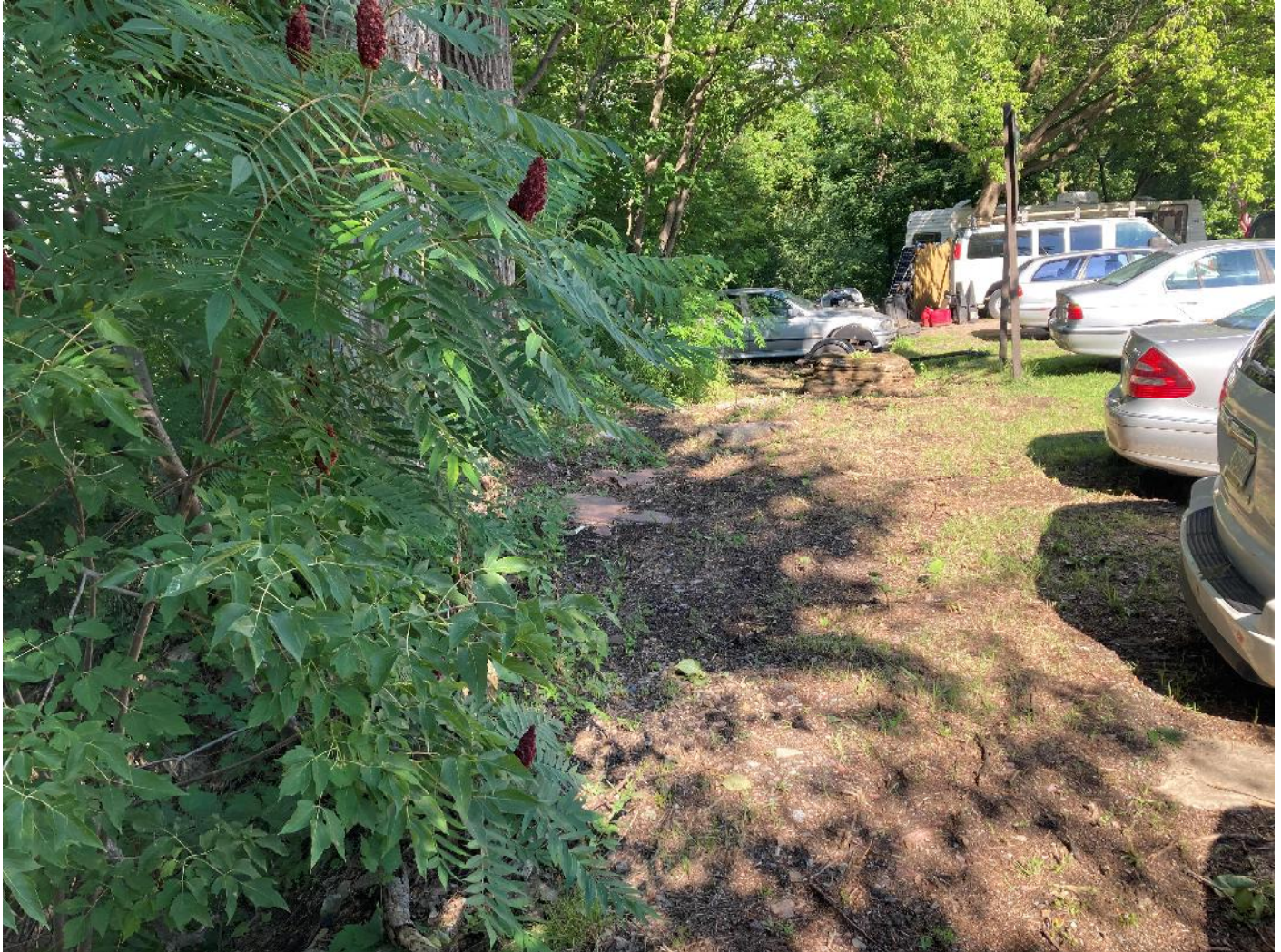
Photograph 23: View to east showing eastern portion of Michael's Auto Sales property; poorly vegetated area subject to continual surface erosion at the top of the slope and downslope; soil scarp from historic failures obscured by vegetation at left of photograph.
