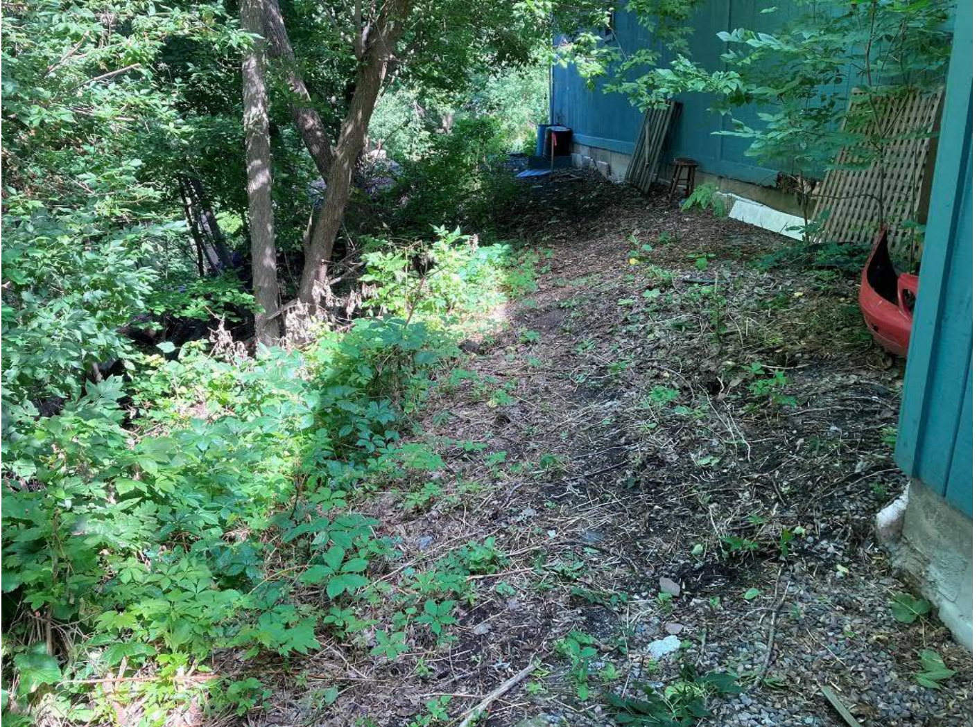
Photograph 1: View to east behind Burlington Collision showing incipient slumping (center and center foreground) of photograph) at top of slope; note leaning trees top left
