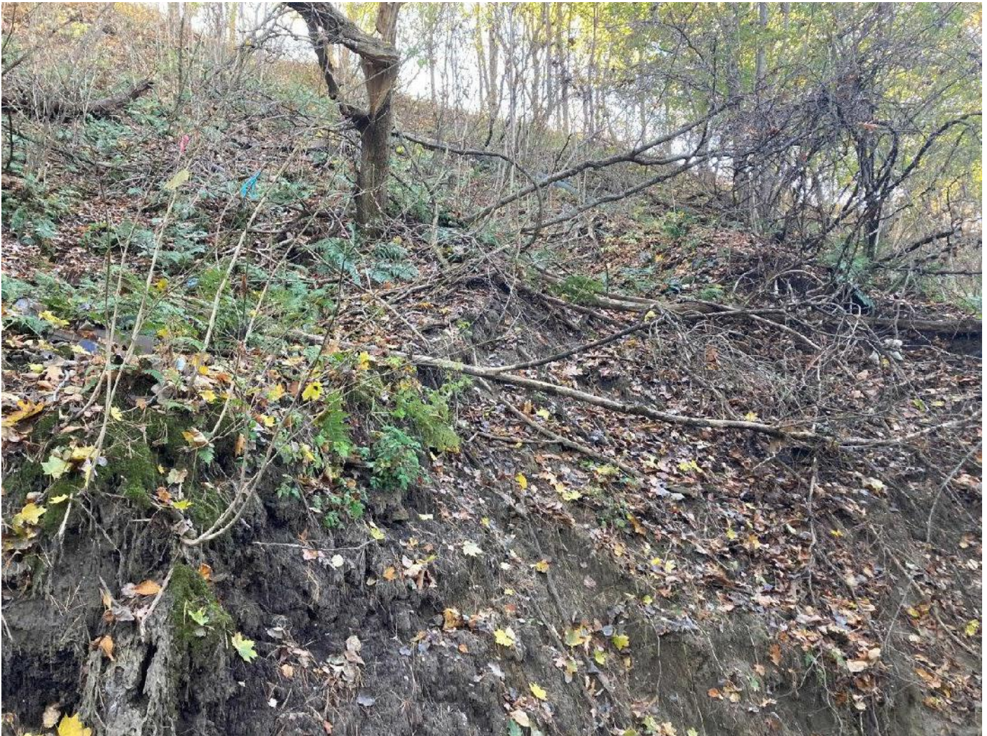
Photograph 23: View to southwest from toe of slope showing discharge pipe from Manhattan Drive at top-center (designated herein as Culvert 4) and failure/erosional surface in foreground at toe of slope; failure a result of historical heavy surface flow cutting into toe of slope;
