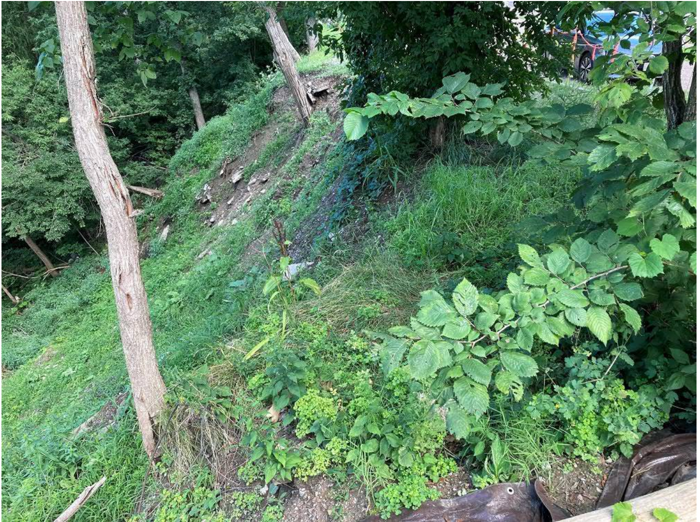
Photograph 20: View to east of soil slide east of residence, looking towards property at 365 Riverside Avenue; note leaning tree top center (see inspection report for 365 Riverside Avenue for additional photographs); exposed surfaces subject to localized failure and erosion during precipitation events
