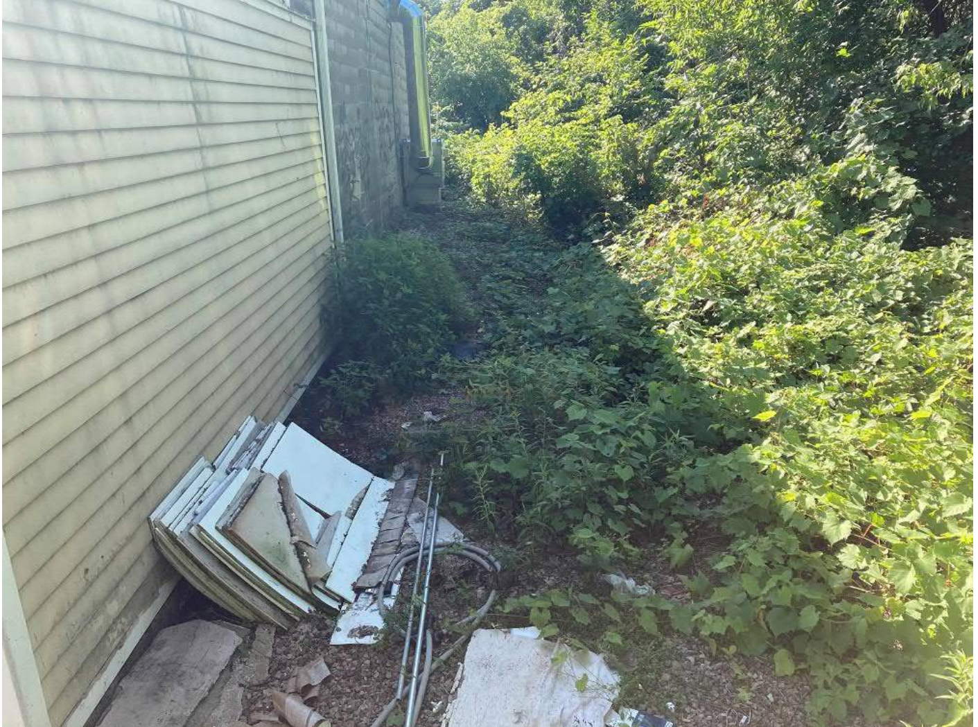
Photograph 12: View to west behind GBG Indian Kitchen showing slight irregular surface and incipient slumping at center of photograph obscured by vegetation; exposed soil scarp to right of photograph is also obscured by dense vegetation (see Photograph 15).
