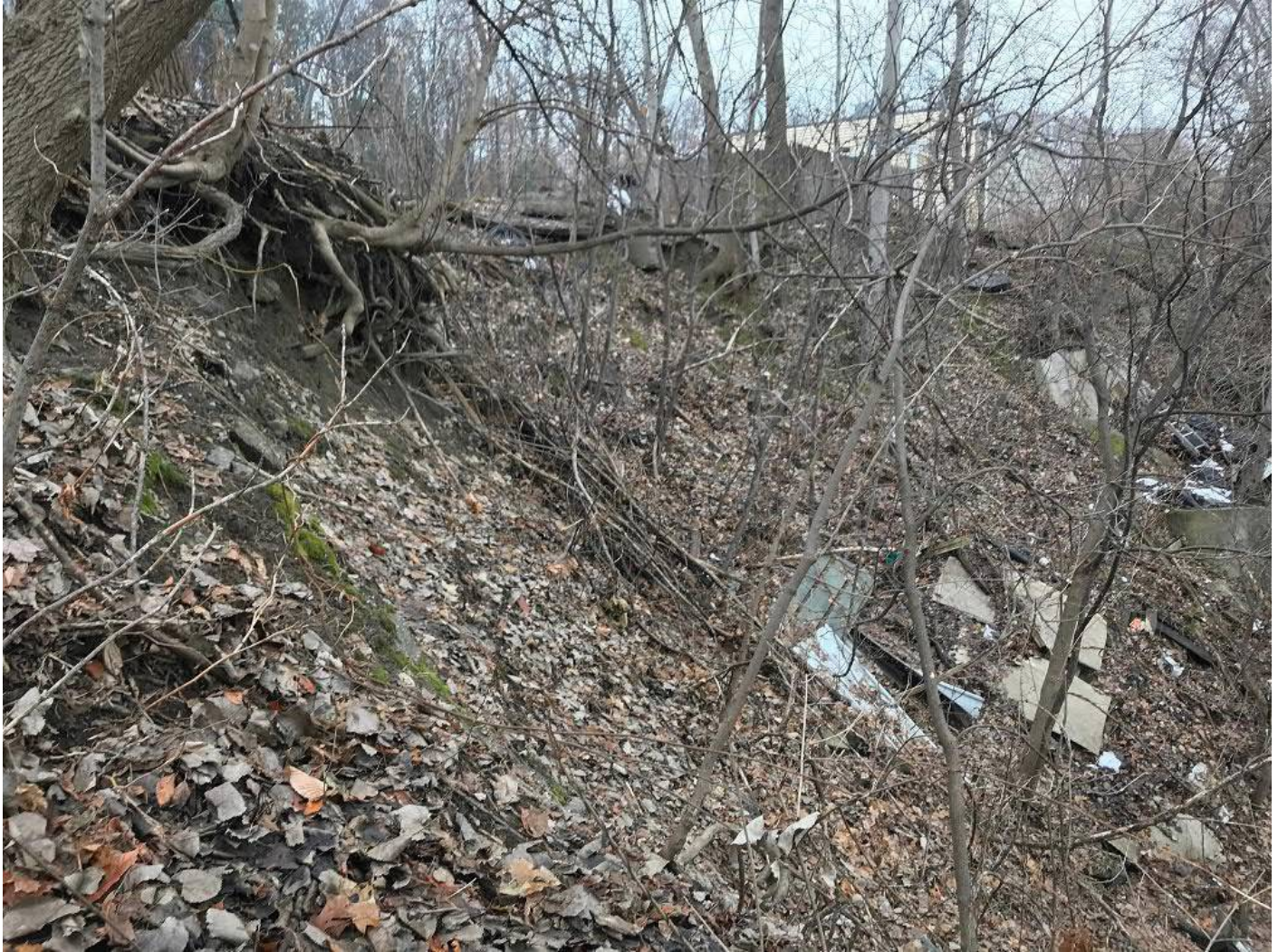
Photograph 17: View to southwest showing GBG Indian Kitchen (top right), and failure scarp top left; photograph taken in December 2019 during inspection by Hoyle-Tanner Associates; note change in density of vegetation; exposed slope subject to surface erosion during precipitation events
