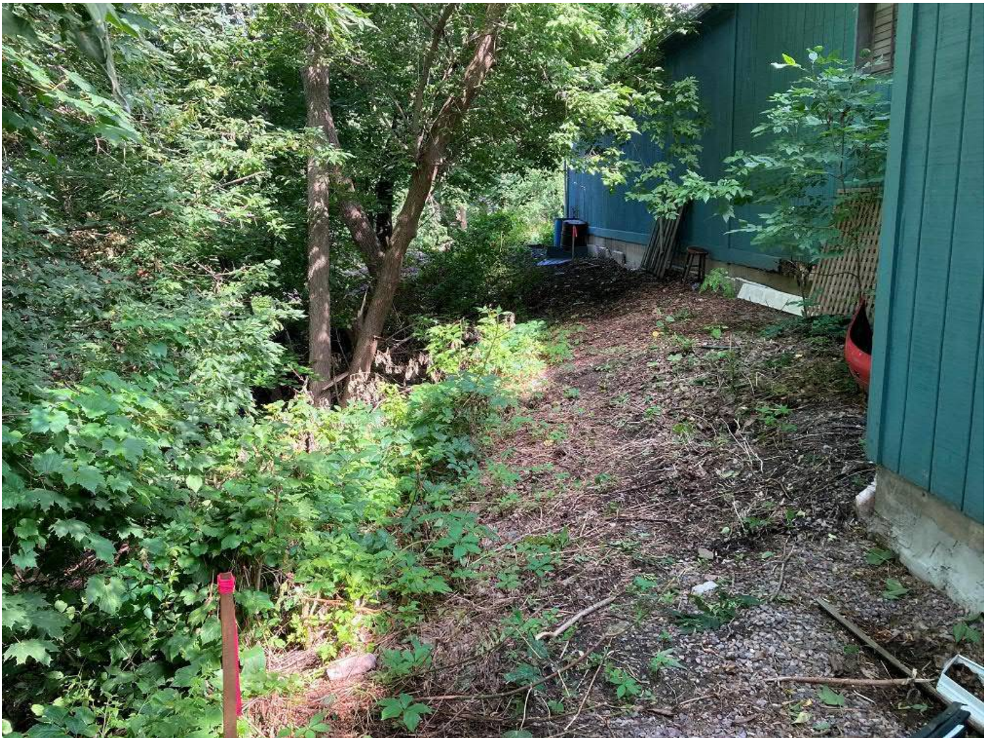
Photograph 2: Additional view of incipient slumping behind Burlington Collision Building
