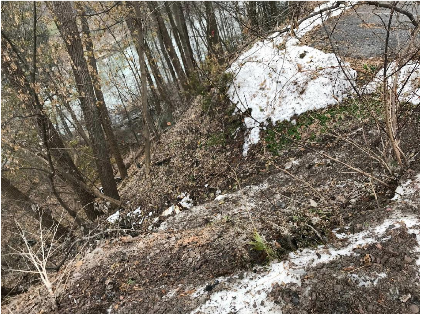
Photograph 31: View to northwest, downslope, taken by Hoyle Tanner Associates during the December 2019 inspection showing the boundary between 365 and 317 Riverside Avenue (Bluebird BBQ); note gully formation from surface runoff at center of photograph and possible crown cracking at bottom right; western parking area for Bluebird BBQ at top right
