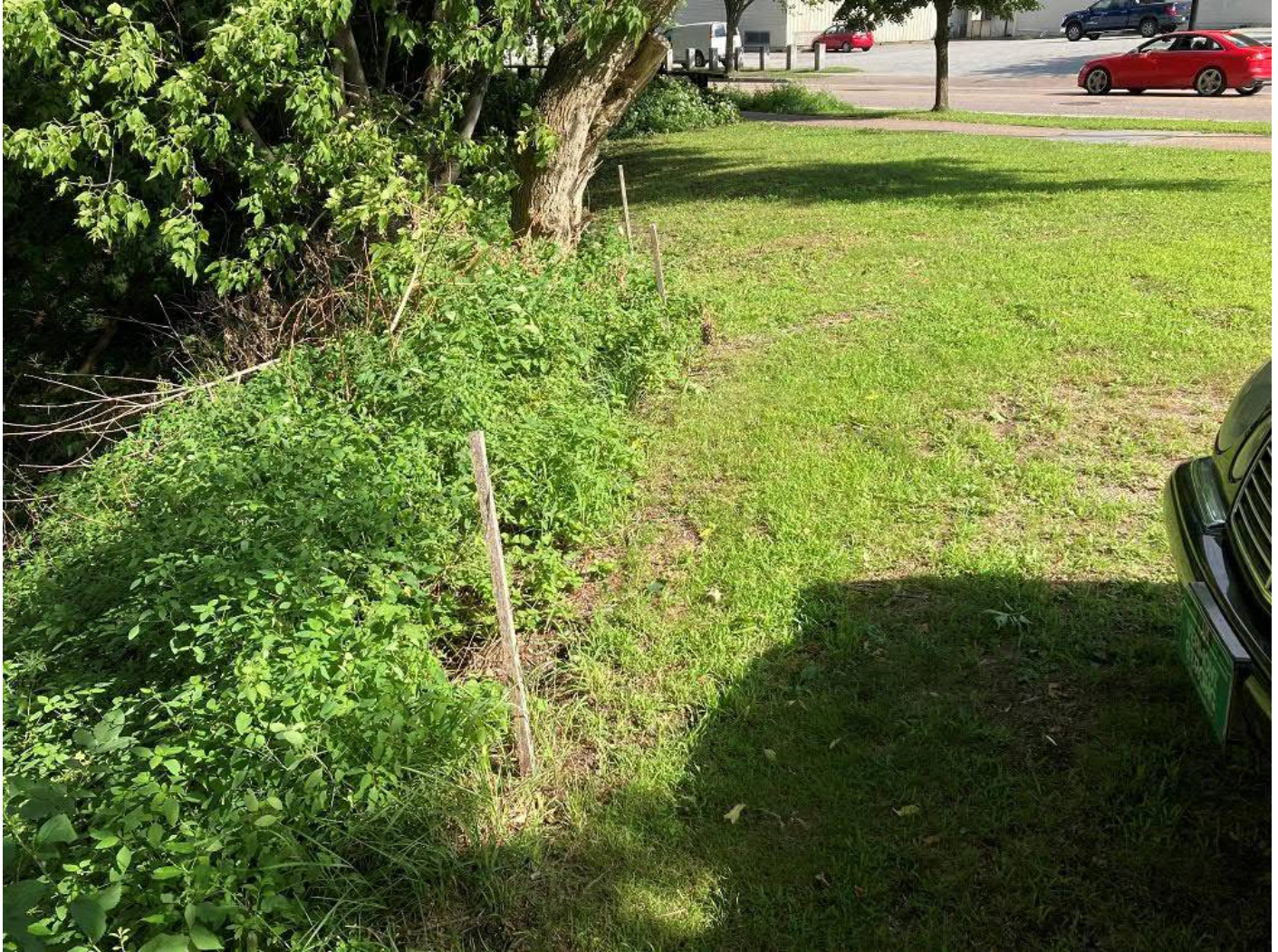
Photograph 20: View to southeast from eastern portion of Michael's Auto Sales property showing beginning of scarp formation at stakes; historic failure scarp obscured by vegetation at left of photograph.
