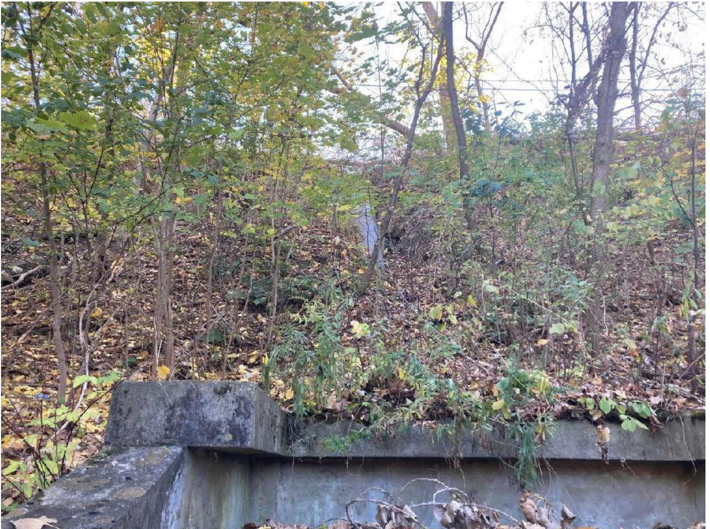
Photograph 5: View to south towards Manhattan Drive of stormwater discharge pipe and top of culvert (designated herein as Culvert 2); note soil erosion around exposed pipe.
