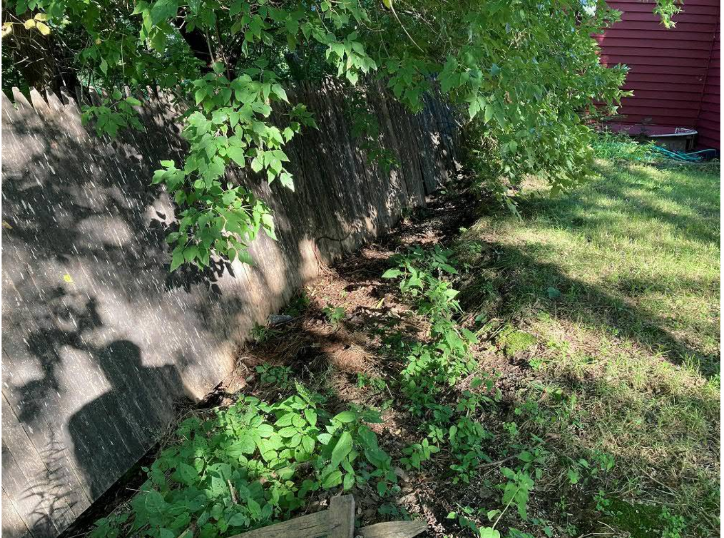
Photograph 1: View to east of scarp formation at top of slope west of Kismayo Kitchen building; note failure of wooden fence
