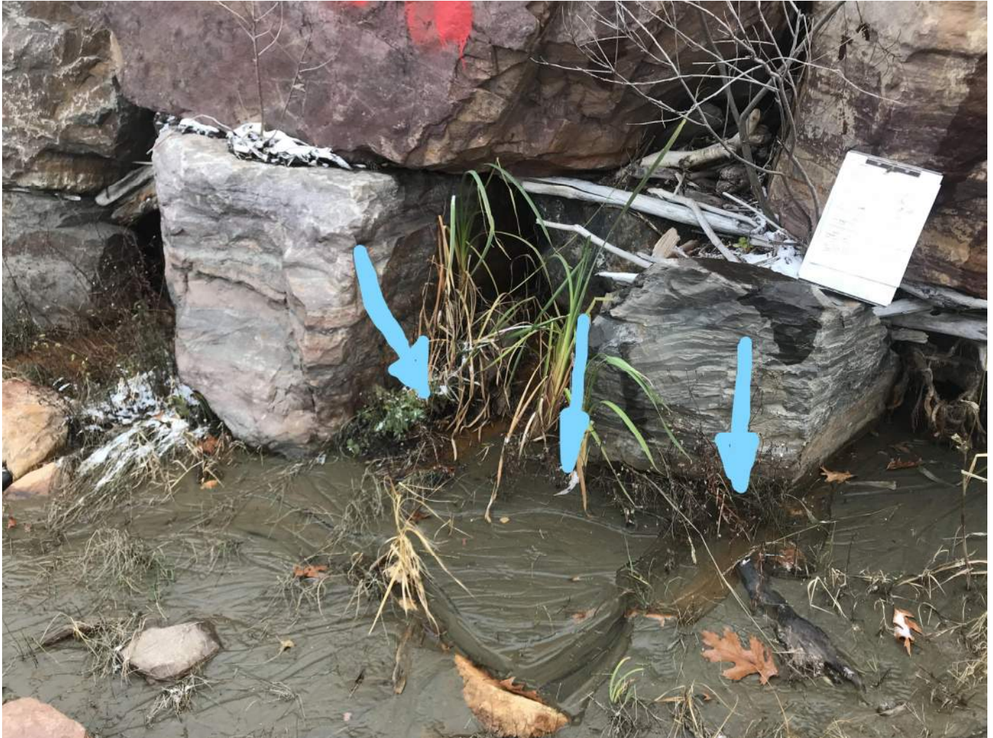
Photograph 8: View to east; seepage at base of rip-rap and basal blocks of remediated slope
