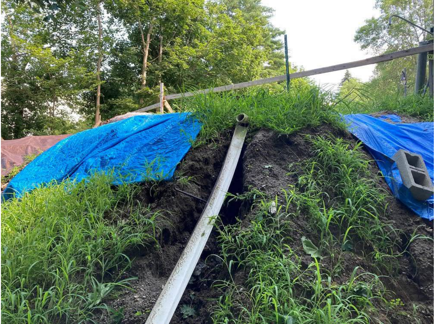
Photograph 15: View to southeast, east of residence, showing discharge pipe; ongoing discharge flow will contribute to surface erosion and creation of flow gully in unvegetated portions downslope
