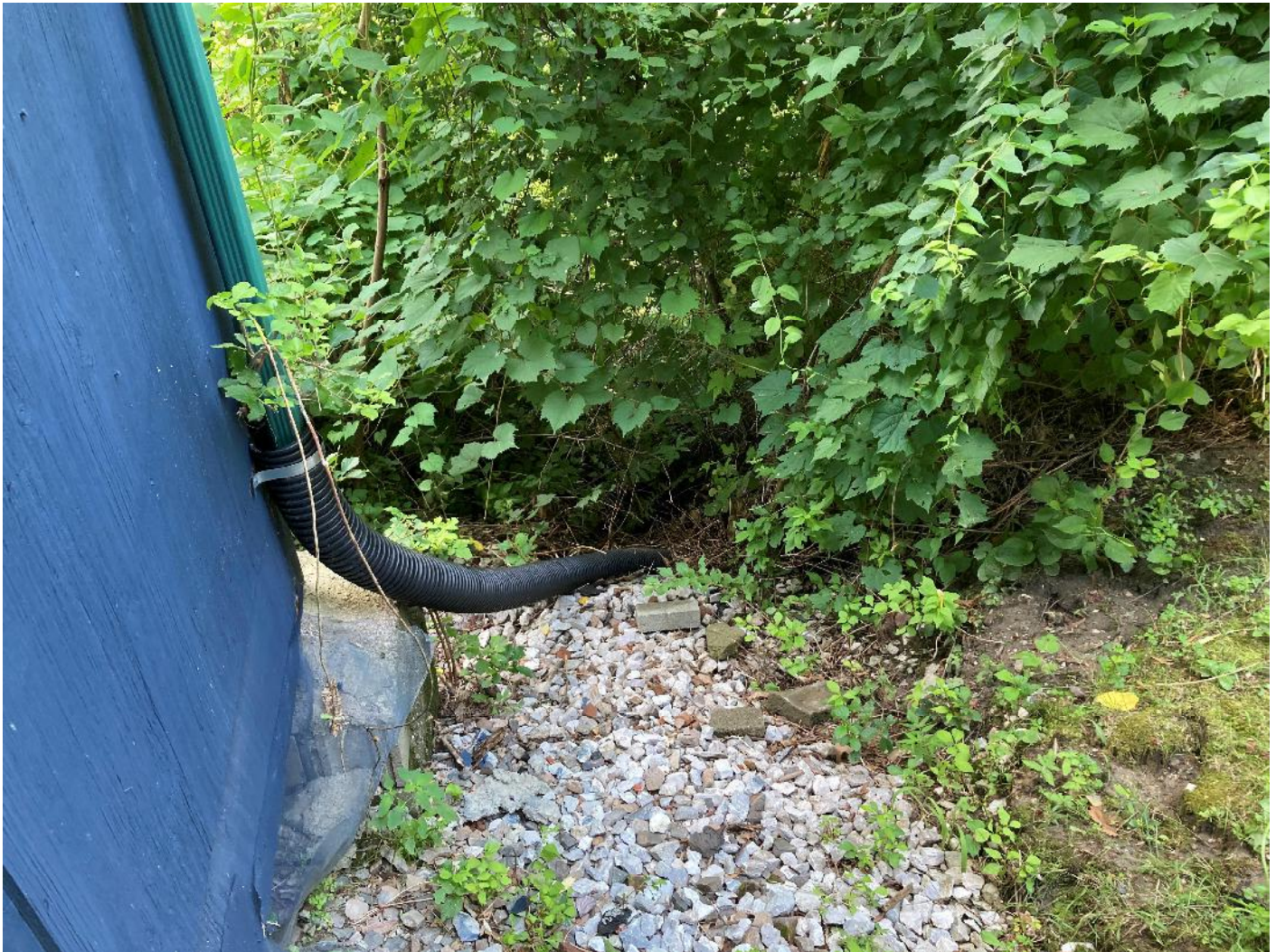
Photograph 8: View to north downslope showing stormwater discharge hose from Bluebird BBQ building; discharge of water downslope has caused surface soil erosion (see Photo 14)
