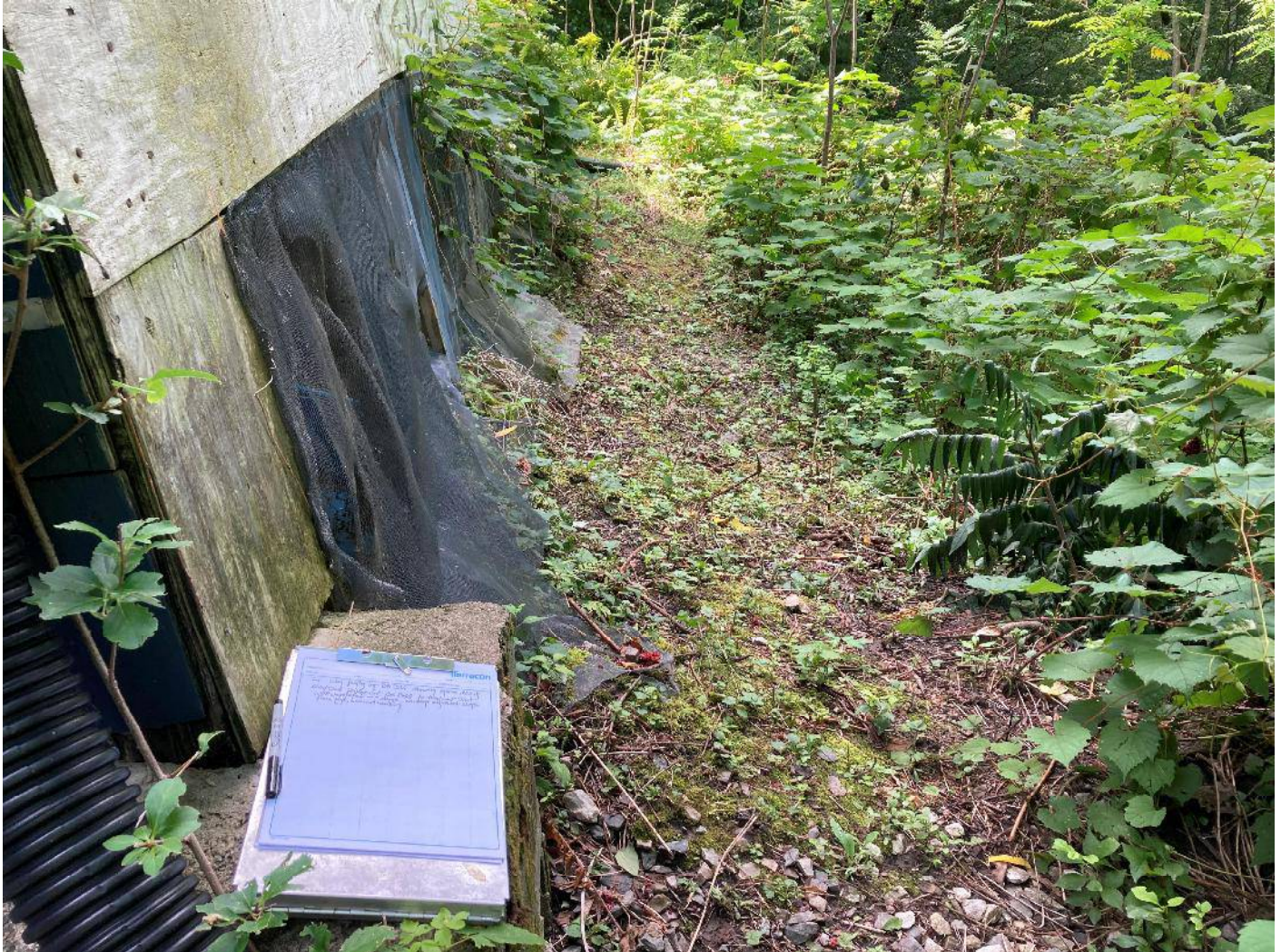
Photograph 6: View to west behind Bluebird BBQ building; note curvature at top of slope but no distinct slump or crack formation at surface; soil scarp obscured by vegetation at right of photograph
