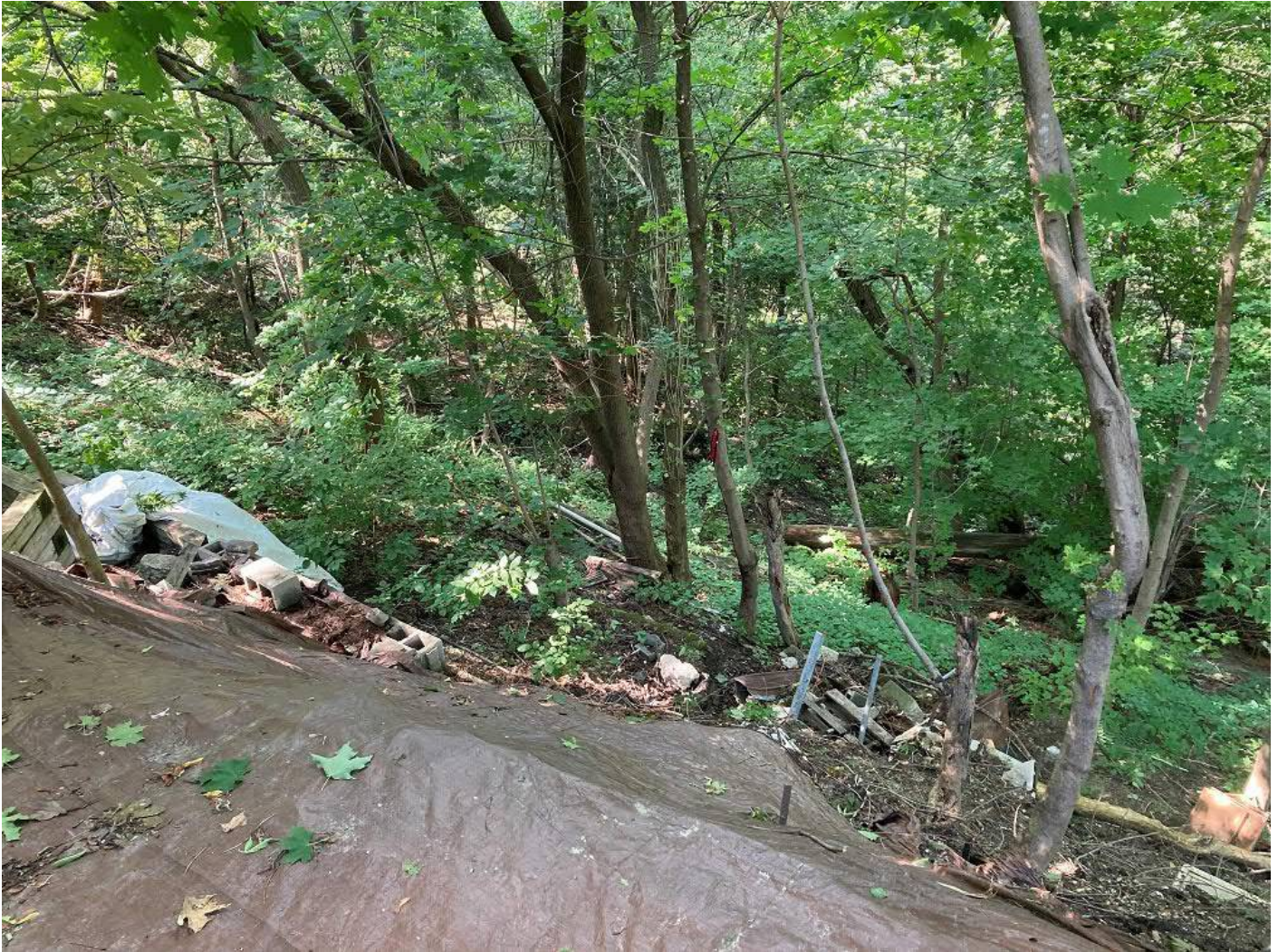
Photograph 13: View to southwest behind residence showing covered scarp at top of slope and head scarp of historic soil slump downslope; note lean of trees upslope at center and left-center of photograph
