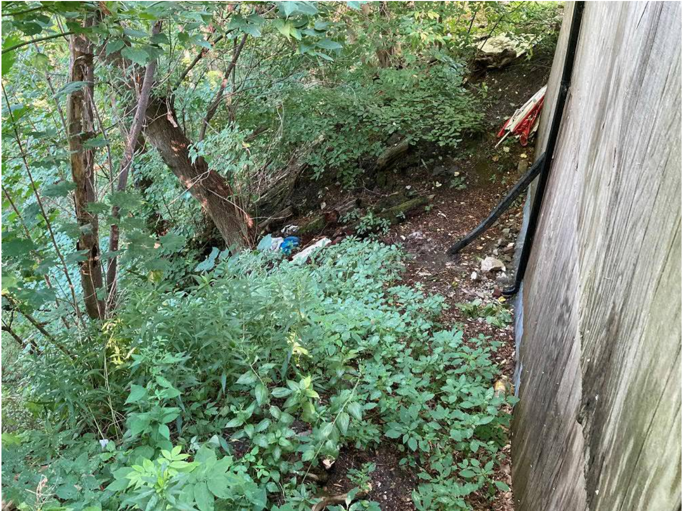
Photograph 3: View behind Kismayo Kitchen building showing erosion gully from surface runoff; soil will continue to erode during precipitation events; note location of downspout; note lean of tree left center of photograph; soil scarp at left obscured by vegetation.
