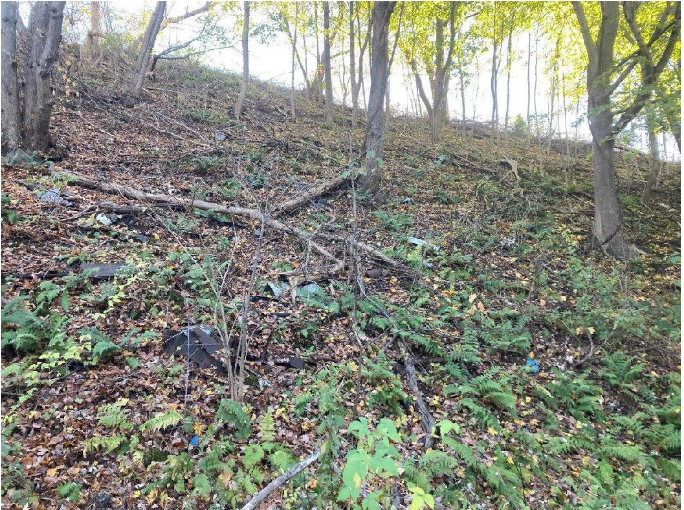
Photograph 9: View southwest from toe of slope, west of Photograph 8, showing surface soil erosion from sheet wash generated during heavy precipitation events; surface expression of gully formation beginning to appear; note lean of trees at top of slope (top center and top left).
