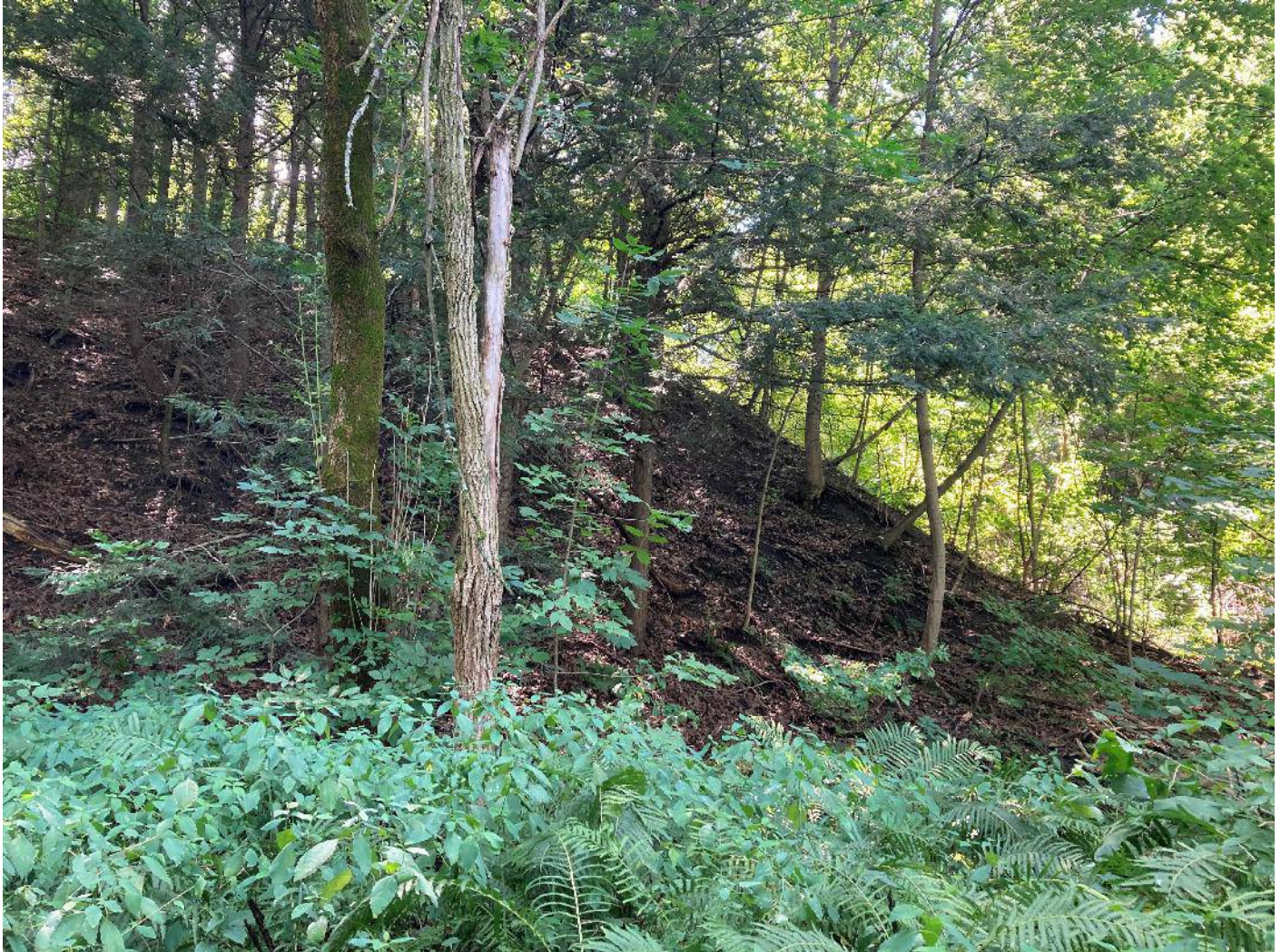
Photograph 18: View to west downslope from GBG Indian Kitchen (just south of River Walk Trail) showing soil slump debris from inferred historic failure event; exposed soil surfaces subject to continual surface erosion from precipitation events;
