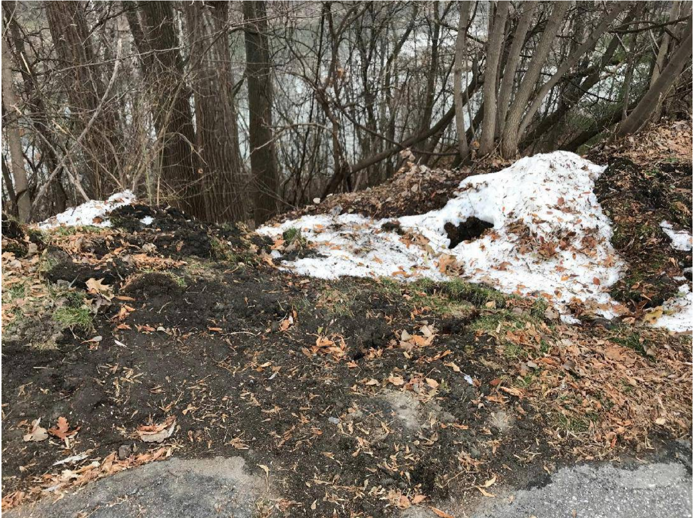
Photograph 4: View to northwest taken by Hoyle Tanner Associates during December 2019 inspection showing gully formation and surface cracking at top of slope at west parking lot of Bluebird BBQ
