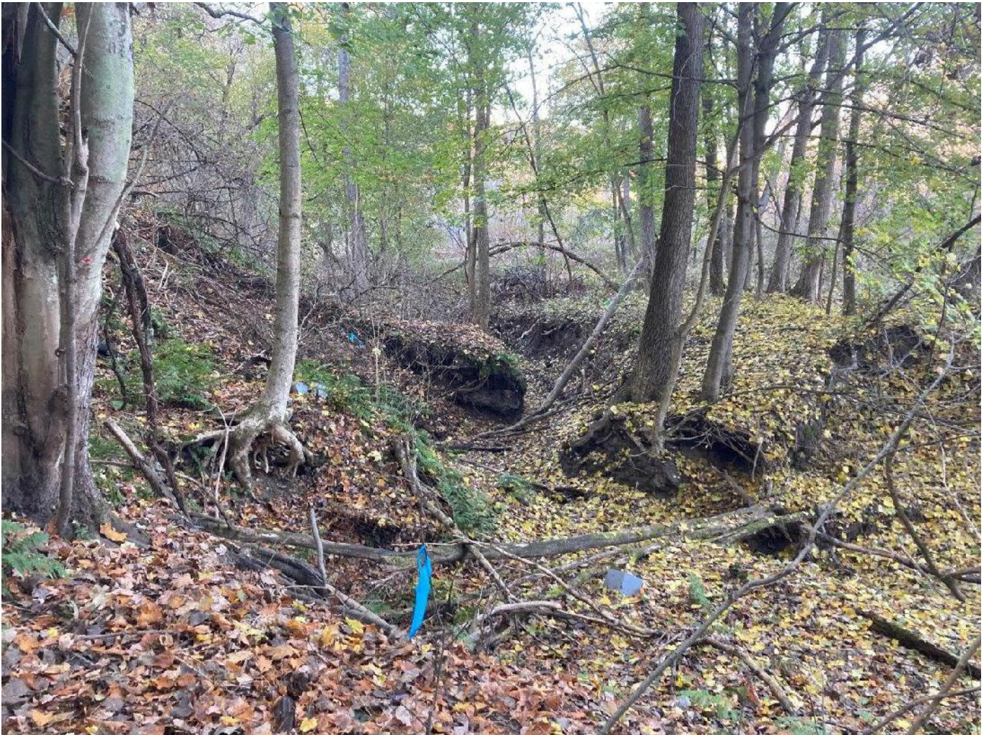
Photograph 21: View to west of erosion channel at the toe of the slope west of Culvert 3; failed lower portion of slope at left-center of photograph a result of erosion undercutting into the toe of the slope.
