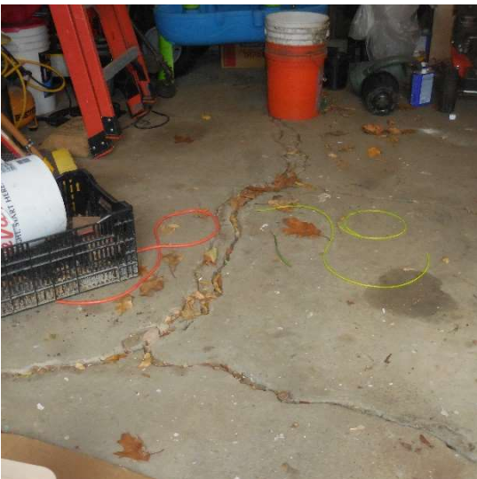
PHOTO 2: Slab - note extensive cracking and vertical displacement
