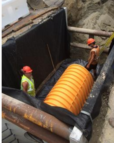
Allen St subsurface infiltration system
