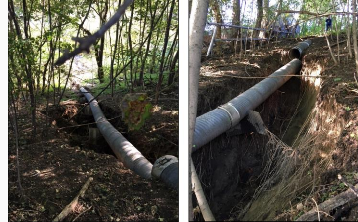
Gully erosion at IV8.0 – Fall 2018 (prior to emergency repair work)
