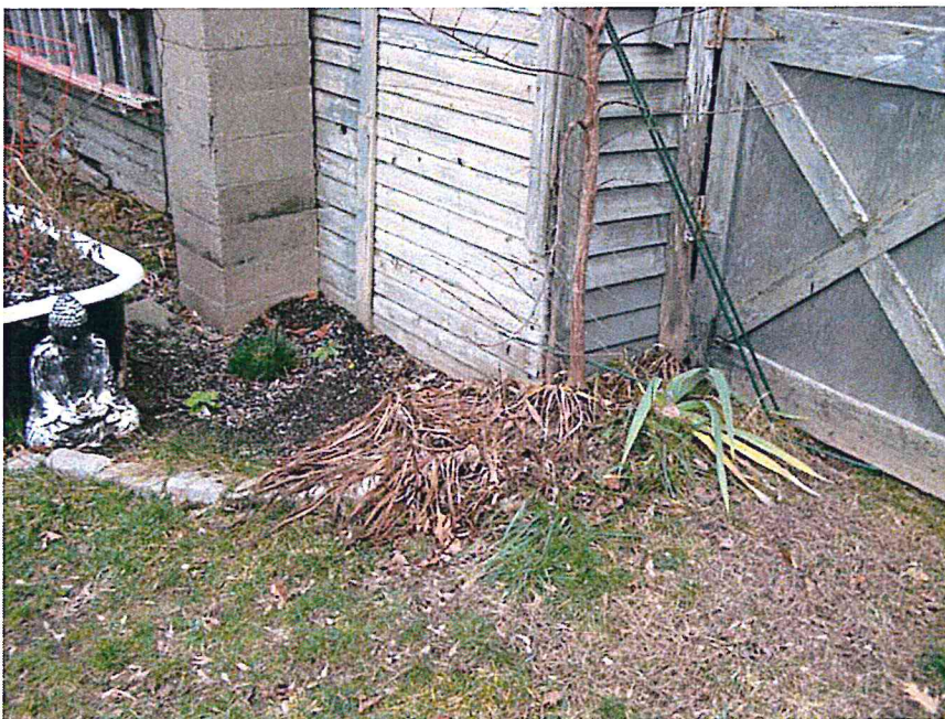
Photo 4 – Southwest corner of the shed. Exterior siding is in contact with the ground.
