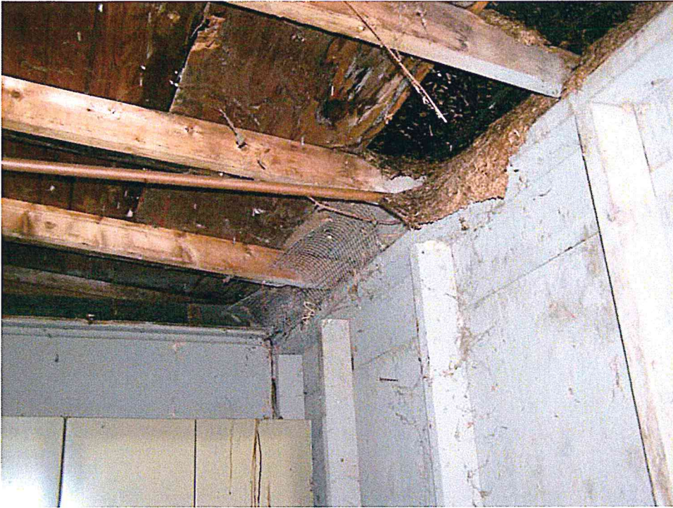
Photo 9 – West end of 2x4 roof rafters (spaced at 24"). Roof sheathing is deteriorated and leaks.
