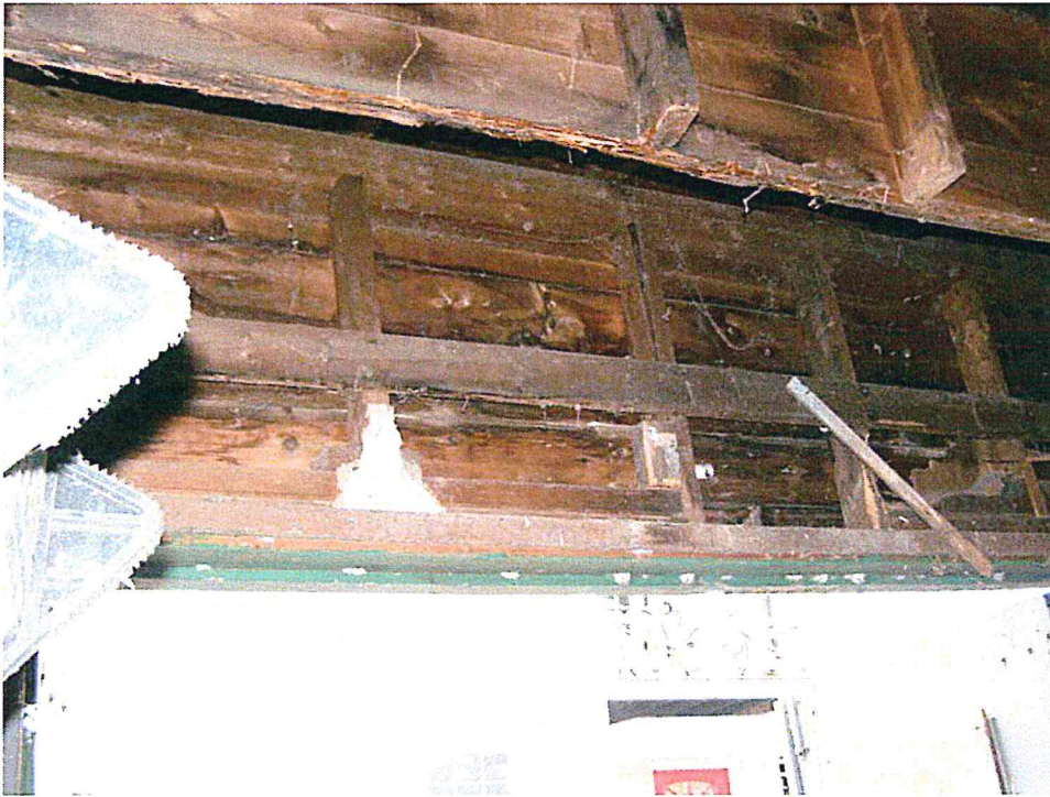
Photo 13 – No header at east wall over garage wall. East wall is a bearing wall for the roof framing.
