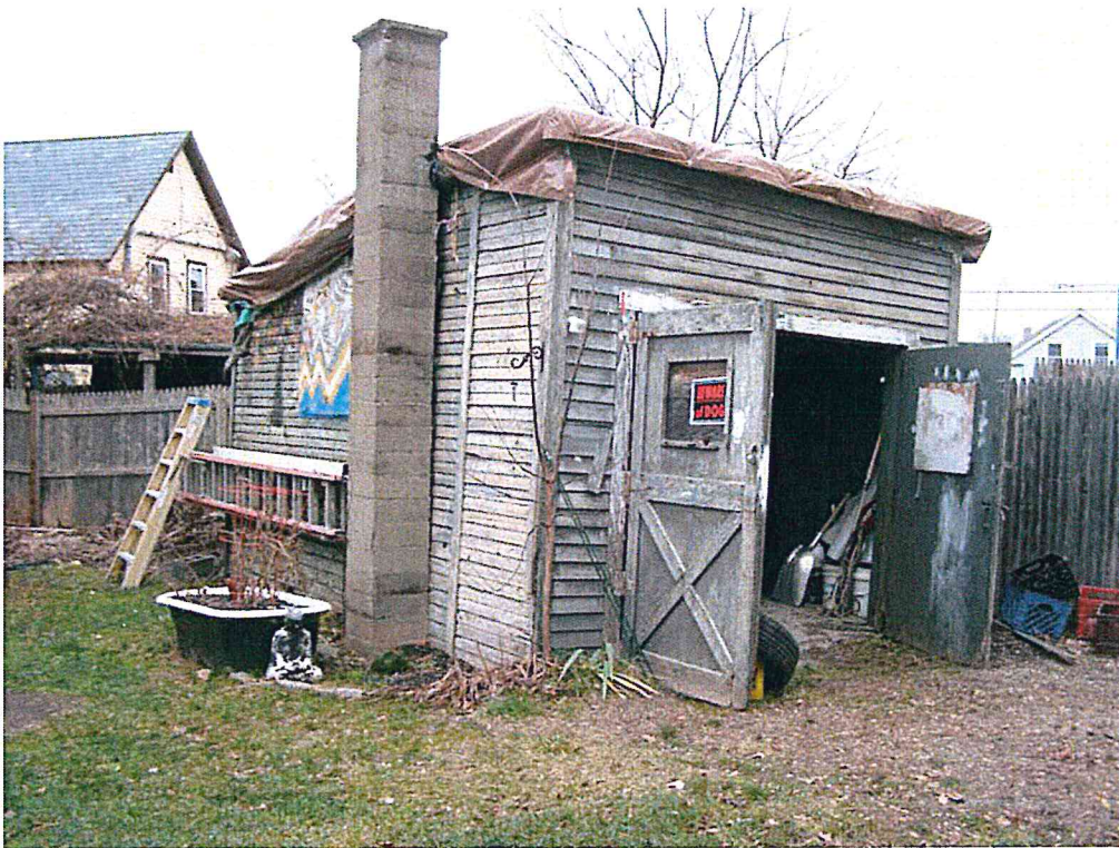
Photo 1 – East and south walls of the shed. The sheds leans significantly to the north.
