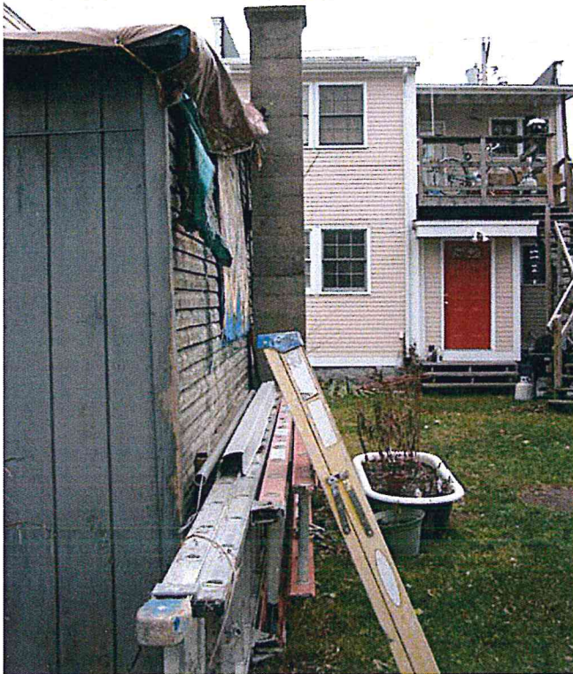
Photo 3 – Looking east along the south wall of the shed. There is a large gap between the chimney and the wall of the shed.
