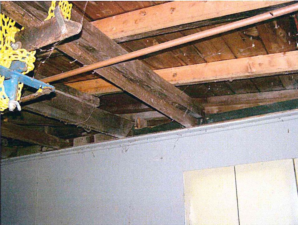
Photo 10 – Roof framing is 2x4 rafters at 24" spanning 18'. Rafters are not continuous.
