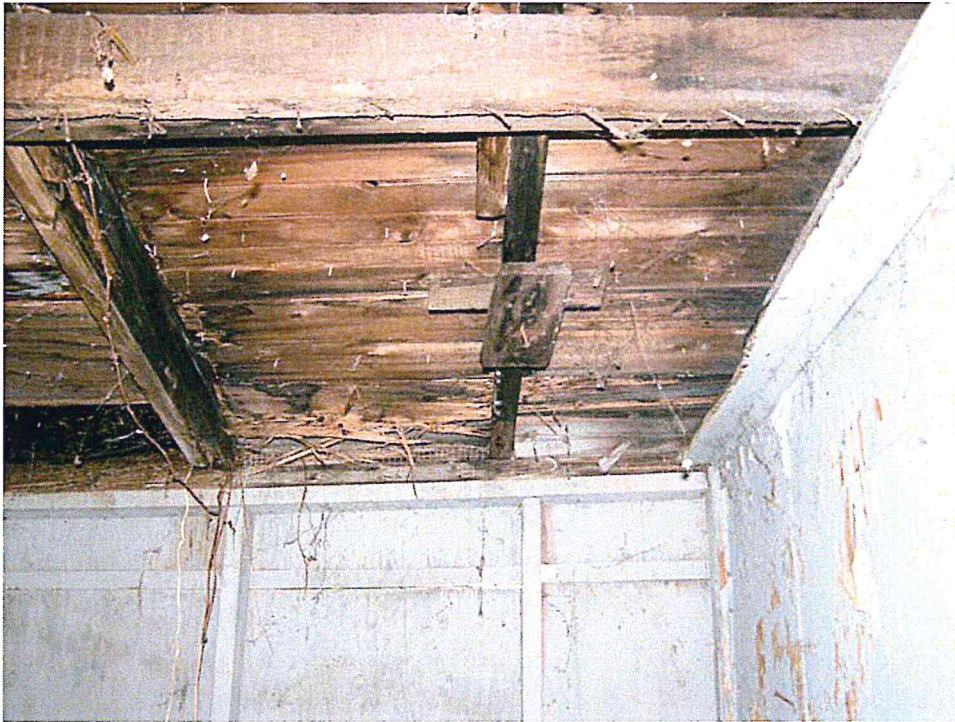
Photo 11 – Looking west at northwest corner. Roof sheathing is severely deteriorated.
