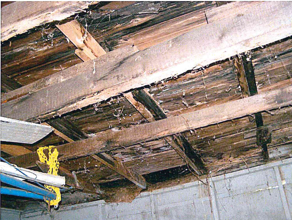
Photo 12 – Severely deteriorate roof sheathing and discontinuous roof rafters.
