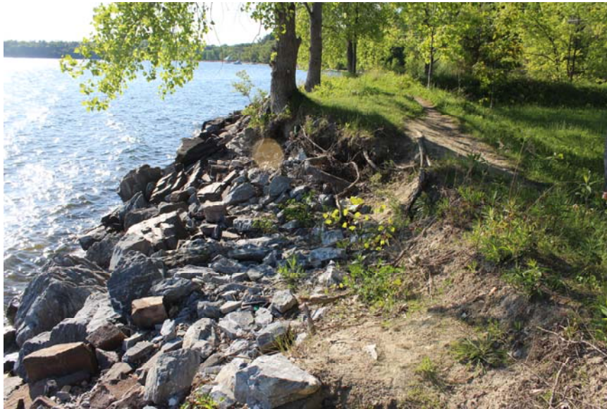
Photograph 1. Representative view of compromised stone revetment in Urban Reserve. Intact revetment visible in background (Date: 6/1/14)
