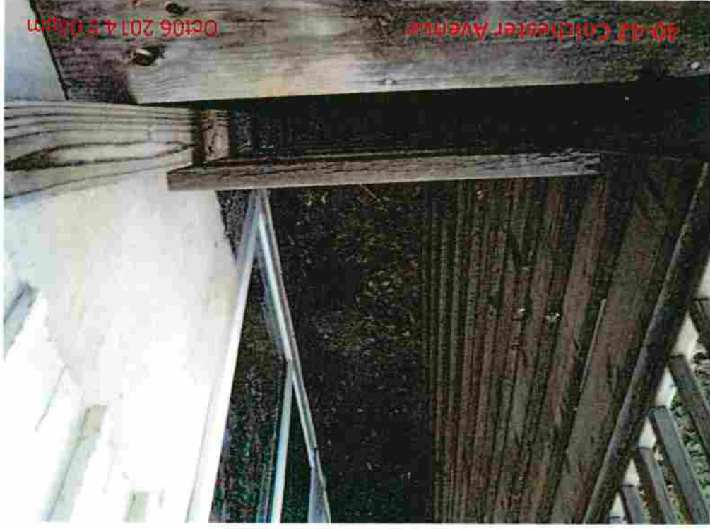
Conditions observed on 10-6-14 Photos taken by William Ward
