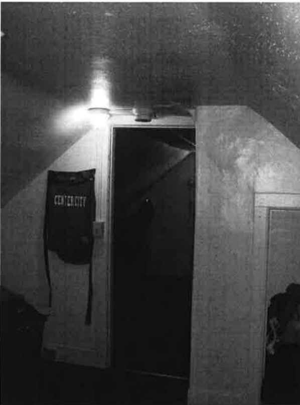
97. Second floor has worn features and finishes.
