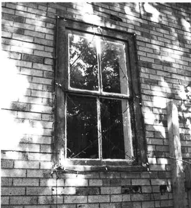
59. Typical window and trim on side elevations in very poor condition.
