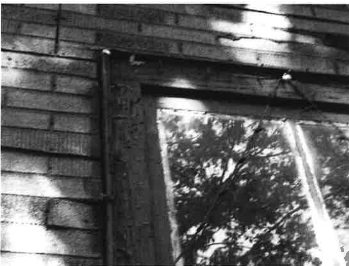
60. Detail of weathered trim and single pane window.
