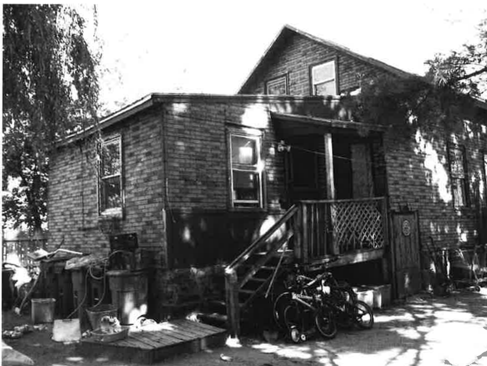
46. View looking northeast of the rear and south elevations. Structural concerns are evident in the shed roof of the rear ell which is sagging at the center of the west end roof eaves.
