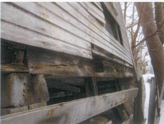
Photo #8 - West wall, rotted sill beam
