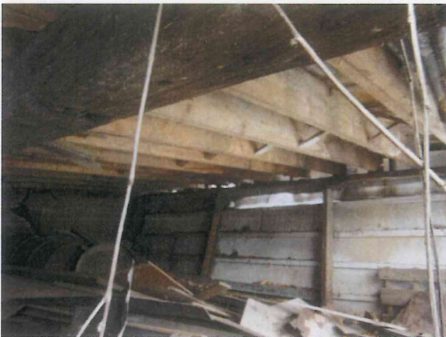
Photo #12 - South wall with failed vertical metal struts, metal sheeting and top horizontal channel
