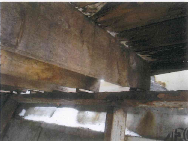
Photo #13 -South wall corroded top horizontal channel and displaced metal sheeting
