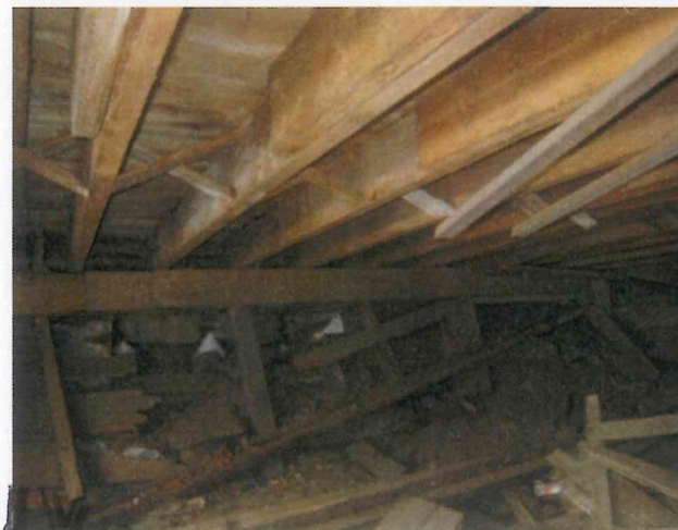
Photo #16 - North wall failed wood sheeting
