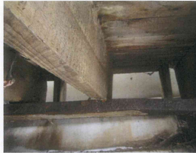
Photo #14 -South wall corroded top horizontal channel
