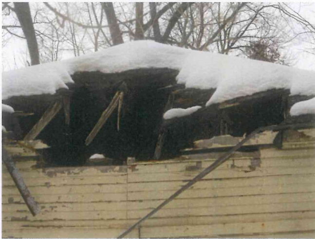
Photo #6 - Roof Damage, South Side
