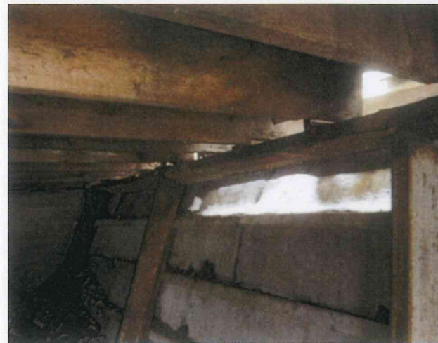
Photo #15 -South wall displaced metal sheeting and vertical struts leaning, probably sheared off at the base
