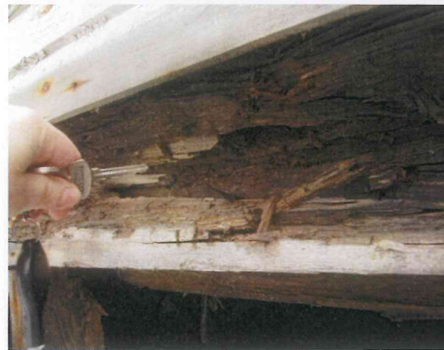
Photo #10 - West wall, rotted sill beam, breaks away with light pressure from key
