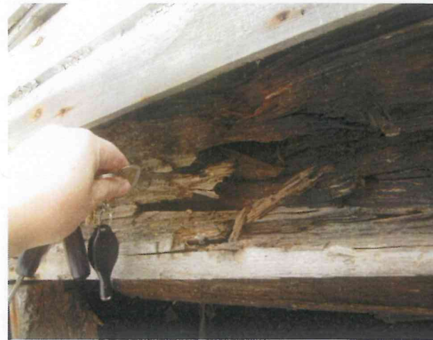
Photo #9 - West wall, rotted sill beam
