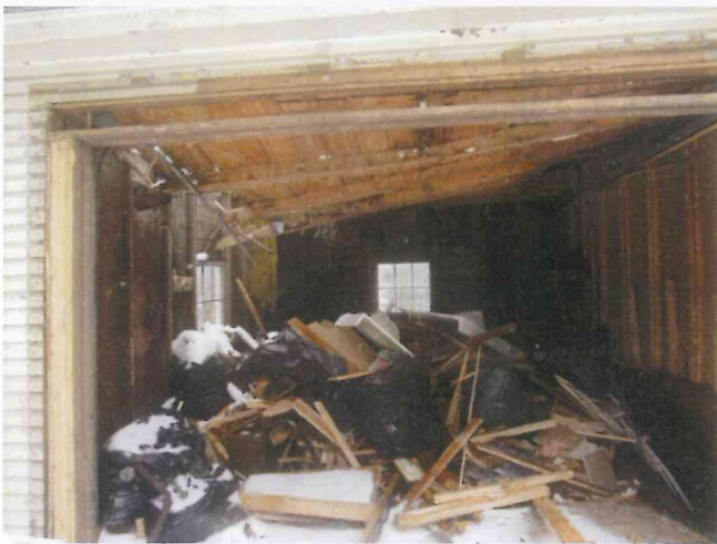
Photo #7 - Roof Damage, South Side
