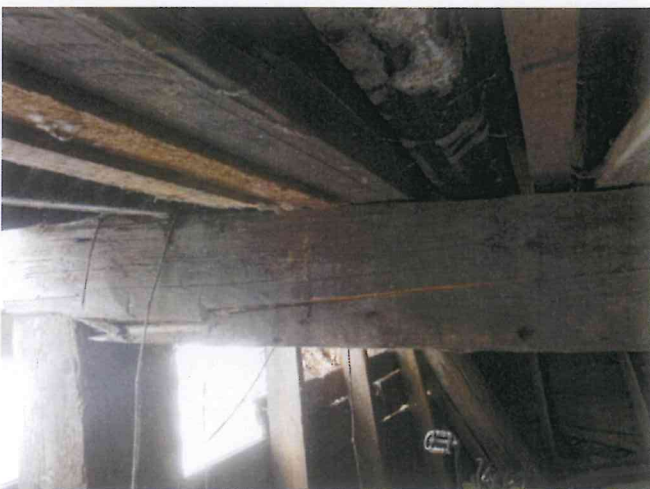
Photo #19 - failed center beam supporting floor joists
