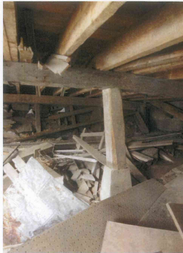
Photo #20 - leaning timber post under center beam
