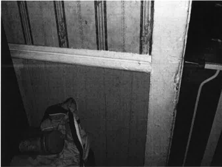
74. Typical view of the worn vertical board wainscoting and door trim.
