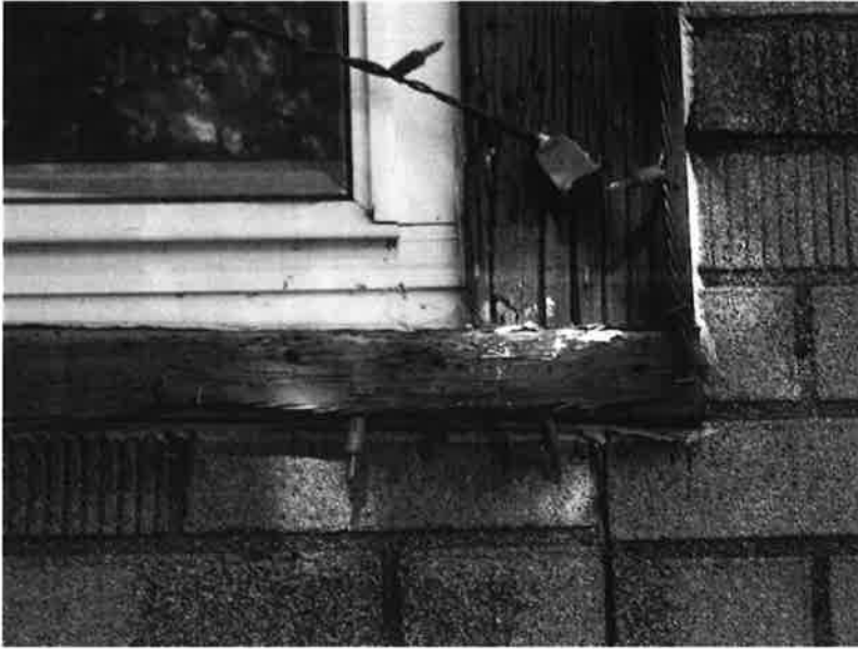
61. Additional view of typical vinyl window and storm, and deteriorated trim.
