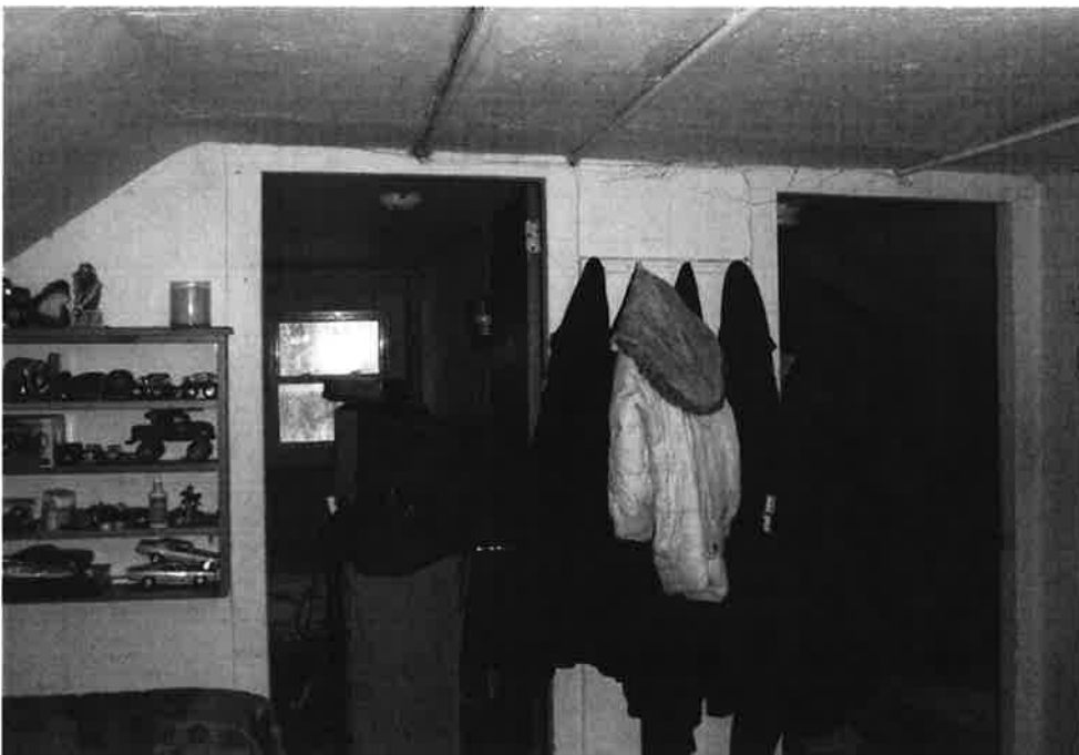
77. Second floor looking west from top of stairs. Note worn features and finishes.
