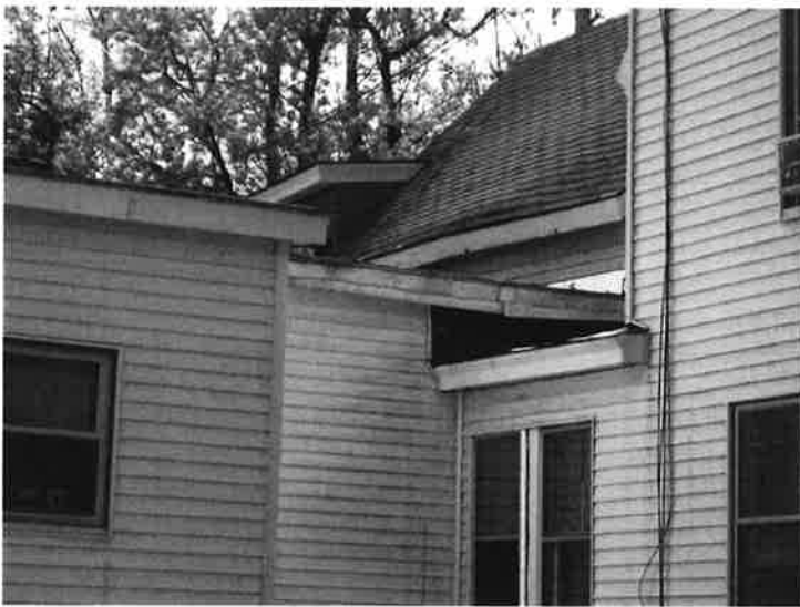
12. Detail of east elevation; note bowed roof at eaves and variety of adjacent roof slopes.
