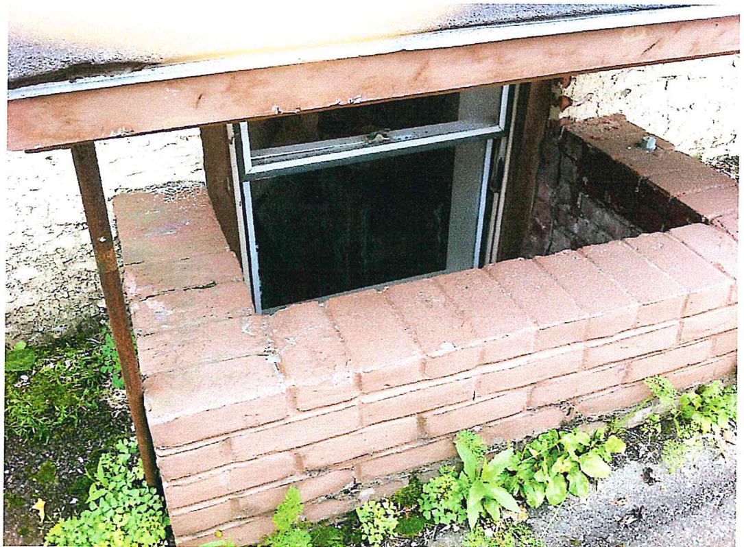
Photo 8. The first floor windows are now mostly buried. The north windows have these little window wells put in to offer some protection from snow and rain. Rooms inside are dark and gloomy. The Cellar is a full floor below the floor these windows are on.
