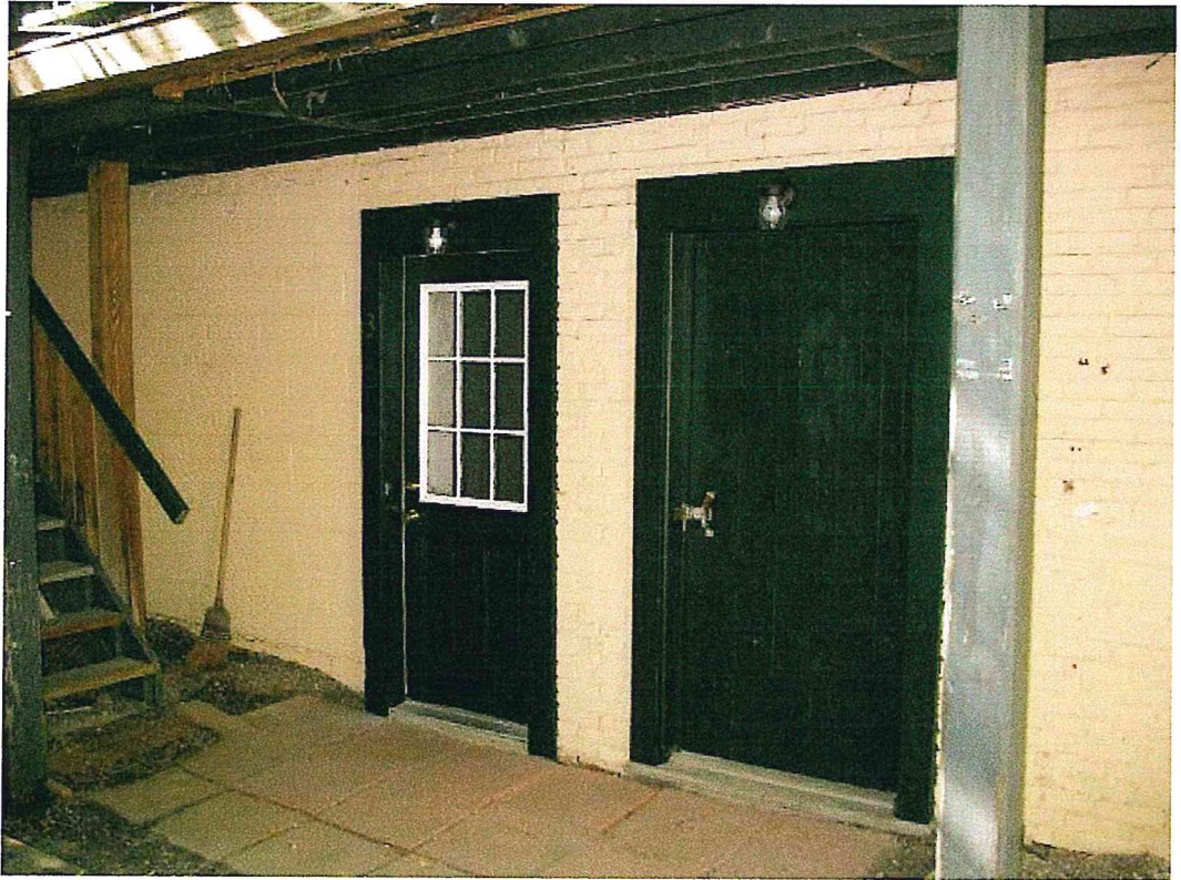
Photo 11. On the south side, the wall east of the first floor apartment past the door with the light in it, was rebuilt in concrete block. We assume that the brick veneer failed at some point and was replaced with concrete block. The renovations will replace this concrete block with brick veneer to match the original brick veneer conditions.
