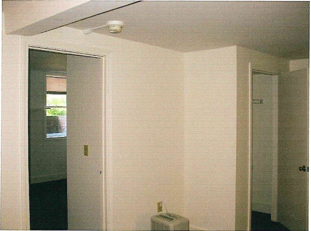
Photo 27. First Floor, west end apartment (#3). Note the mostly buried window visible through one of the two bedrooms in the apartment. One of the historic 8x8 beams (now covered in Sheetrock) is visible in the upper right hand corner.
