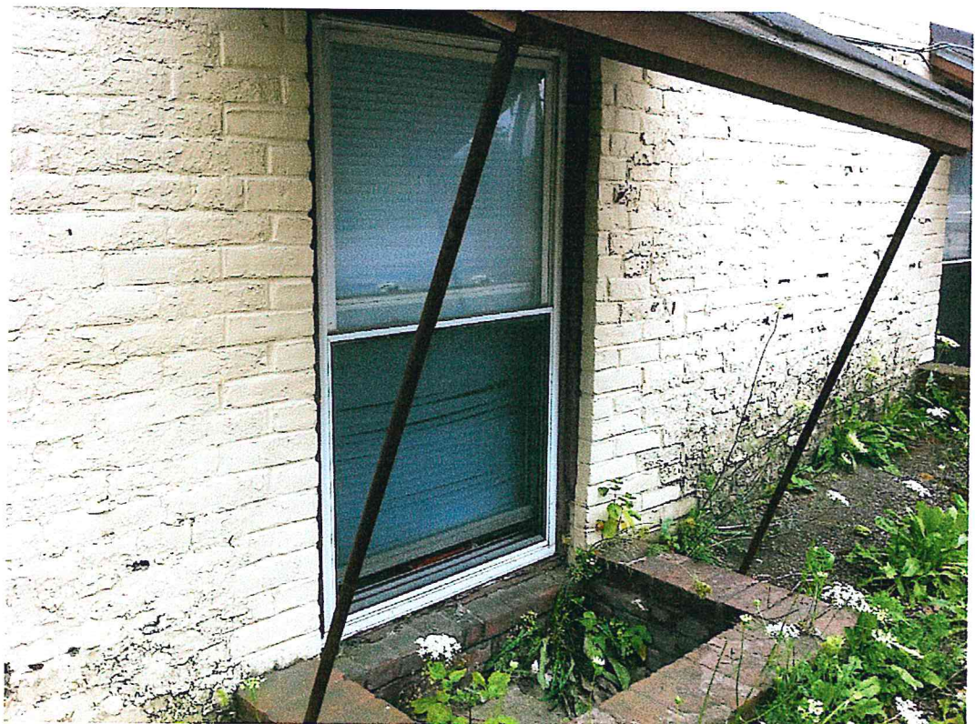
Photo 18. North side windows are buried to various depths. They have more exposure the closer they are to the east side of the building. None of the windows are the original 2-over-2 pattern seen in historic PHOTO 3.
