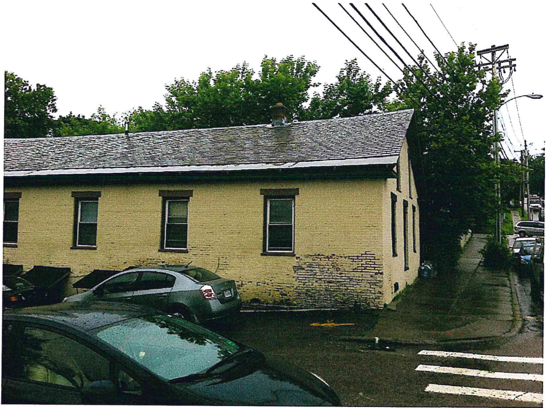
Photo 5. North elevation photo taken 2014. Note evidence of rising damp on the bricks at the west end of the north elevation, caused by the building being buried.
