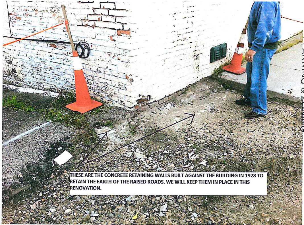
Photo 35. Retaining walls built in 1928 to retain the earth of the raised roads. Wall is poured directly against the brick veneer of the building, and is causing damaging rising damp to the façade. Note that original color of building was unpainted dark red/maroon colored bricks.
