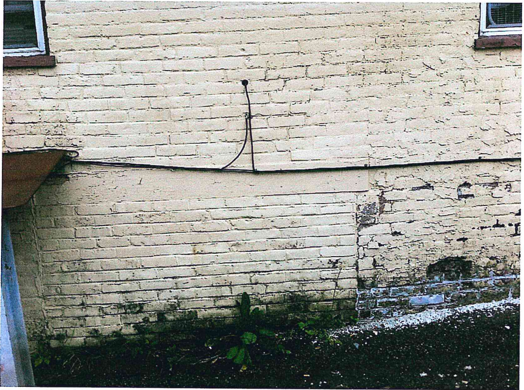
Photo 17. Evidence of where loading dock doors were filled in with brick on the north elevation. The painted wood lintel remains. Note damage from rising damp to the right of the blocked opening. The black lines are cable TV cables.
