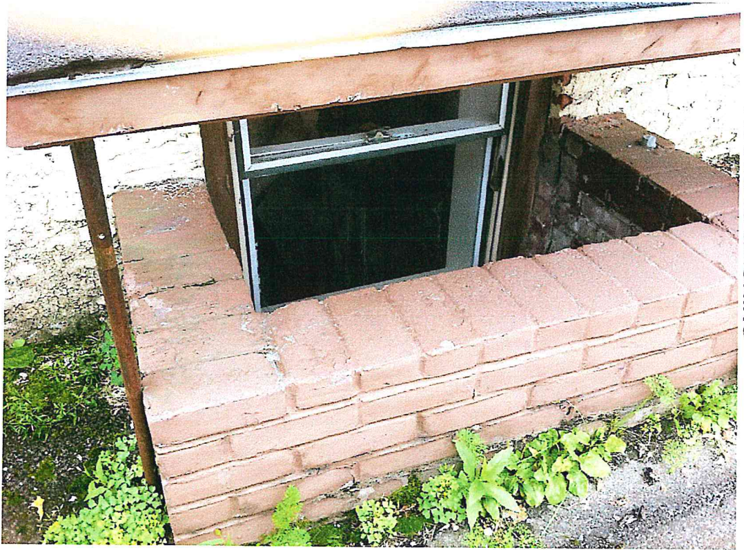
Photo 19. North side first floor windows on the west are buried more than those toward the east due to the slope of the street in front of the windows. The brick window wells were built when the building was buried in 1928.
