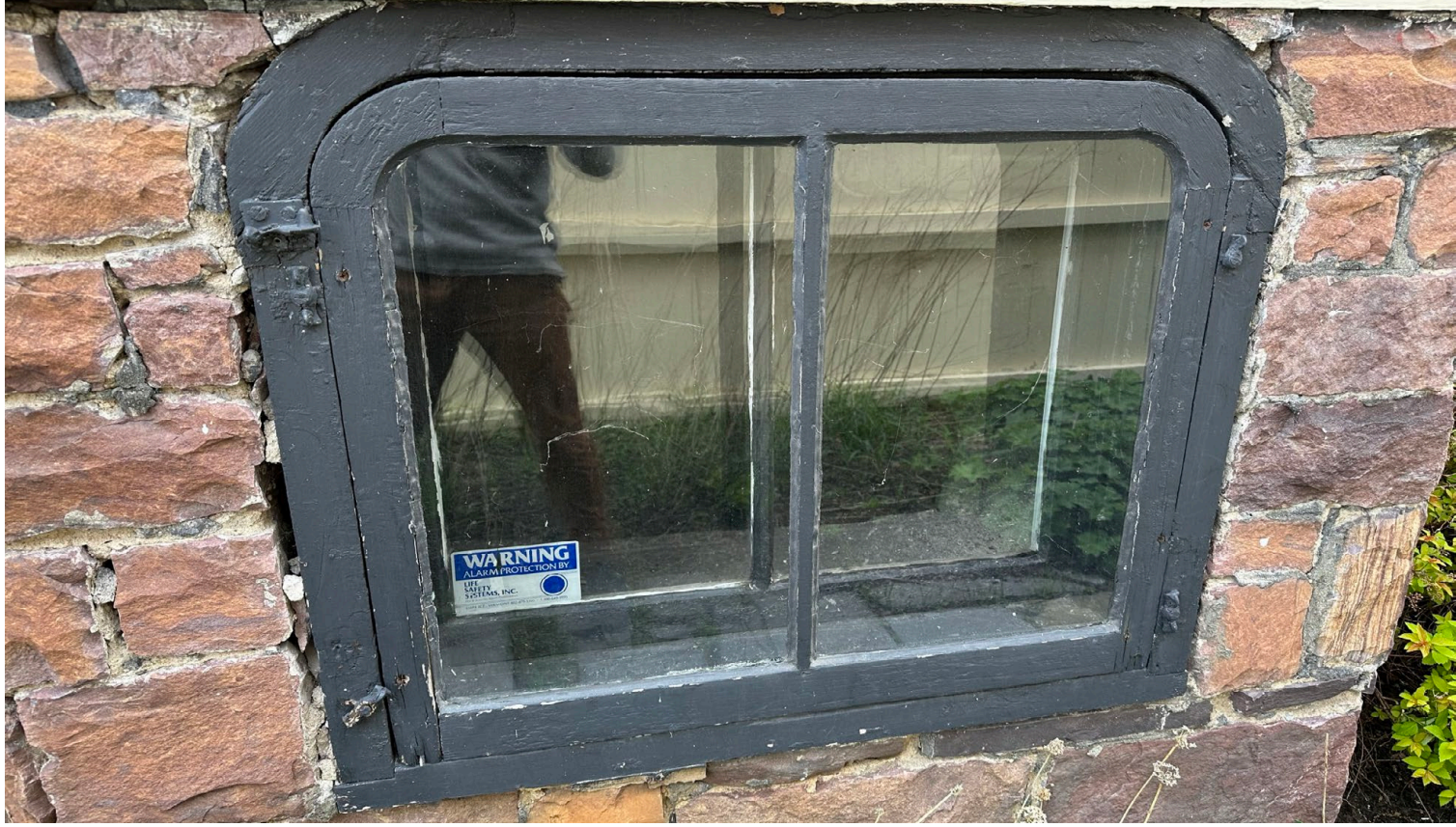
SEALANT FAILURE, FOUNDATION RE-POINTING NEEDED
