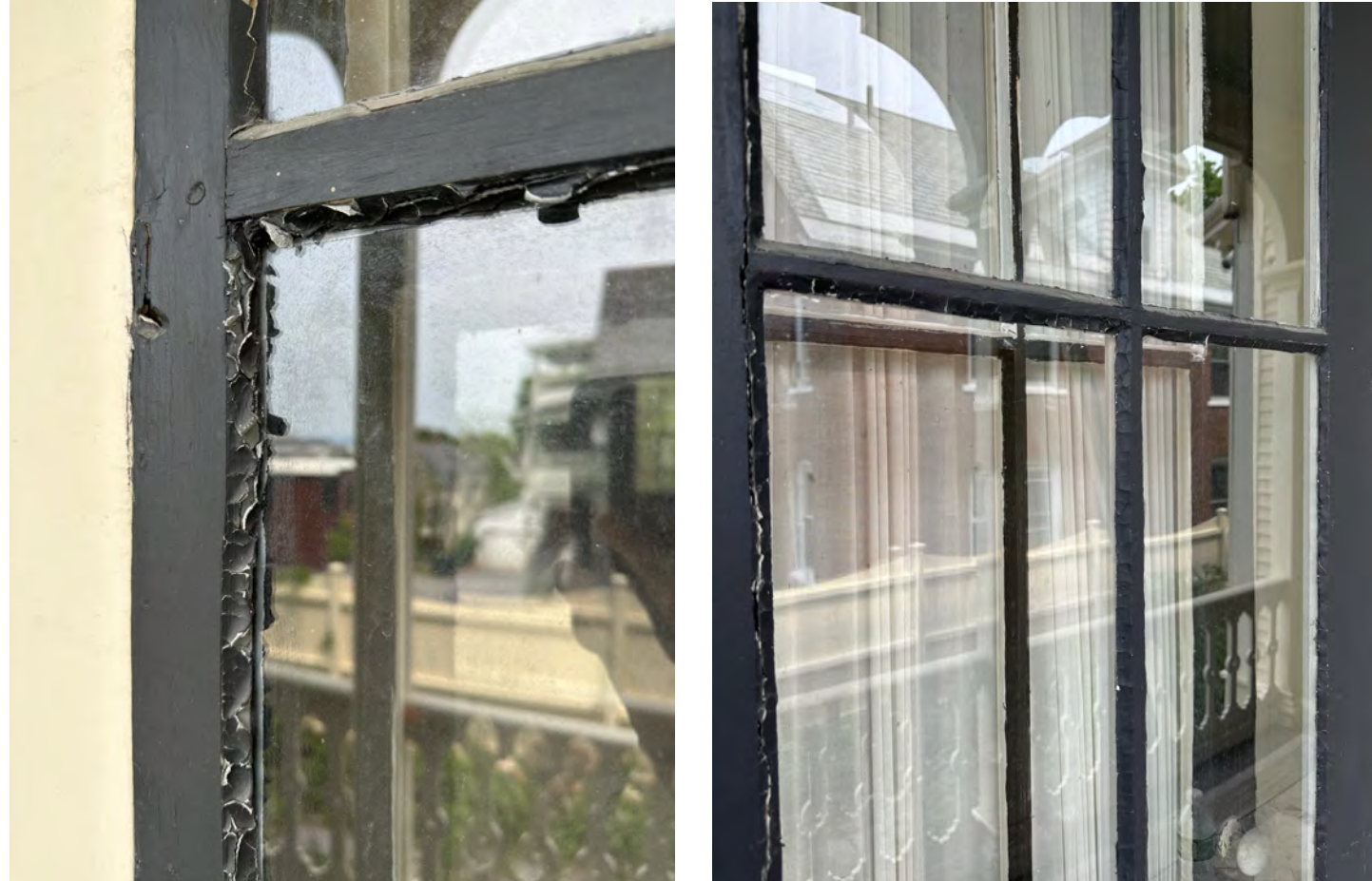
MAIN HOUSE - TYPICAL CONDITIONS OF ORIGINAL WINDOWS
