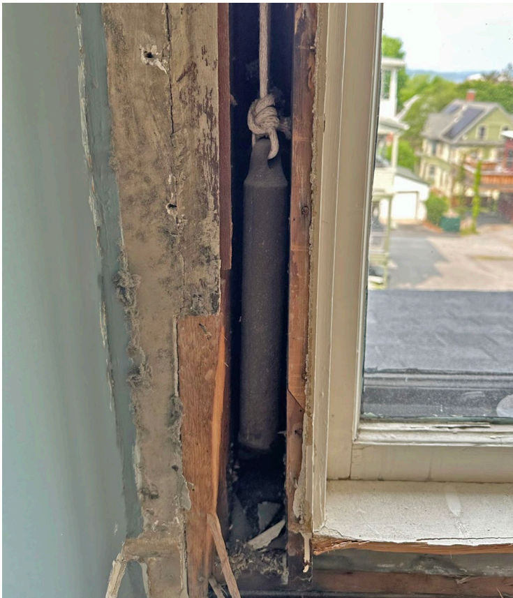
UNINSULATED COUNTERWEIGHT CAVITY
