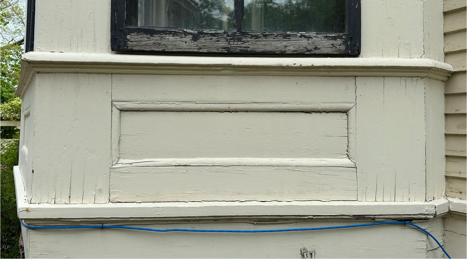
TRIM REPLACEMENT & REPAINTING NEEDED
