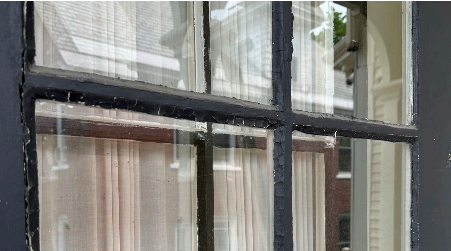
SEALANT FAILURE, SINGLE PANE
