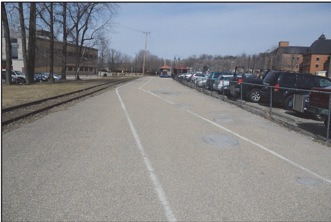
Photo 6. Minimal Bike Path delineation (fading paint) between the high traffic area of King Street and College Street. View is to north.
