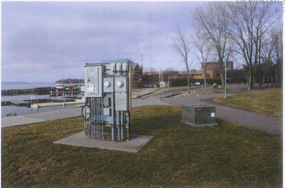
Photograph 5: View of backboard and electrical panels, west side of Event Grounds at intersection of Bike Path and sidewalk (VHB, 12/4/13)
