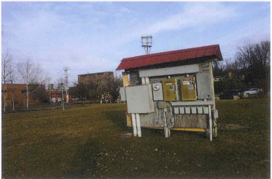
Photograph 6: View of backboard and electrical panels, north end of Event Grounds (VHB, 12/4/13)
