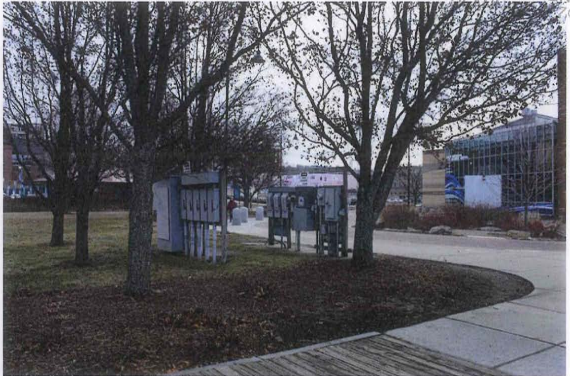
Photograph 1: View of backboards and electrical panels, College St. (VHB, 12/4/13)
