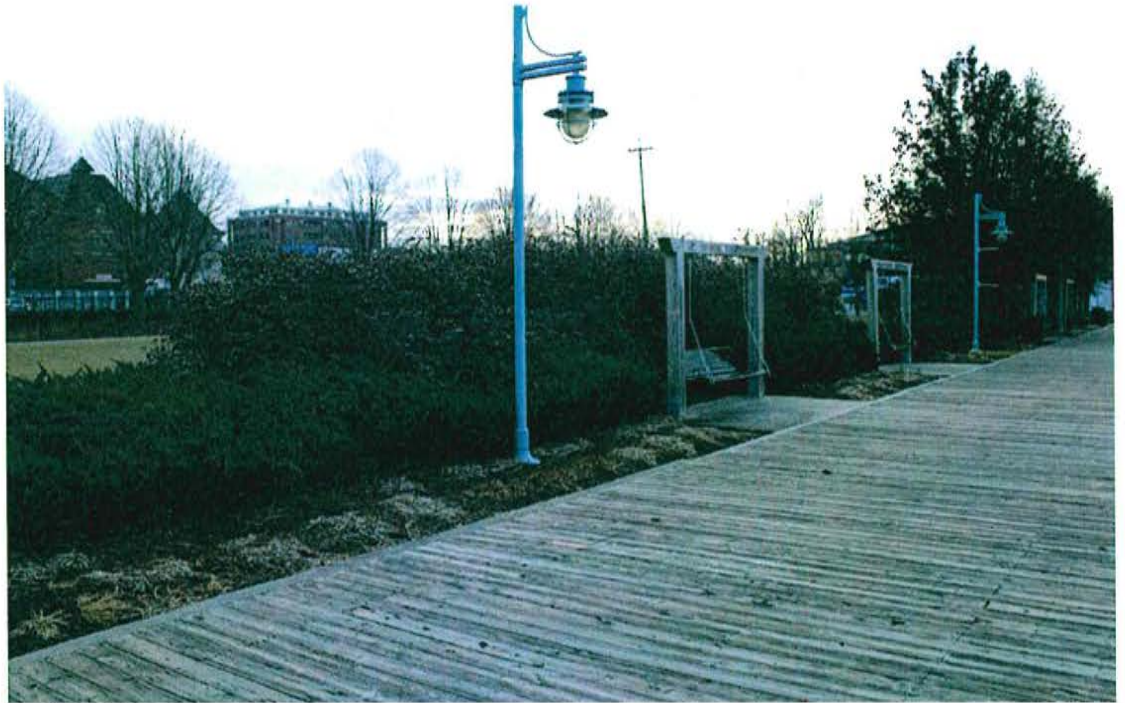
Photograph 7: View boardwalk planks to be replaced, light fixture to be replaced (VHB, 12/4/13)
