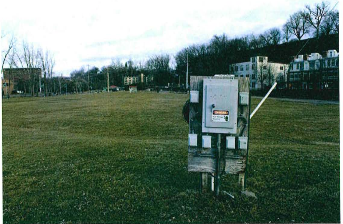
Photograph 3: View of backboard and electrical panels, south center of Event Grounds. (VHB, 12/4/13) (VHB, 12/4/13)
