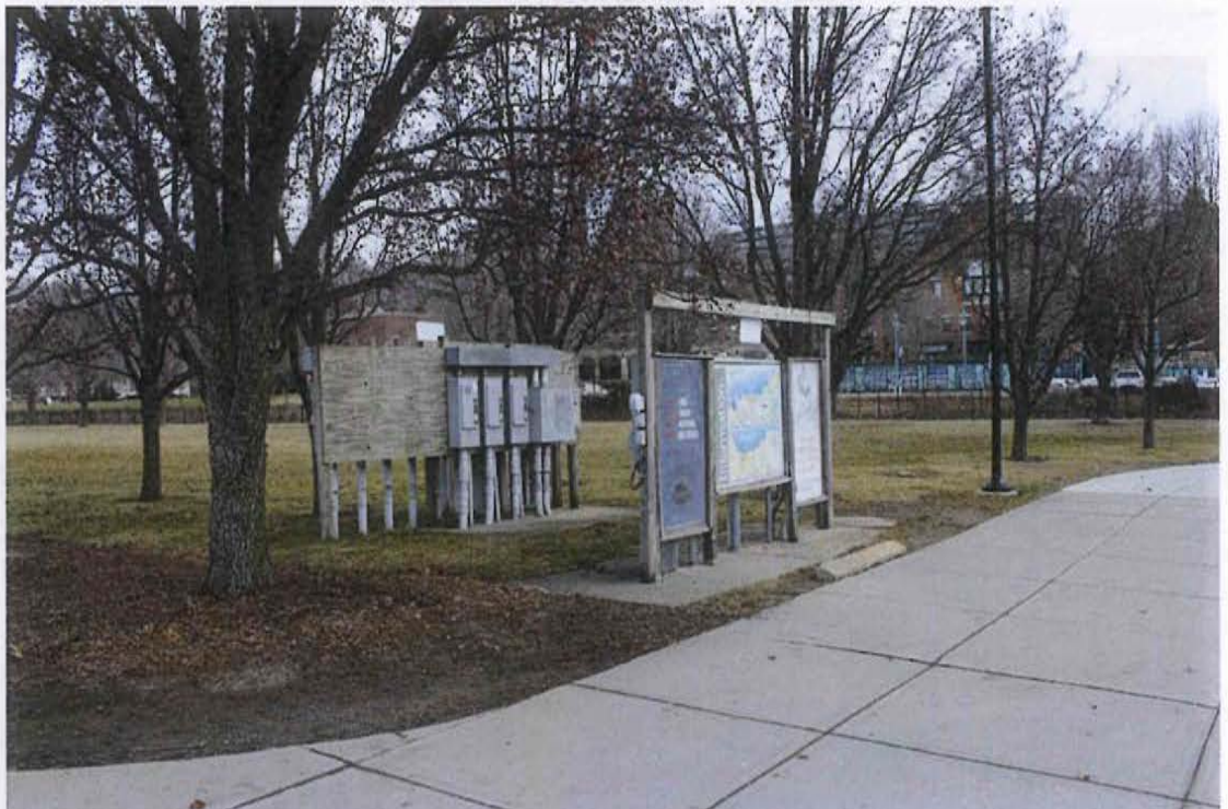
Photograph 2: View of backboards and electrical panels, College St. (VHB, 12/4/13)
