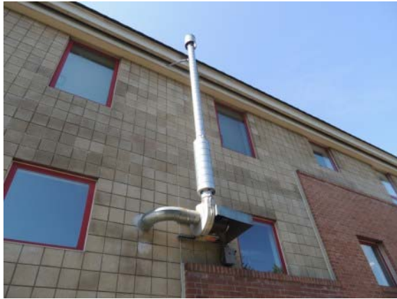
Photo #13: Vehicle engine exhaust system at west elevation
