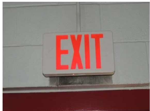
Photo #36: Typical exit sign
