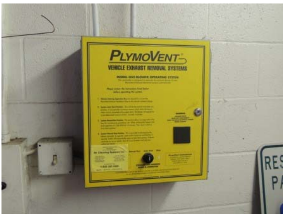
Photo #53: Vehicle exhaust system located in the garage equipment bay
