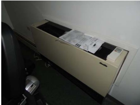
Photo #19: Fan cabinet unit located in the first floor workout room
