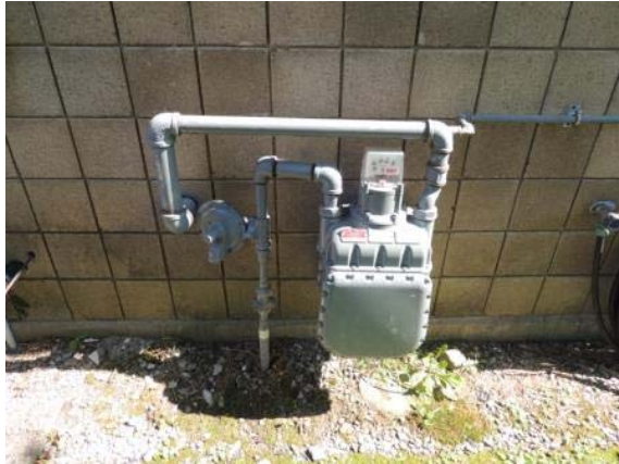
Photo #1: Natural gas meter at west elevation
