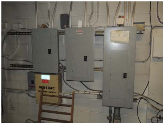
Photo #39: Incoming electrical service located in the first floor mechanical room
