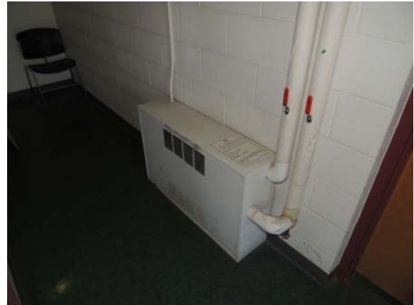
Photo #20: Radiator located in first floor hallway
