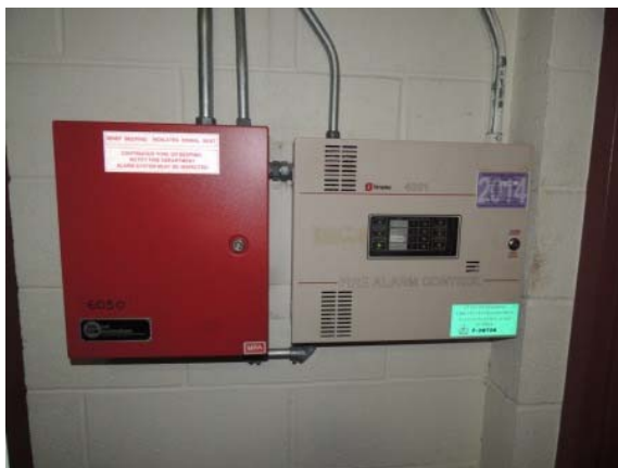
Photo #41: Fire alarm panel
