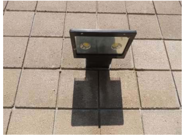
Photo #32: Exterior light at rear south entrance
