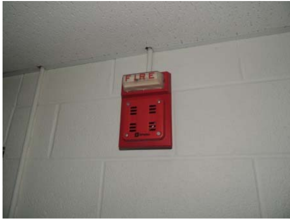
Photo #43: Typical fire alarm with strobe
