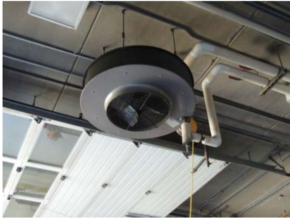
Photo #7: Hot water unit heater located in the garage equipment bay
