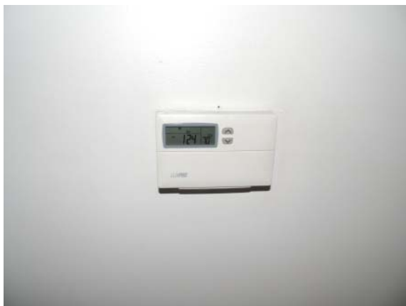
Photo #11: Thermostat located in the second floor living quarters
