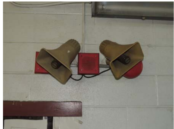
Photo #46: Fire alarm located in the garage equipment bay
