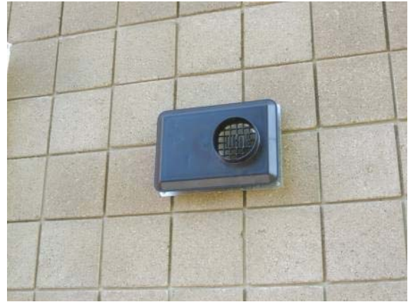
Photo #14: Boiler exhaust located west elevation
