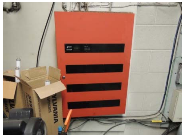
Photo #42: Fire alarm panel
