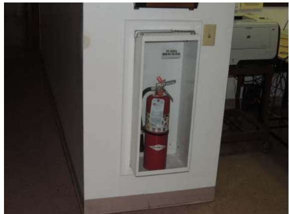
Photo #52: Typical fire extinguisher
