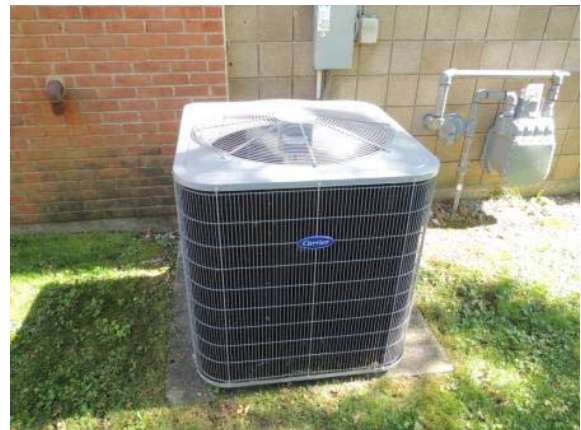
Photo #4: Air cooled condensing unit located at the west elevation
