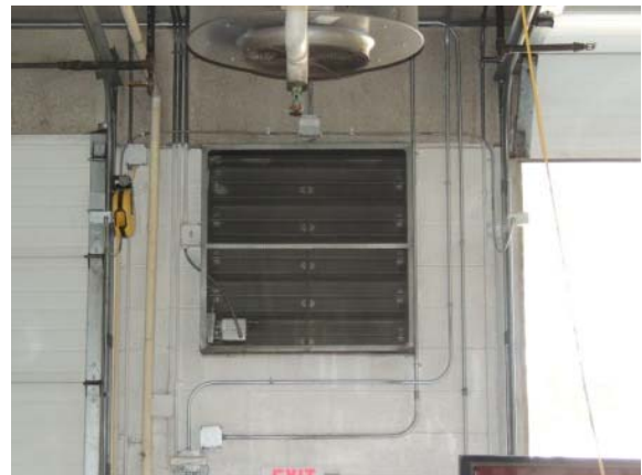
Photo #10: Exhaust ventilation louver located in the garage equipment bay
