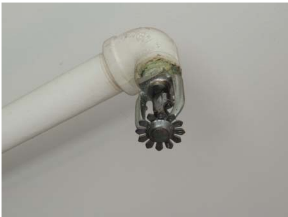
Photo #51: Typical sprinkler
