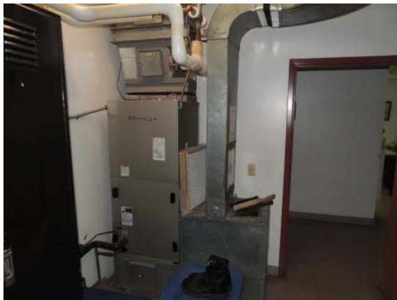
Photo #3: Vertical second floor fan coil unit with hot water heating coil located in the second floor mechanical room
