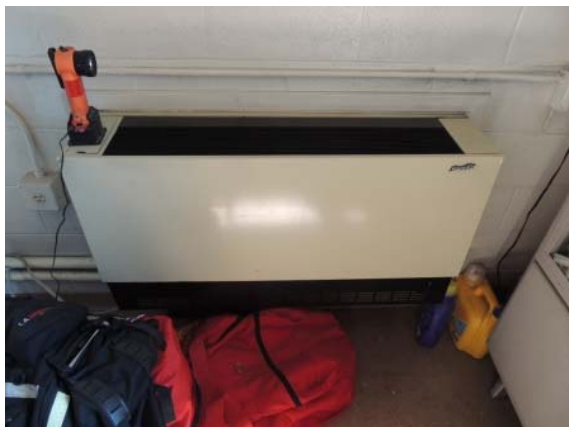
Photo #5: Fan coil unit located in the first floor office area
