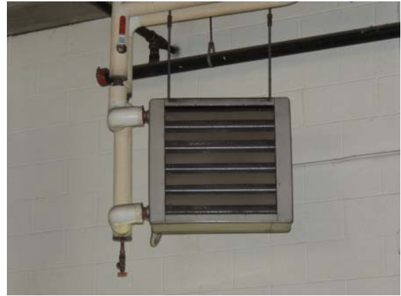
Photo #8: Hot water unit heater located in the garage equipment bay
