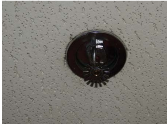
Photo #50: Typical sprinkler
