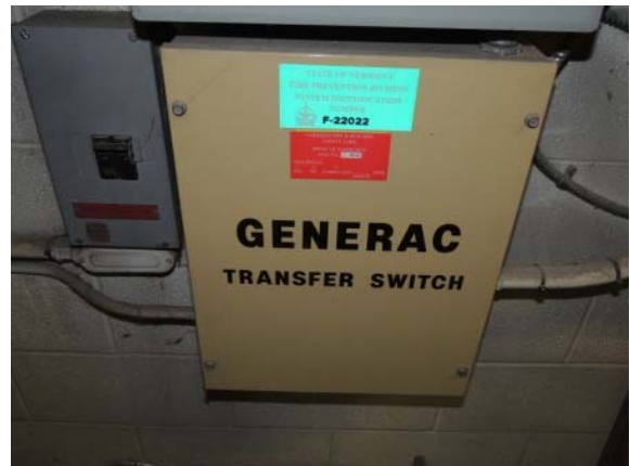
Photo #40: Generator transfer switch
