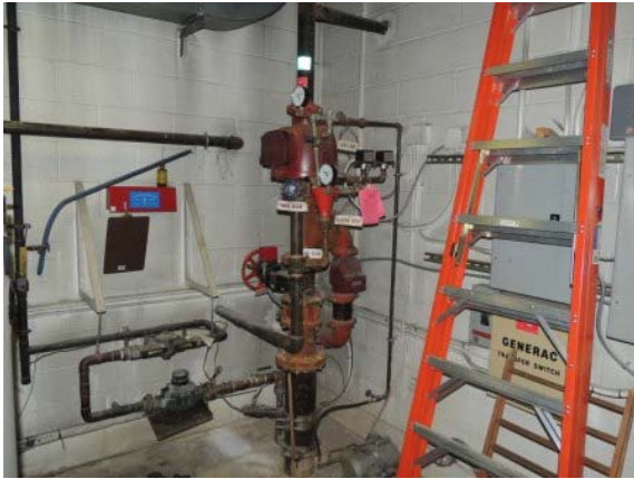
Photo #49: Incoming water and sprinkler service located in the first floor mechanical room
