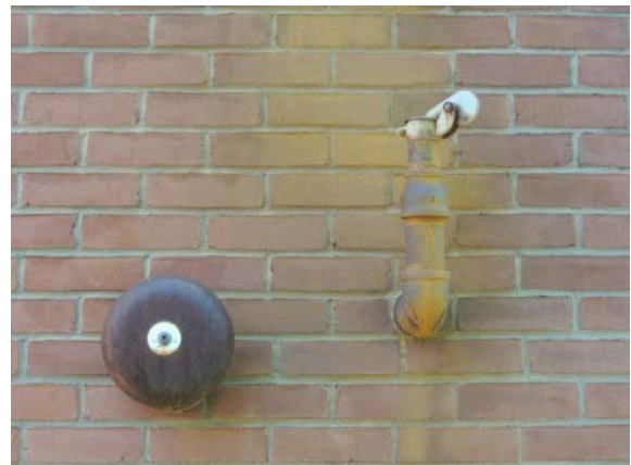
Photo #16: Sprinkler alarm and generator exhaust at west elevation
