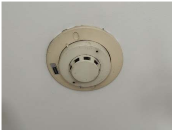
Photo #45: Typical fire alarm sensor
