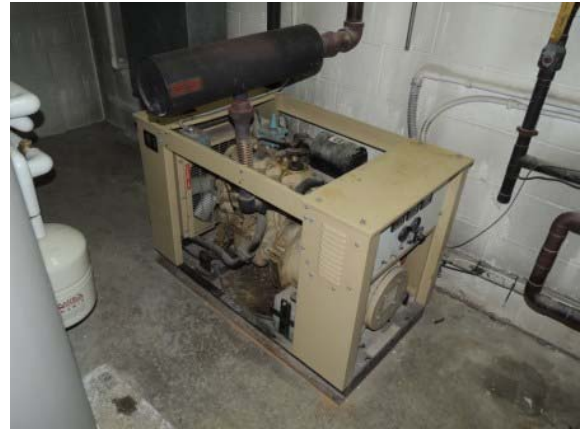
Photo #38: Emergency backup generator located in the first floor mechanical room
