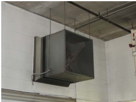
Photo #9: Exhaust ventilation fan located in the garage equipment bay
