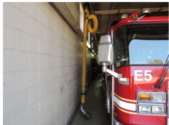
Photo #12: Vehicle engine exhaust system located in the garage equipment bay
