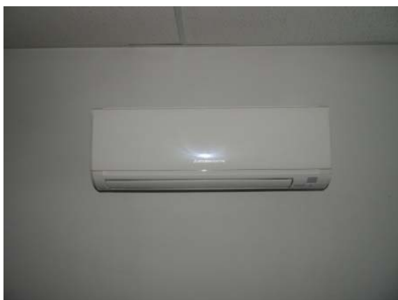
Photo #17: Ductless mini split air conditioner located in the first floor workout room
