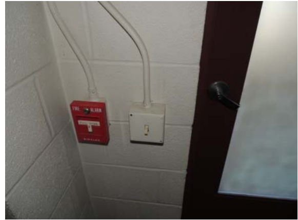
Photo #44: Typical pull station
