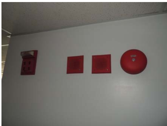
Photo #47: Fire alarm located in the second floor living quarters
