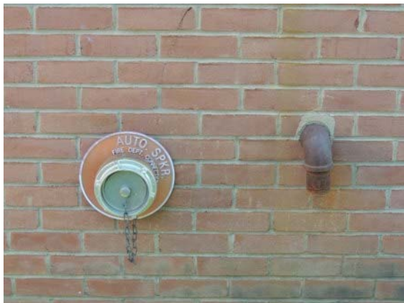
Photo #15: Fire department sprinkler connection at west elevation
