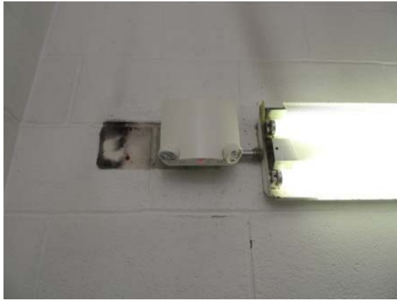
Photo #37: Typical emergency lighting
