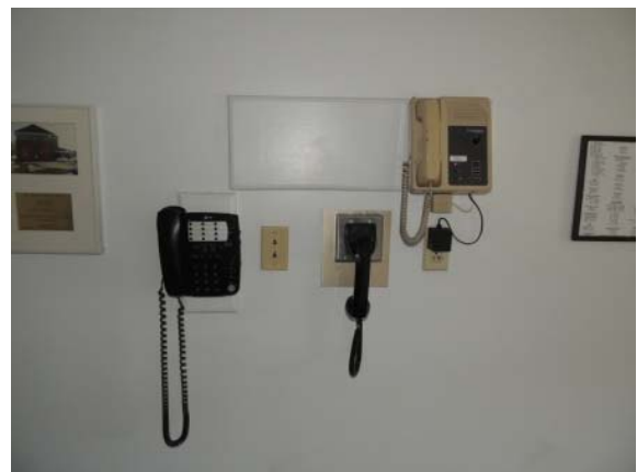
Photo #48: Communications area located in the second floor living quarters
