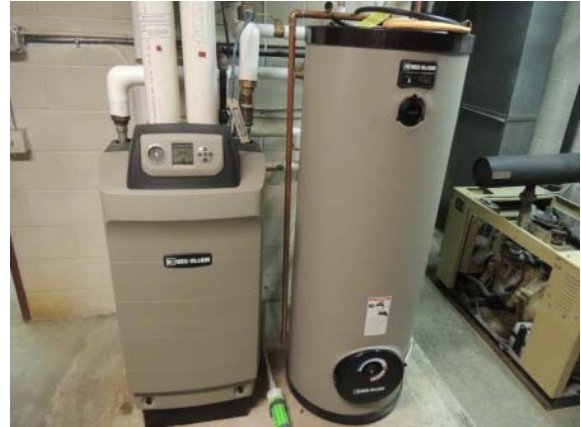
Photo #2: Hot water gas boiler and domestic hot water tank located in the first floor mechanical room
