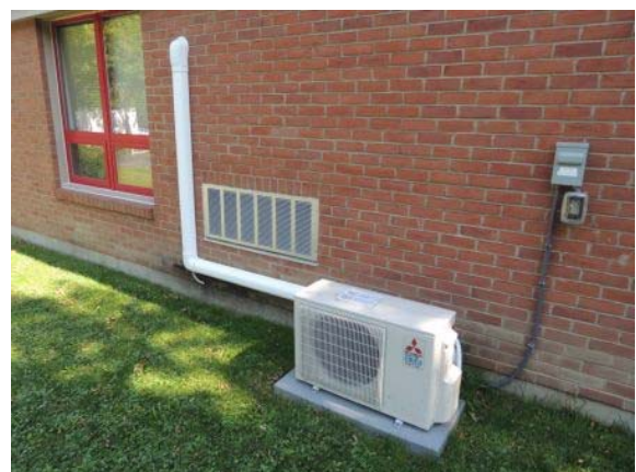
Photo #18: Ductless mini split air cooled condensing unit at west elevation
