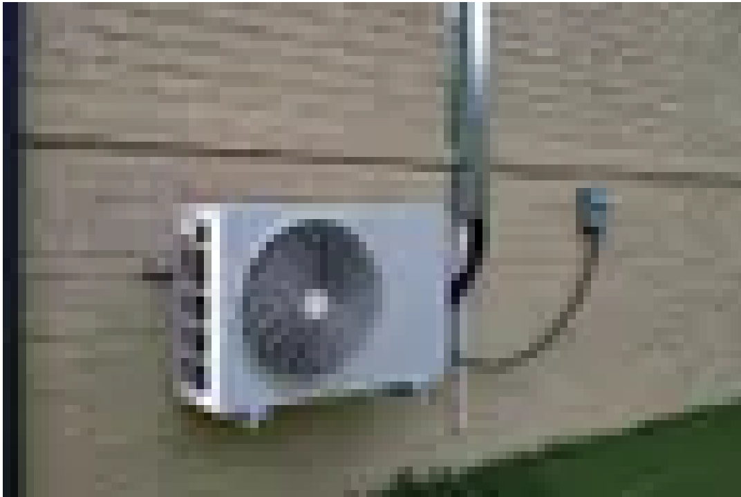
Heat pump mini split system next to home with painted brick wall and space for text copy GETTY
