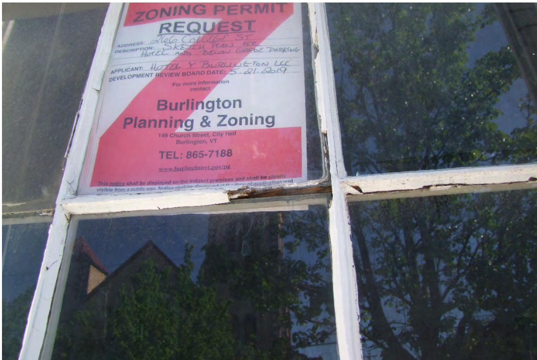
Photograph 31: Example of deteriorated historic wooden window on the south elevation.
