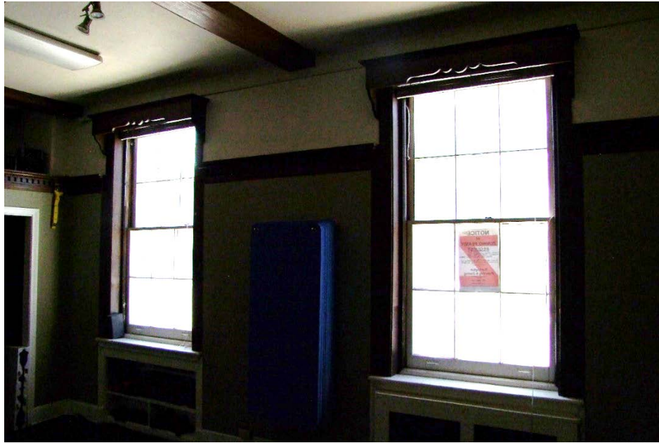
Photograph 27: Interior view of representative wooden sash windows on the first floor of the south elevation. The historic wooden, sash windows are in fair condition throughout and are proposed to be replaced.
