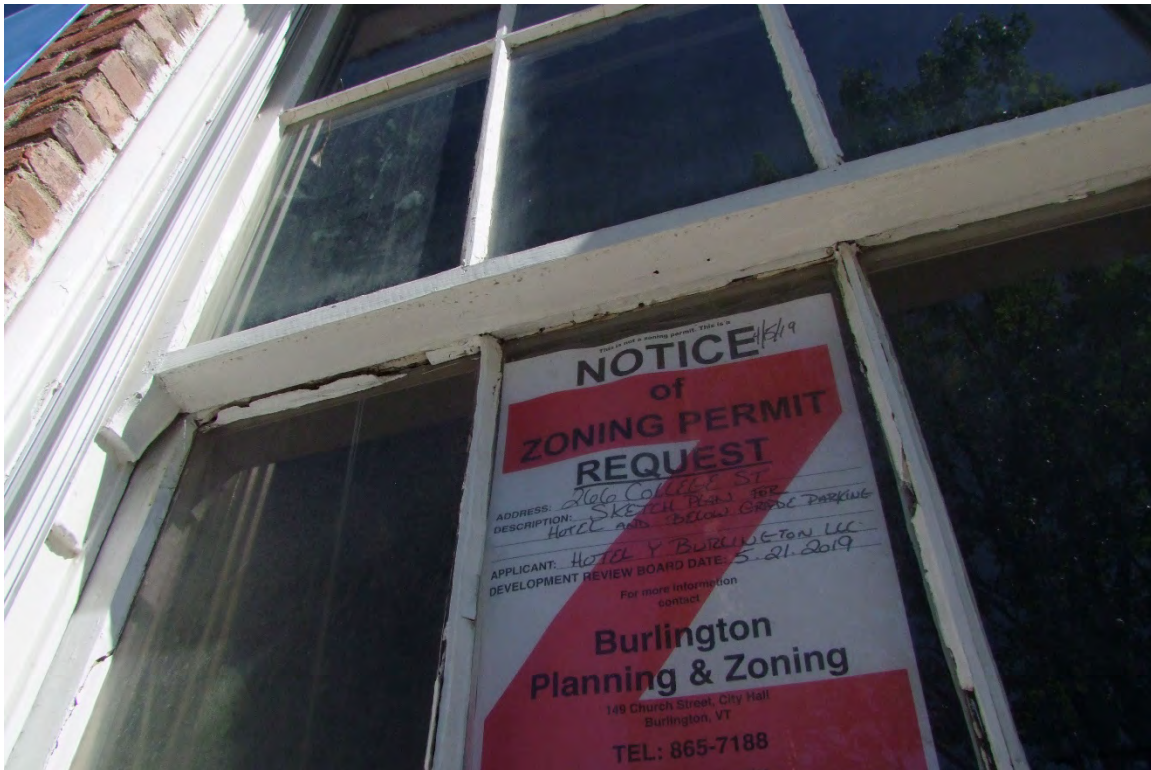
Photograph 30: Example of deteriorated historic wooden window on the south elevation.
