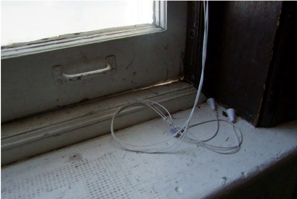
Photograph 29: Example of deteriorated historic window at the south elevation interior.
