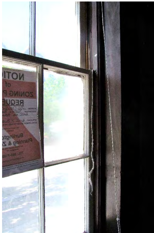
Photograph 28: Example of broken sash cord on an historic wooden window on south elevation. Many of the historic windows have deteriorated or broken sash cords.
