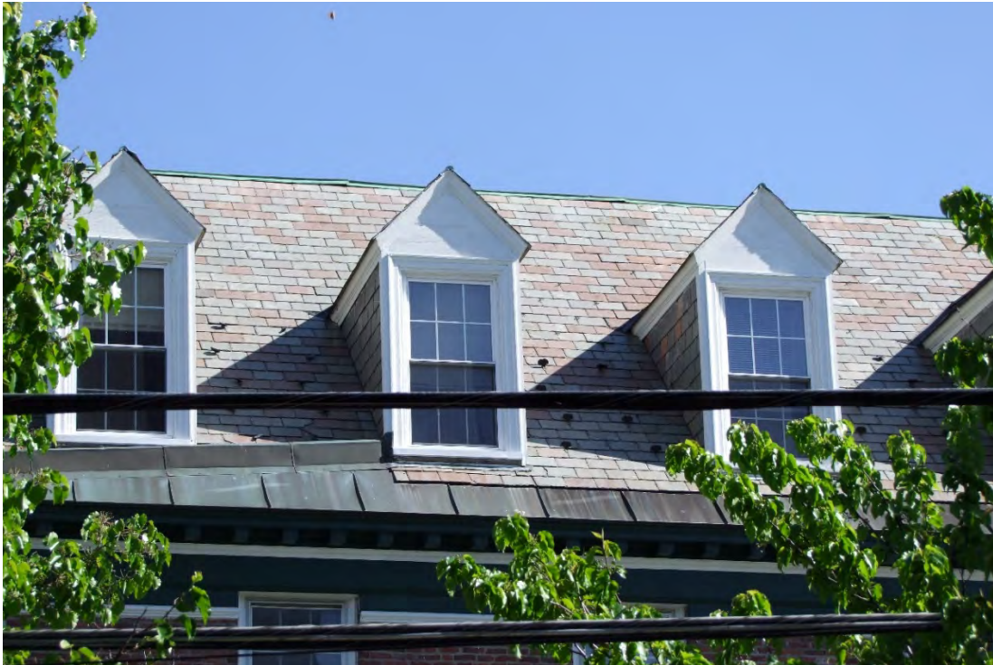
Photograph 3: Vinyl replacement windows visible on fourth floor of the south elevation. The slate roof will be repaired as needed following the Secretary of the Interior's Standards for the Treatment of Historic Properties
