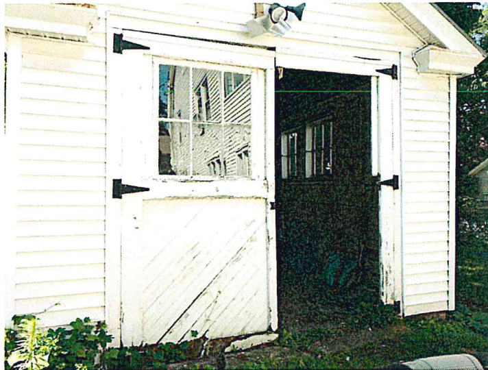
Figure 3: Half of current garage door is missing, other half is a safety hazard.
