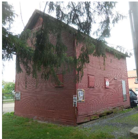
PHOTO 2: North-East Corner - Note deteriorated siding along bottom of structure
