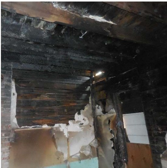
PHOTO 7: South-East Corner - Note charred framing at bottom of 2 nd Floor framing
