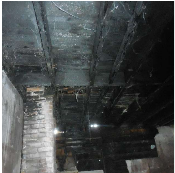
PHOTO 6: South-East Corner - Note charred framing at bottom of 2 nd Floor framing
