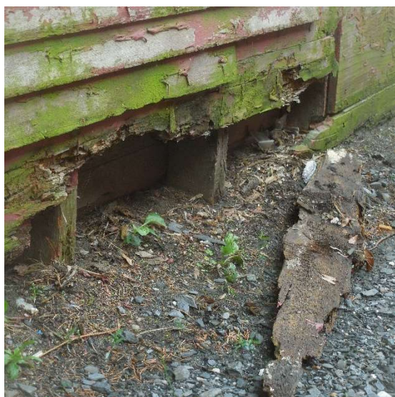
PHOTO 3: North Side – Top of stone foundation. Note wood decay at base of building
