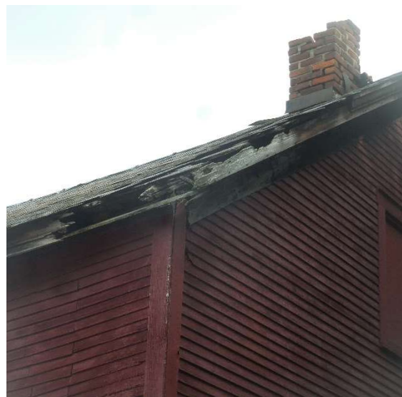
PHOTO 8: South-East Corner - Note loose & missing brick at top of chimney
