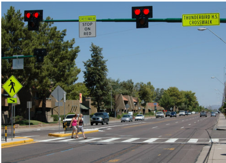
Typical installation of Pedestrian Hybrid Beacon
