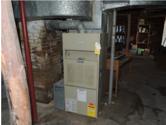
Photo #79: Residential gas-fired furnace located in the House/Office basement
