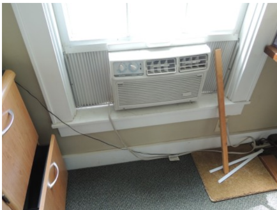
Photo #81: Window air conditioner
