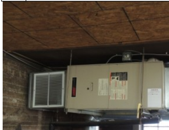
Photo #96: Maintenance Building furnace
