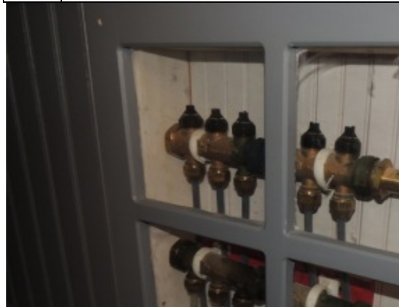
Photo #94: Heating system hot water manifold
