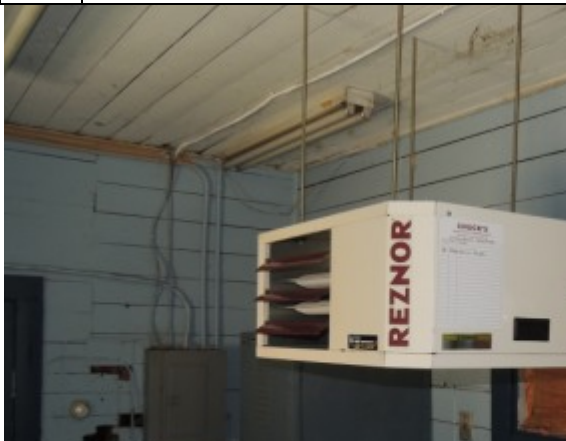
Photo #95: House/Break Room unit heater
