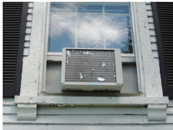
Photo #82: Window air conditioner
