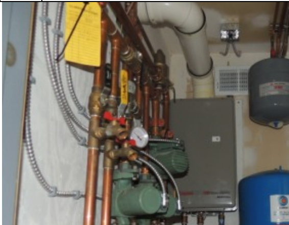
Photo #93: Chapel hot water central heating system
