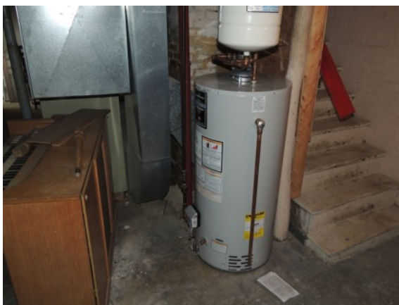
Photo #83: Domestic gas fired water heater
