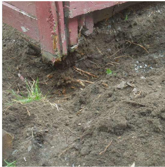
PHOTO 4: North-East Corner – Note wood decay at base of building
