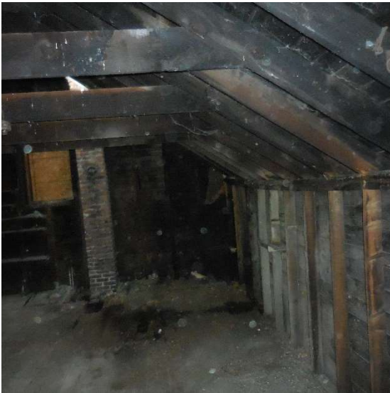
PHOTO 5: South-East Corner (2 nd Floor) - Note hole in floor near chimney
