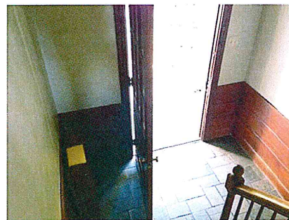
Front door, obstructing the landing and use of the stairs
