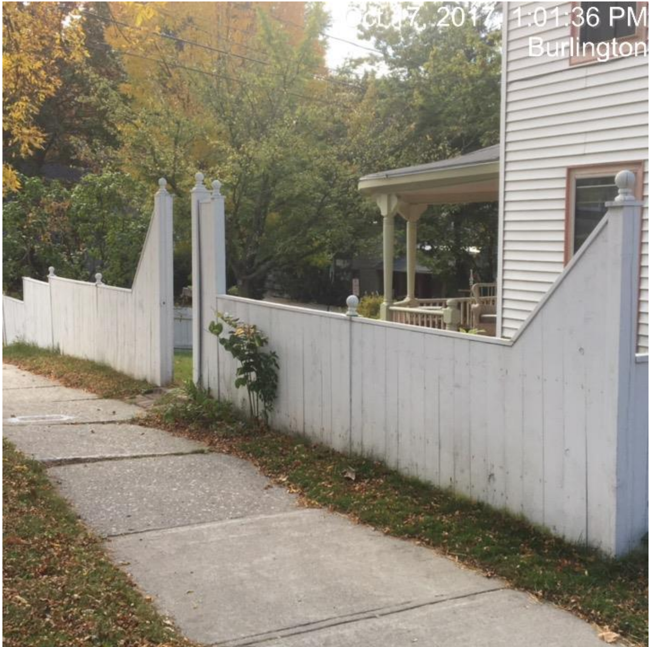
Fence does not comply with its approved style and height.
