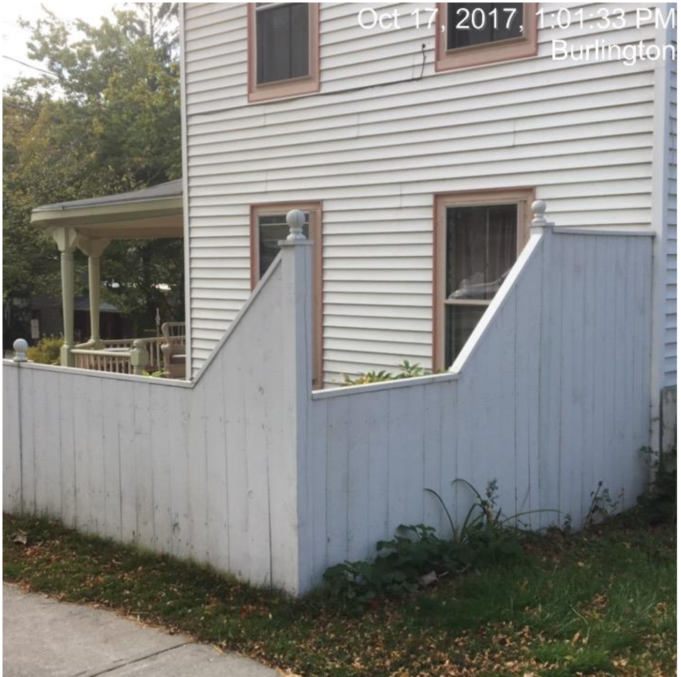
Fence does not comply with ZP 99-430
