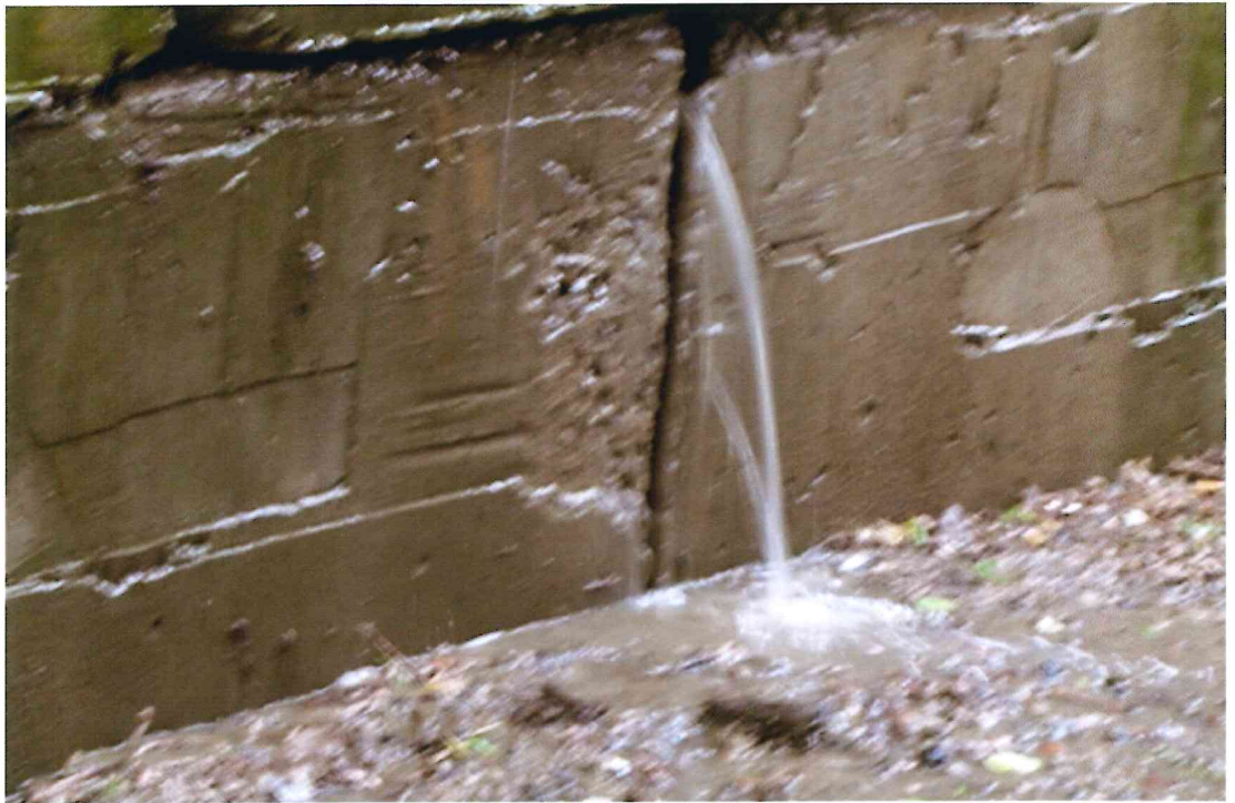
various photos of water flow from wall during rain storm...water flow onto property and into catch basin...resulting silt and winter seepage from ...
