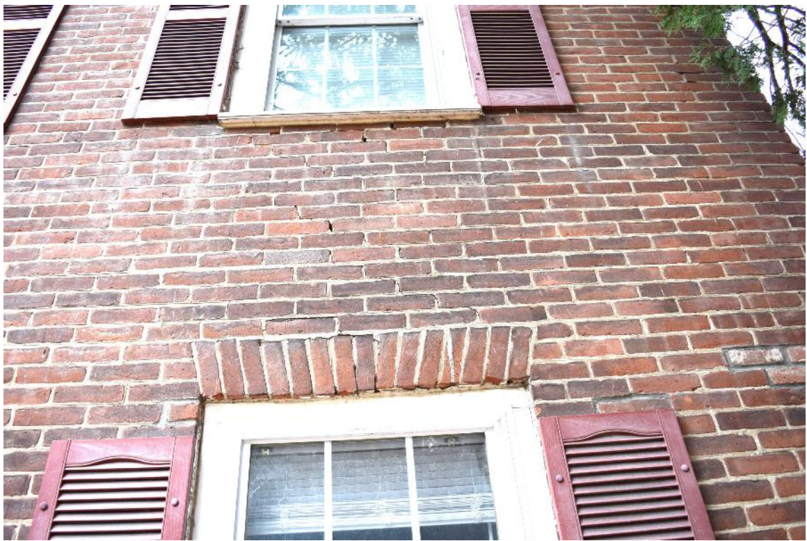
Figure 28: View shows example of widespread structural problems with the brickwork
