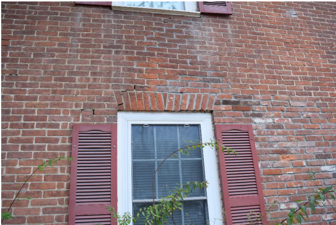
Figure 27: View shows example of widespread structural problems with the brickwork
