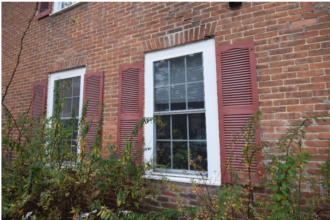
Figure 31: View shows example of widespread structural problems with the brickwork, and vinyl window inserts which don't fit (fill) the openings.
