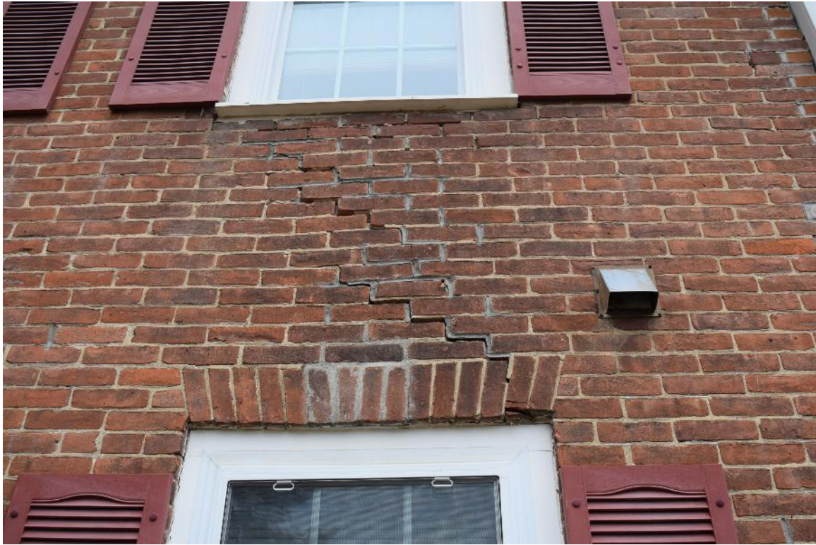
Figure 26: View shows example of widespread structural problems with the brickwork
