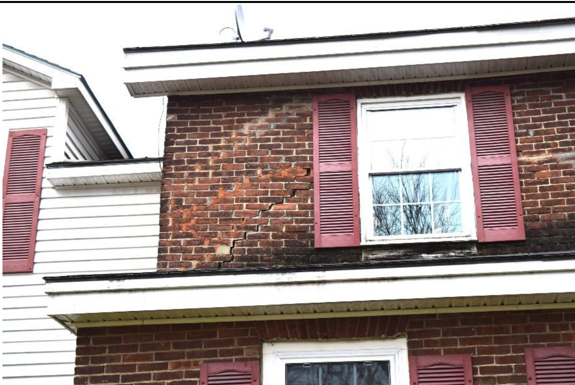
Figure 29: View shows example of widespread structural problems with the brickwork
