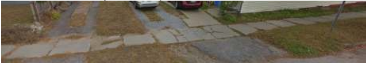
Figure 1: St Mary Street Sidewalk Condition
