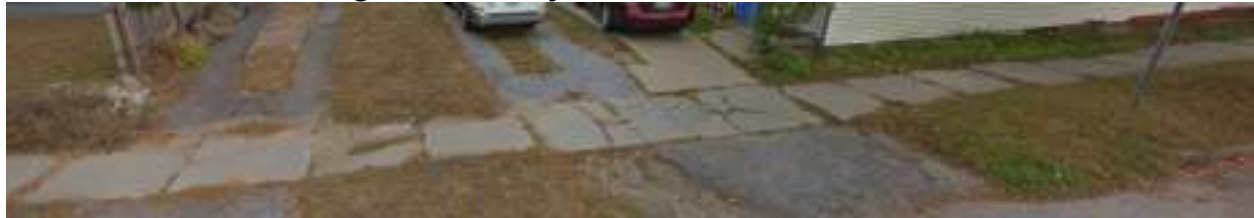
Figure 1: St Mary Street Sidewalk Condition
