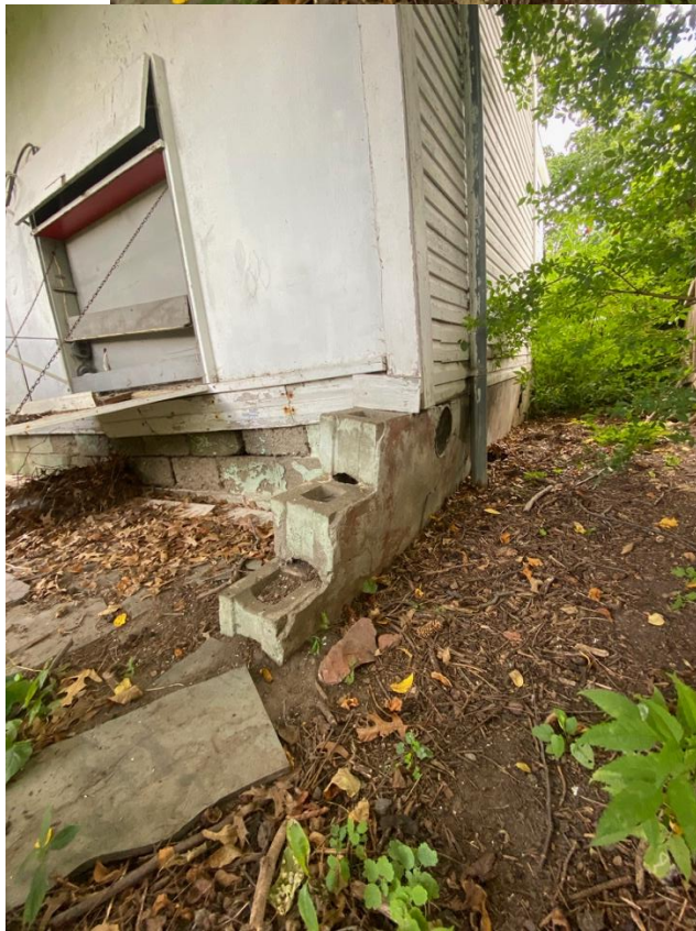
-Metal support Columns are bowed and sinking into improper footings.
