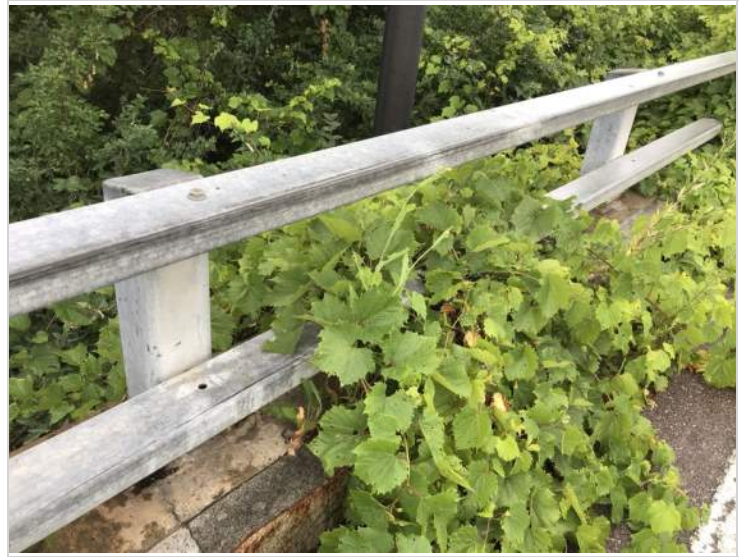
Missing lower rail bolts wingwall 2 rail posts 2 & 3
