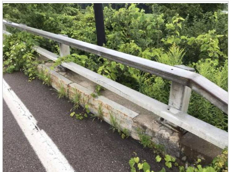
Missing rail bolts from last 3 posts on wingwall 3
