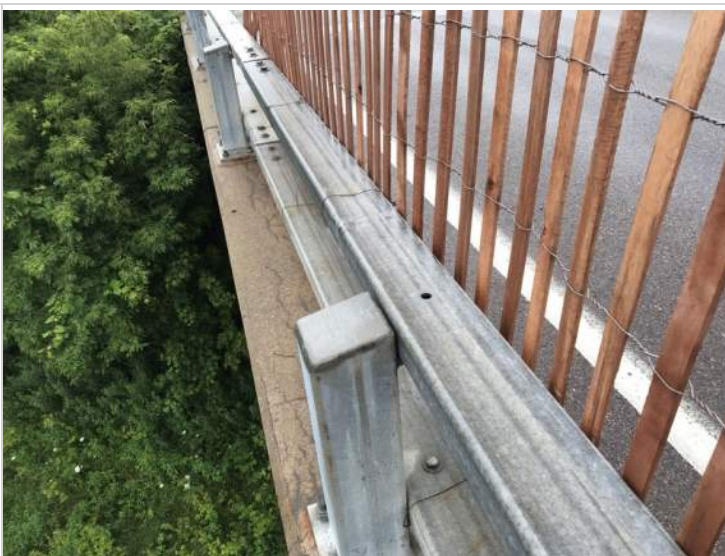
Missing top bridge rail bolts at 2nd & 3rd rail posts West of abutment 2
