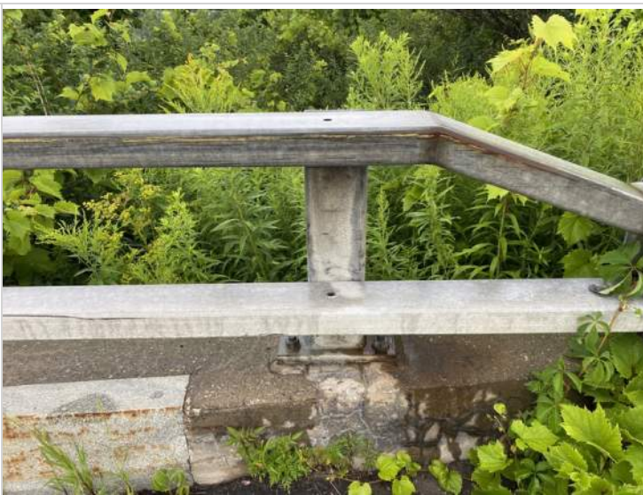
Post #24 Missing Both Connection Bolts
