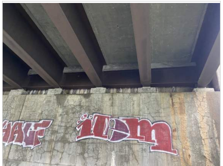
Heavy Efflorescence Leakage at Abutment #1 Backwall
