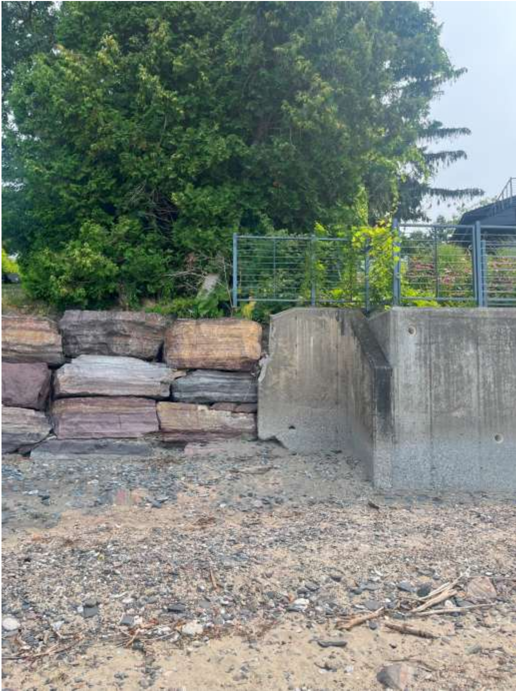
View of South–East property corner showing the last remaining section of concrete wall that was removed and replaced with boulders. This section of wall is to remain and the new wall will but up to the existing remaining section of concrete wall.
