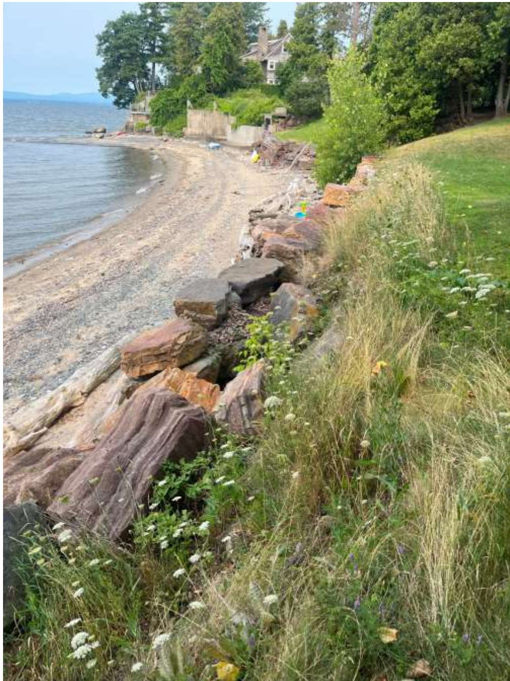
Photo showing the erosion and failing wall stones
