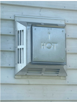
GAS FIREPLACE VENT
