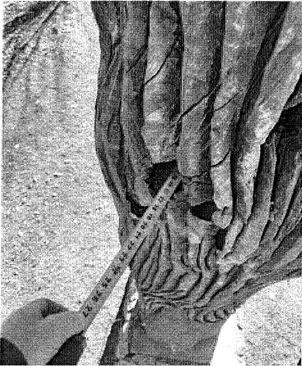
17" depth of decay along length of the upper structure
