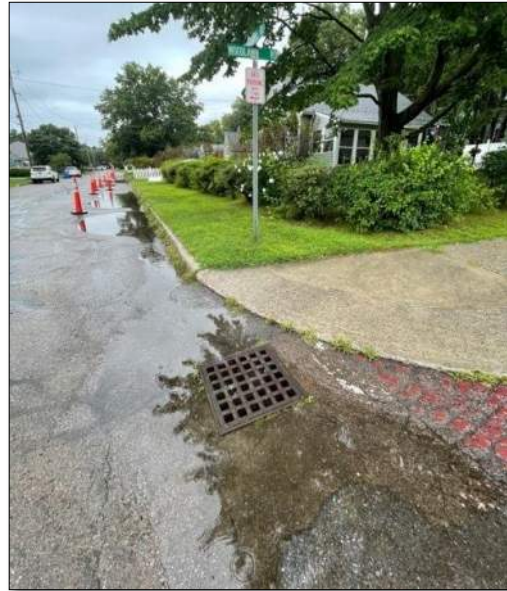
Standing Water on Stanbury Road
