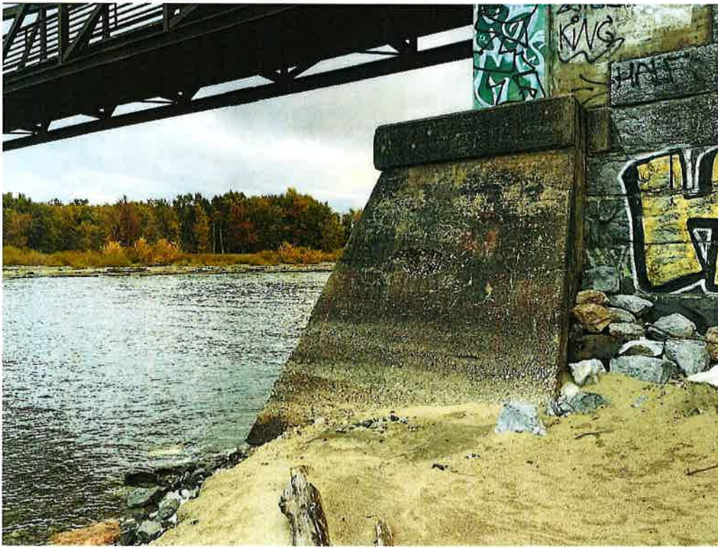
Southern Abutment – Downstream – Fill is small granular material covered in fine sand.
