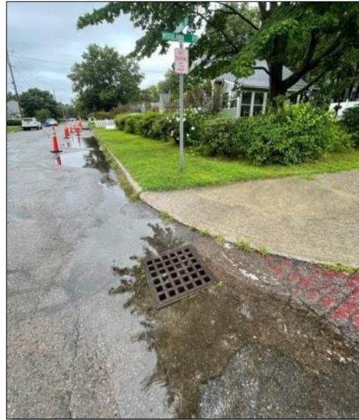
Standing Water on Stanbury Road
