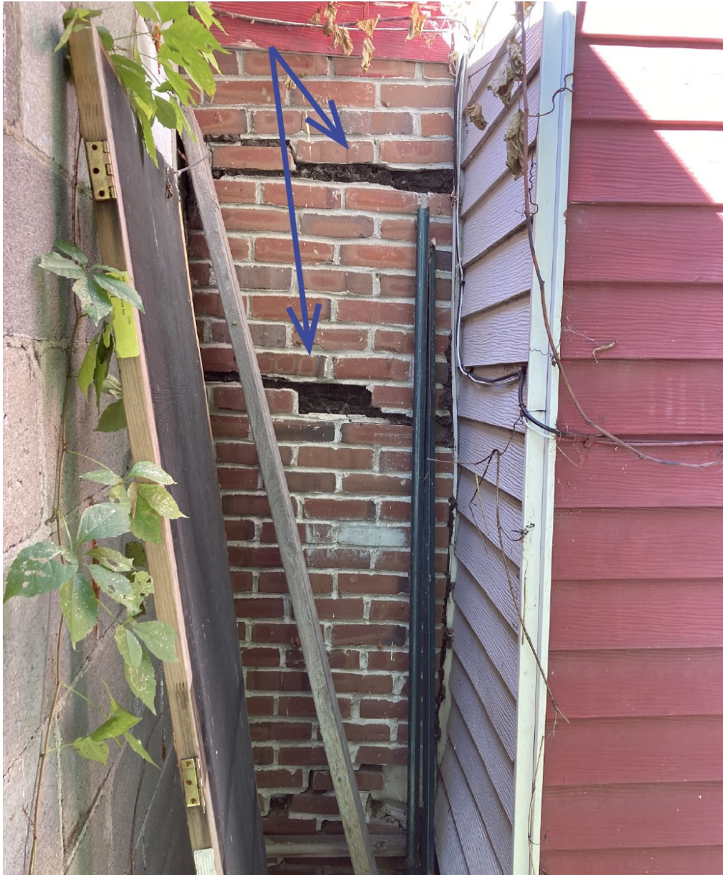
Photograph 3: Separation of the exterior wall of the structure on the Parcel. The slope is to the right of this view; note the relative horizontality of bricks at the top of the wall (intact), while bricks lower down on the wall are cracked and progressively slanted into the slope as the soils below the foundation are compromised.
