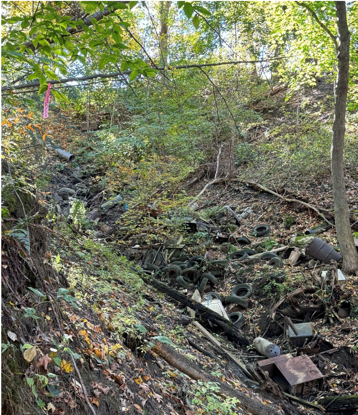
Photograph 2: View facing southeast and upslope toward the structure on the Parcel of artificial fill material exposed by gully erosion caused by stormwater diversion onto the slope. Note the location of the stormwater discharge pipe in the upper left portion of the photograph.
