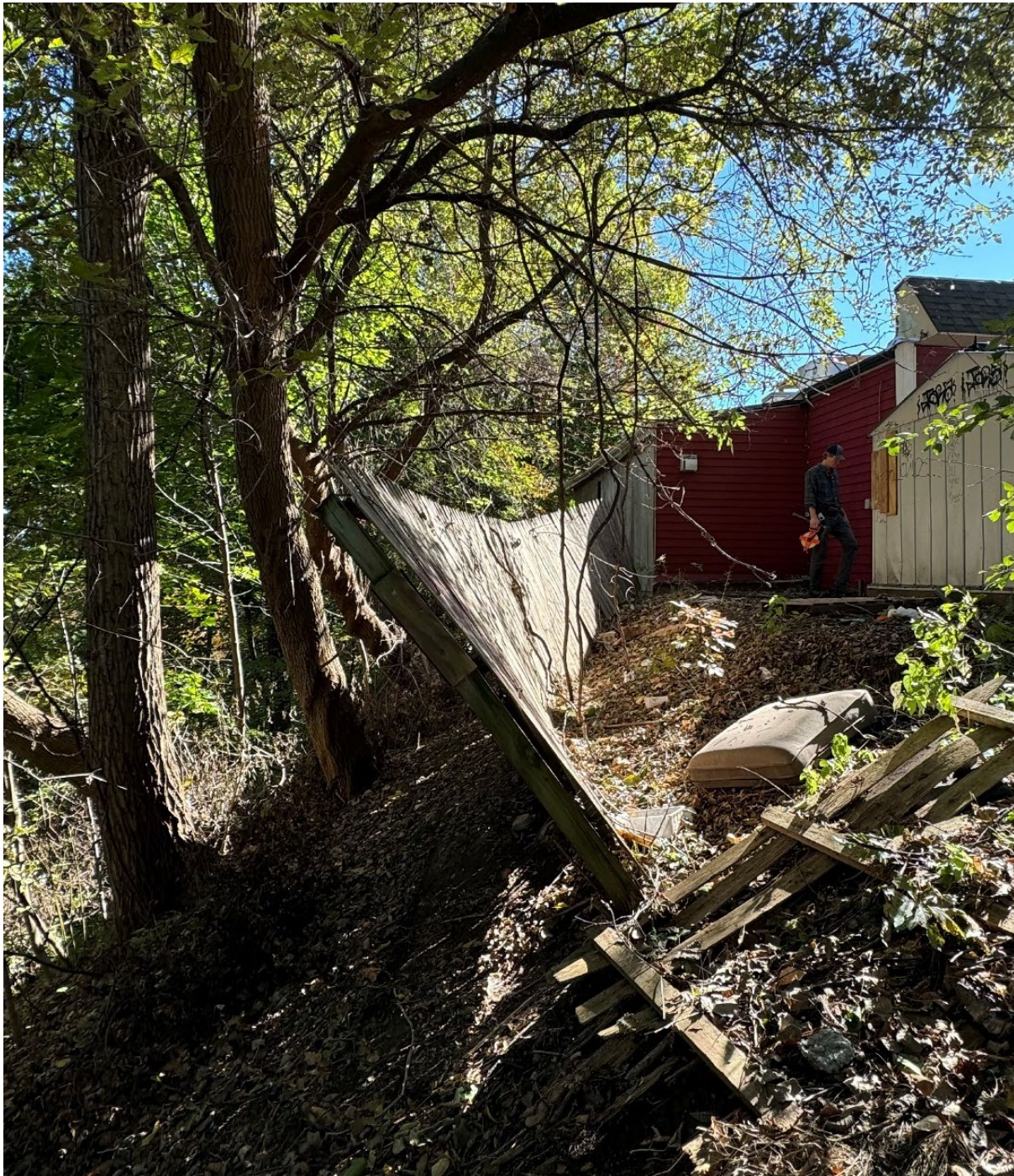
Photograph 4: View facing to the east showing the compromised wooden fence behind the structure on the Parcel. The tree trunks to the left of fence also show deformation and curvature.
