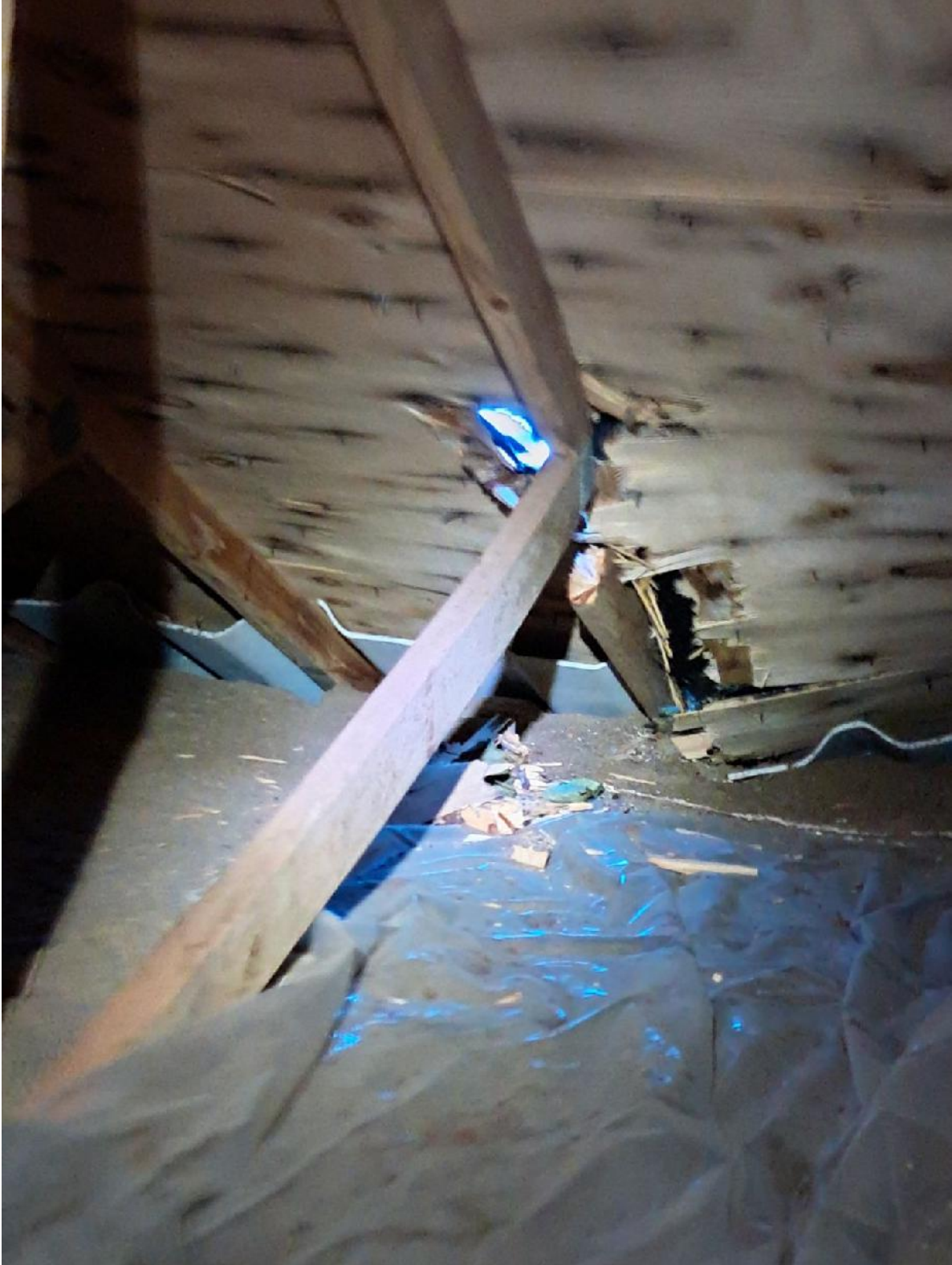
Photo 3: Structural roof damage caused by July 22, 2024 GMHFH tree felling incident, interior view, Rockland Condominiums, unit A.
