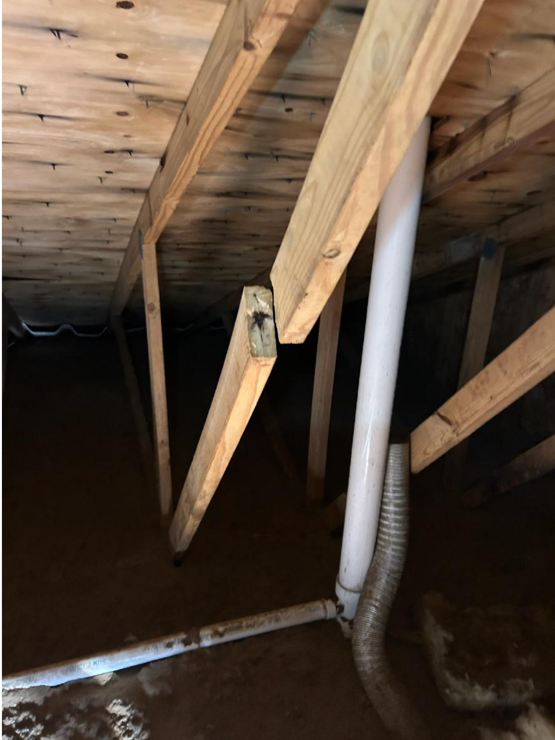
Photo 4: Structural roof damage caused by July 22, 2024 GMHFH tree felling incident, interior view Rockland Condominiums, unit B.
