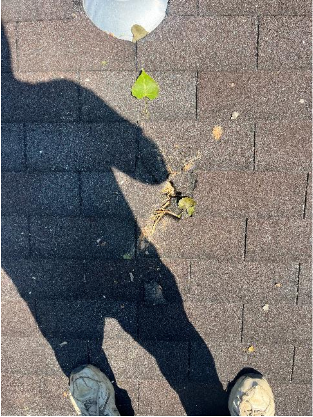
Photo 6: Damage caused by GMHFH tree felling incident, exterior view. July 22, 2024.
