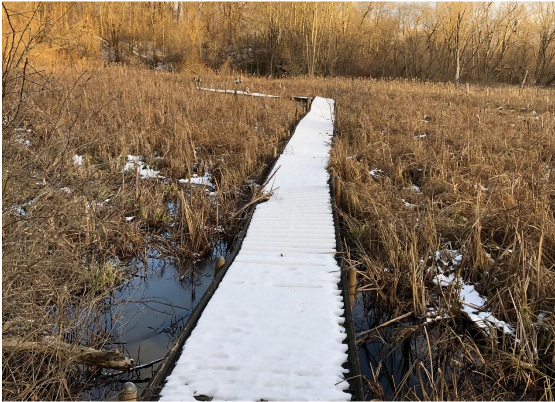
View of Wetlands Walk North Boardwalk looking east showing uneven/warped decking sections from damage to steel anchor supports. Photo taken December 13, 2023.
