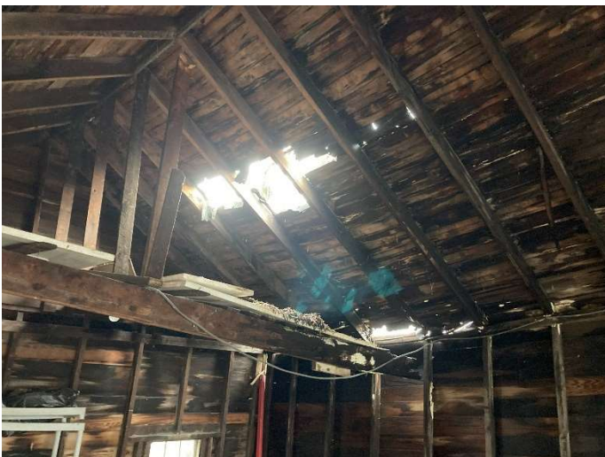
PHOTO 7: Failed section of roof at west side
