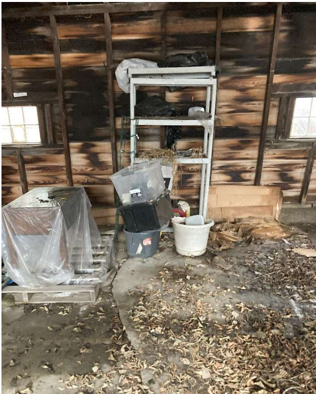
PHOTO 5: Cracking and displacement/settlement of garage slab
