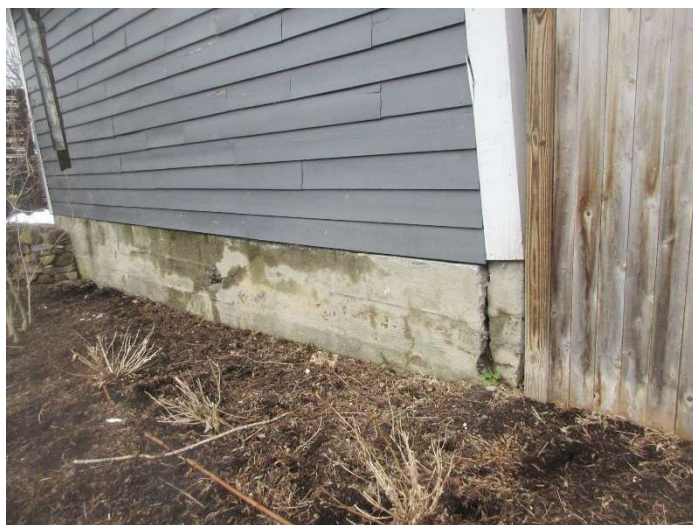
PHOTO 4: Displacement in west foundation wall
