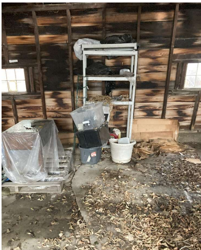
PHOTO 5: Cracking and displacement/settlement of garage slab
