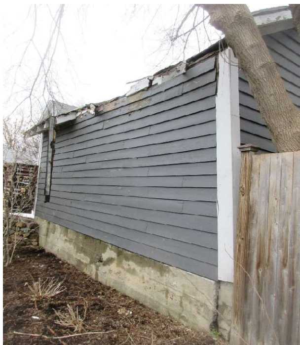
PHOTO 3: Cracks & displacement in west foundation wall
