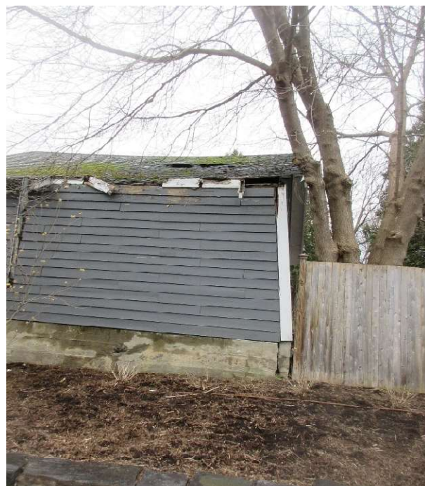
PHOTO 8: Warping of building due to tree growth
