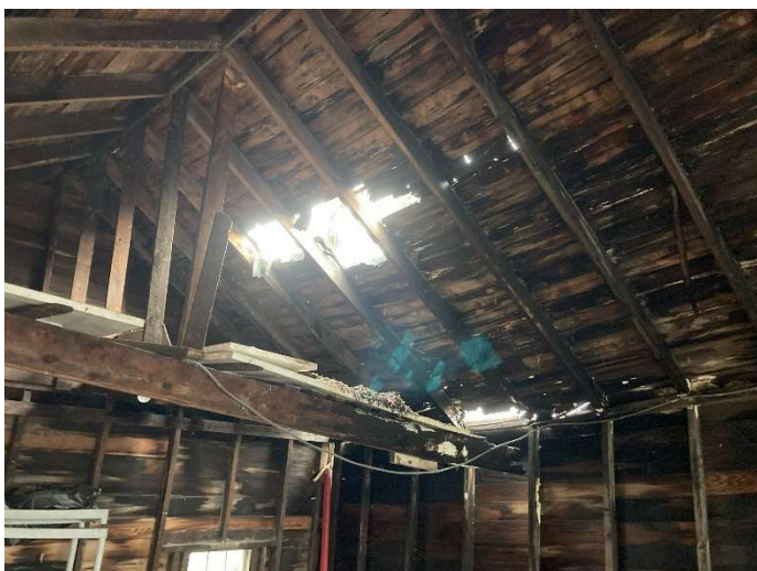
PHOTO 7: Failed section of roof at west side
