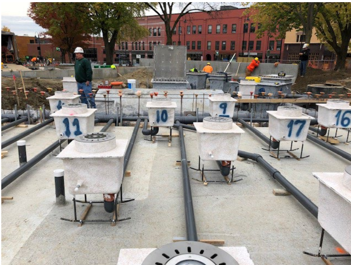
Nozzle Plumbing, Tanks, and Structures
