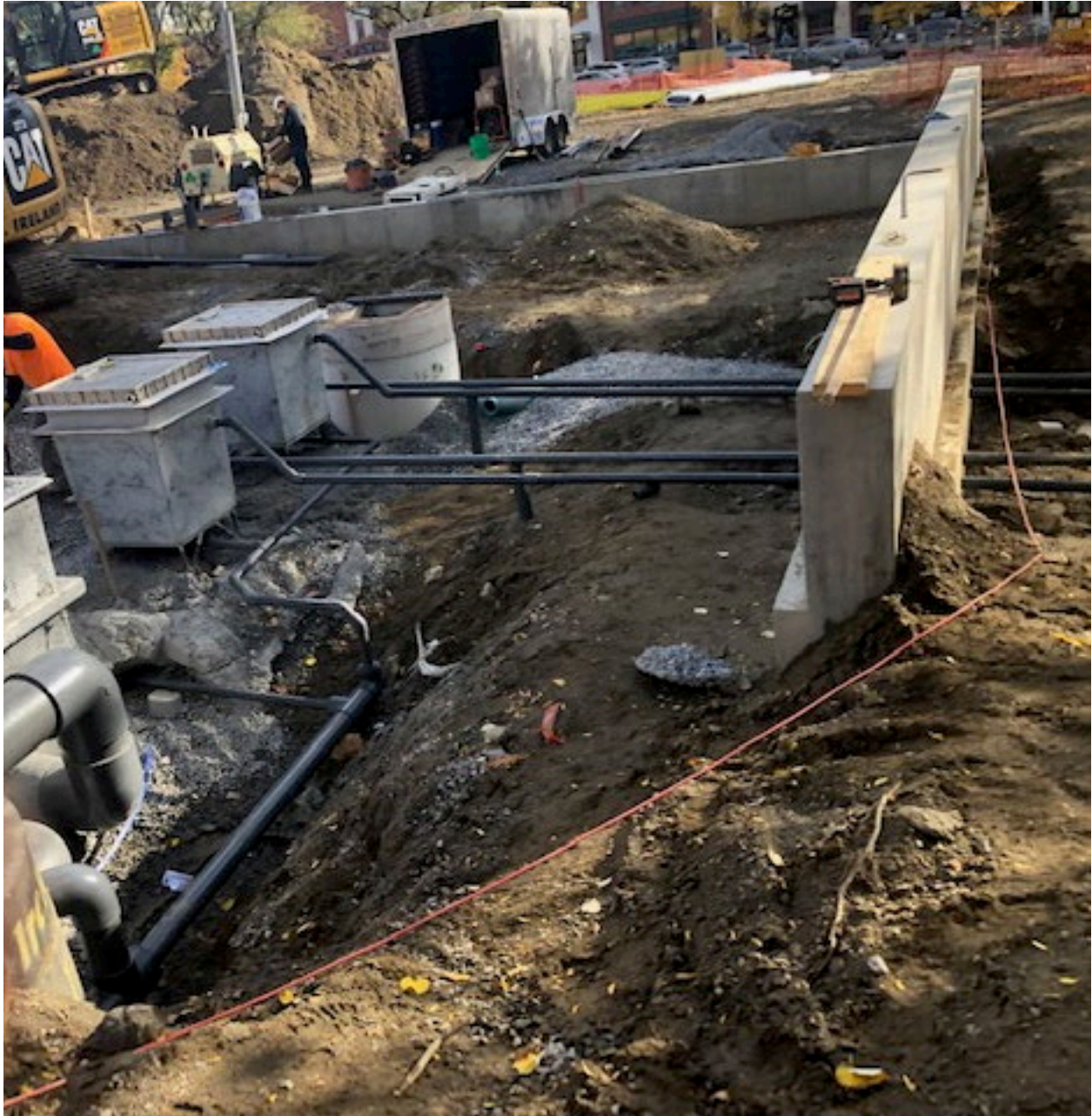
Chemical Tanks Plumbing (below location of Kiosk)
